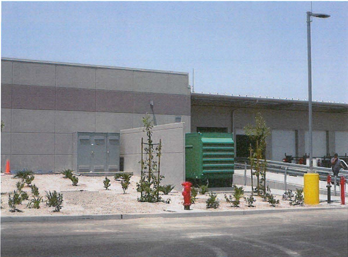
Picture of emergency generator screening
