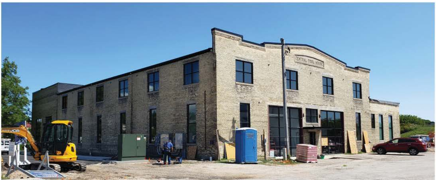
▲ A view of the ongoing historic rehabilitation efforts of 1320 Niagara Avenue. This building will feature 2-3 new mixed-use tenants.
