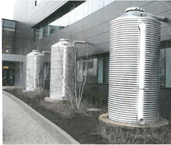
Green Infrastructure-Rainwater Harvesting
