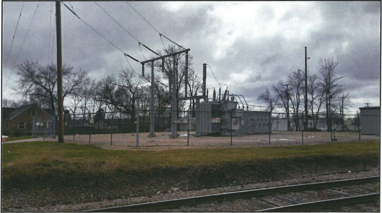
Sauk Trail Substation Looking Southeast
