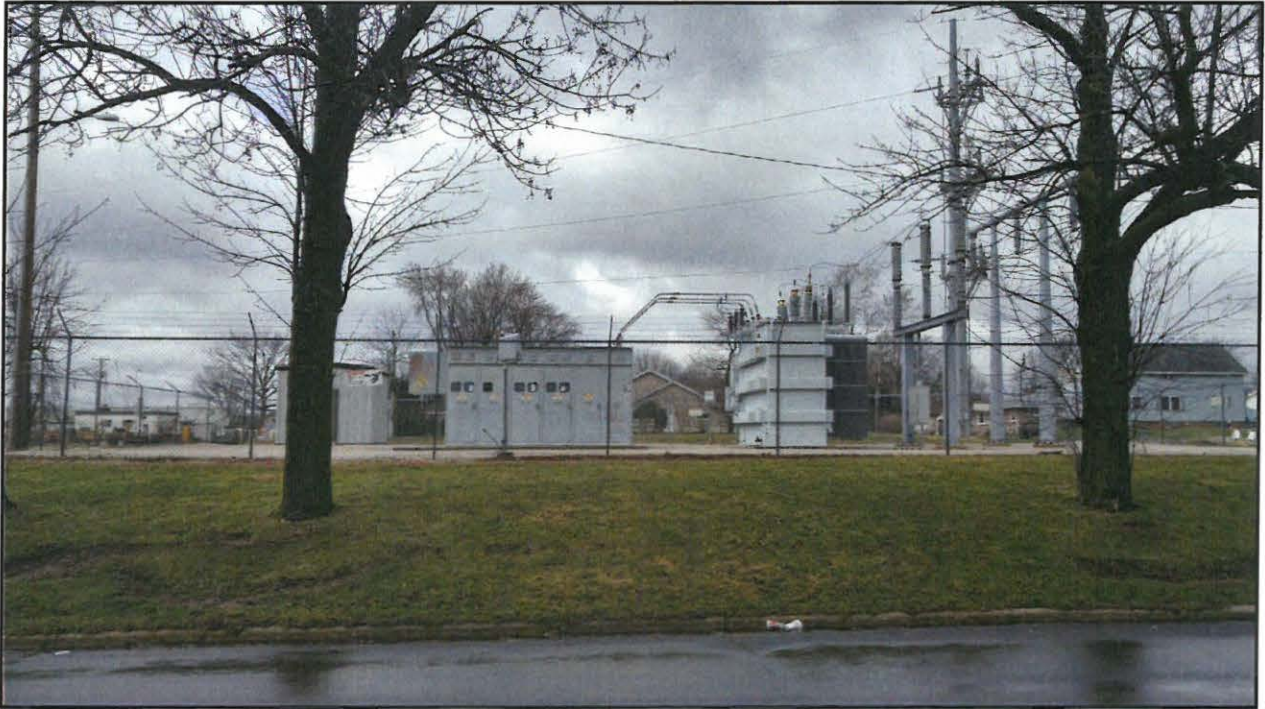
Sauk Trail Substation Looking West
