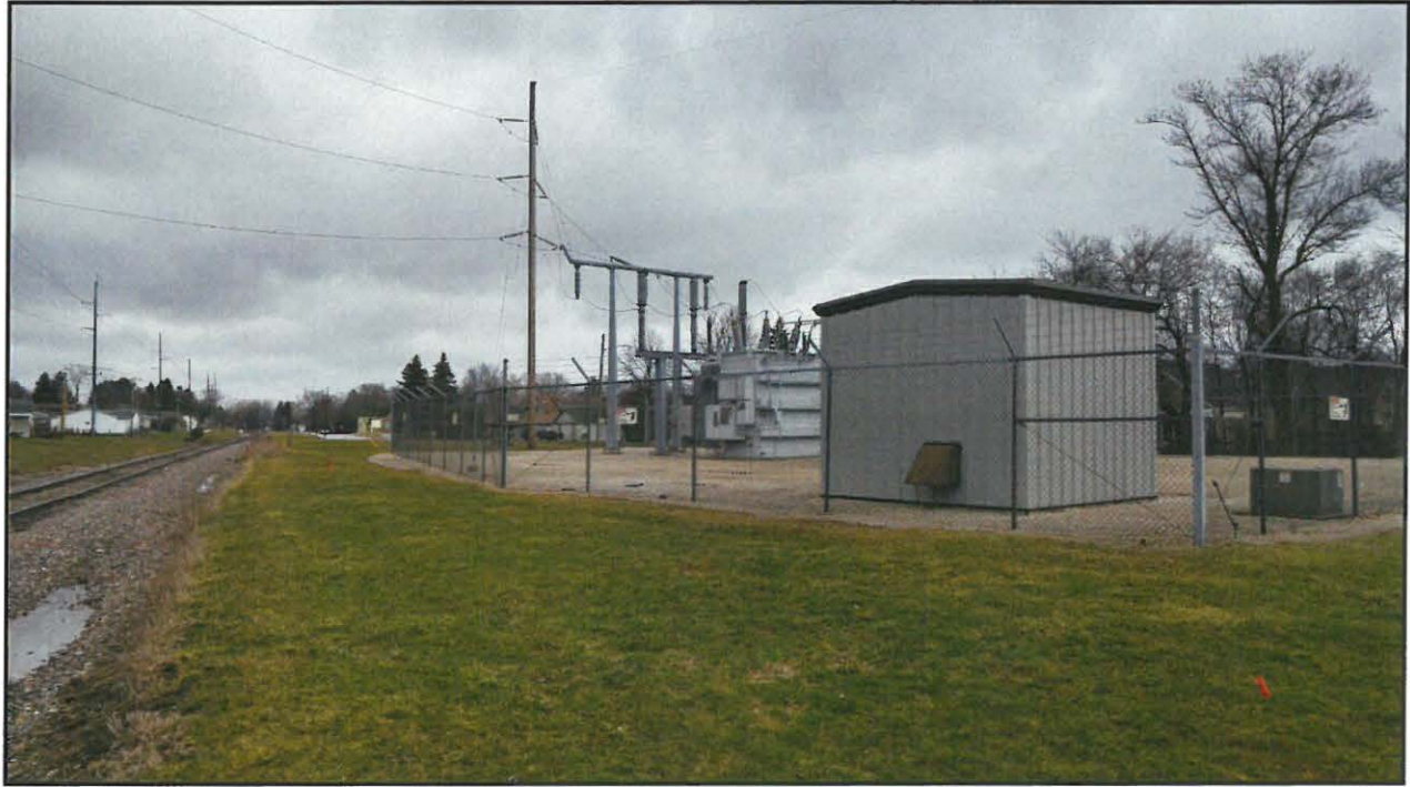
Sauk Trail Substation Looking North
