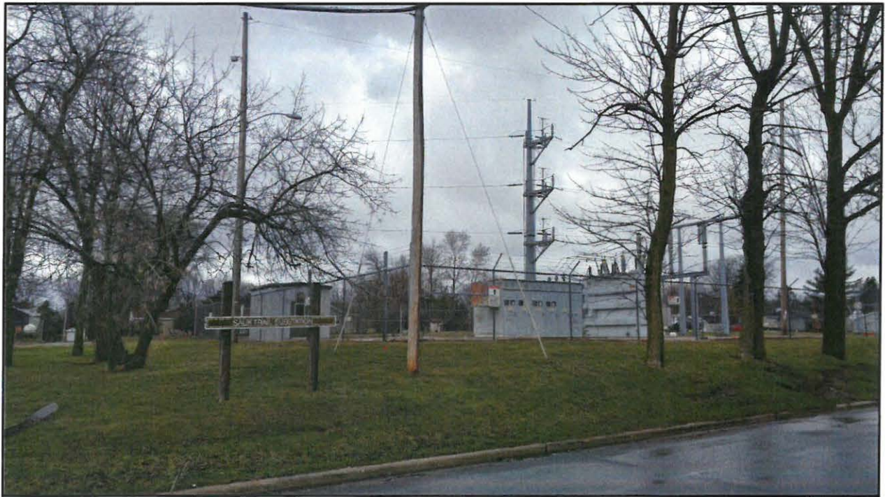
Sauk Trail Substation Looking Northwest
