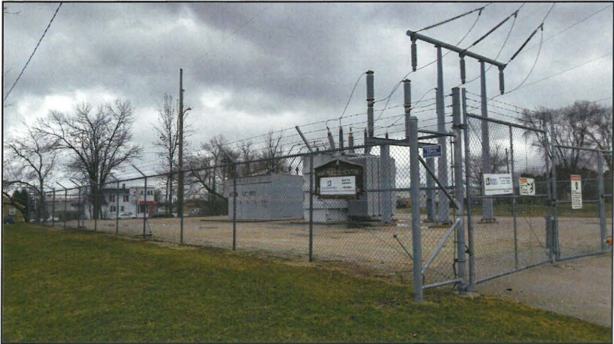
Sauk Trail Substation Looking Southwest
