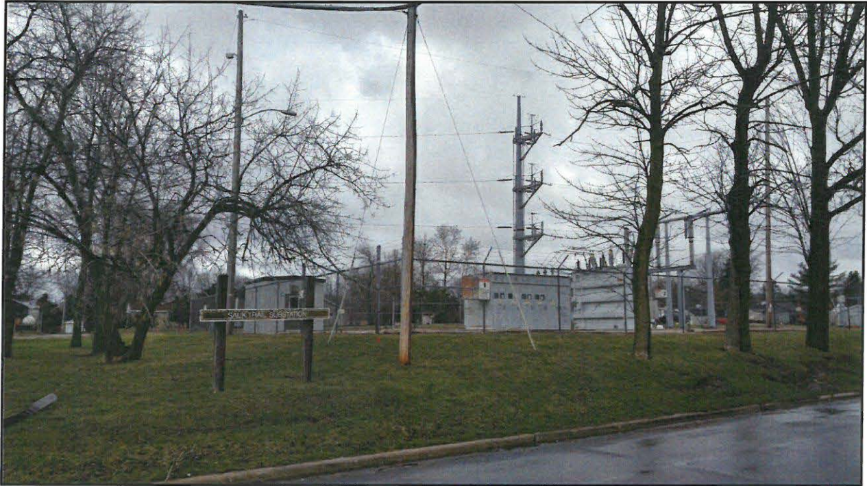
Sauk Trail Substation Looking Northwest
