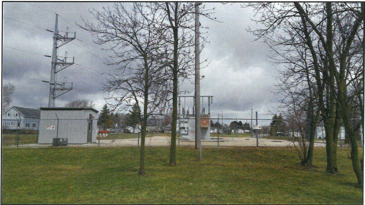
Sauk Trail Substation Looking North
