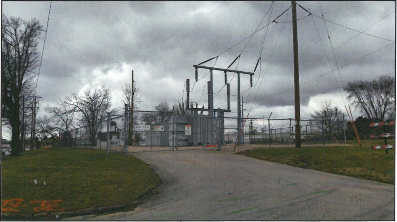
Sauk Trail Substation Looking South/Southwest
