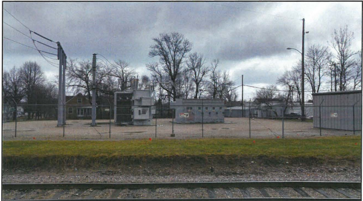
Sauk Trail Substation Looking East
