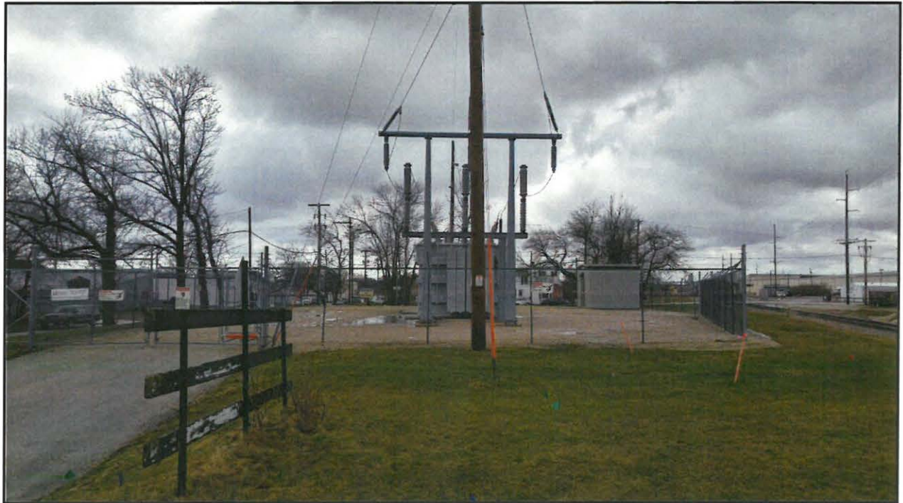
Sauk Trail Substation Looking South
