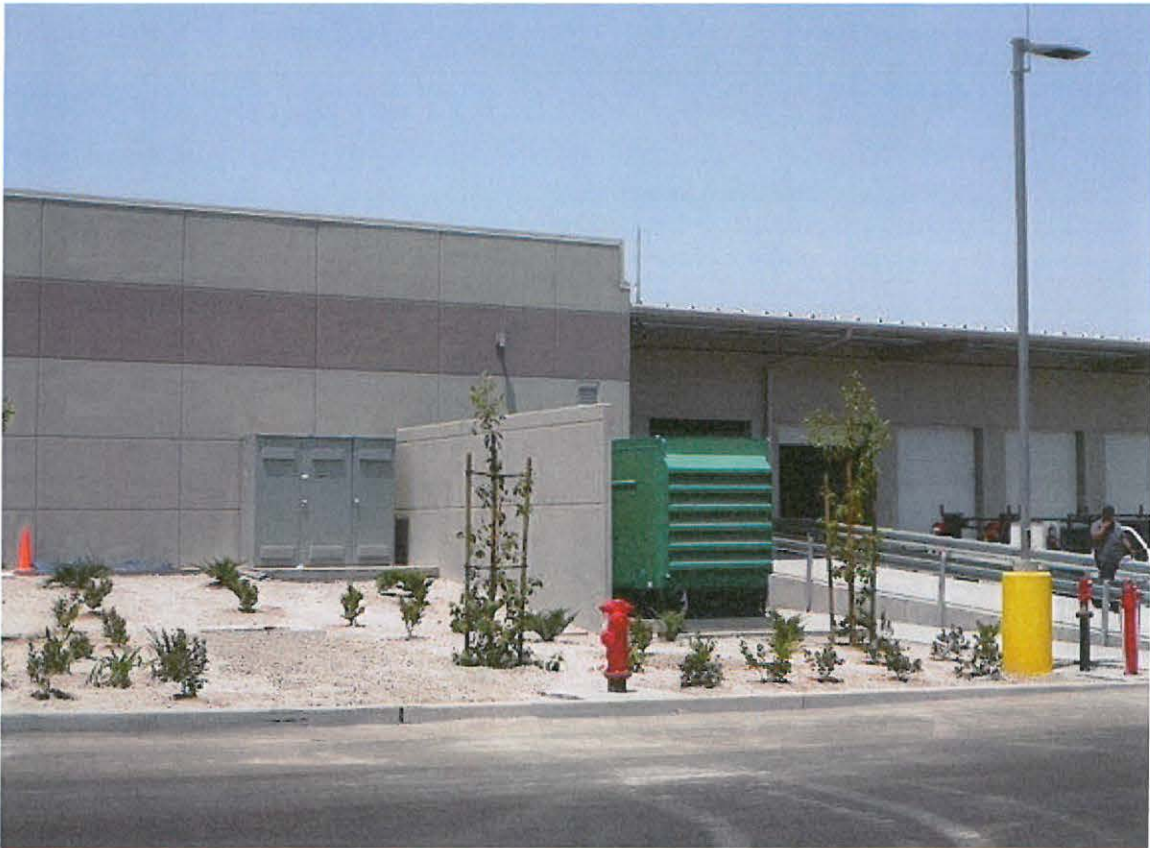
Picture of emergency generator screening
