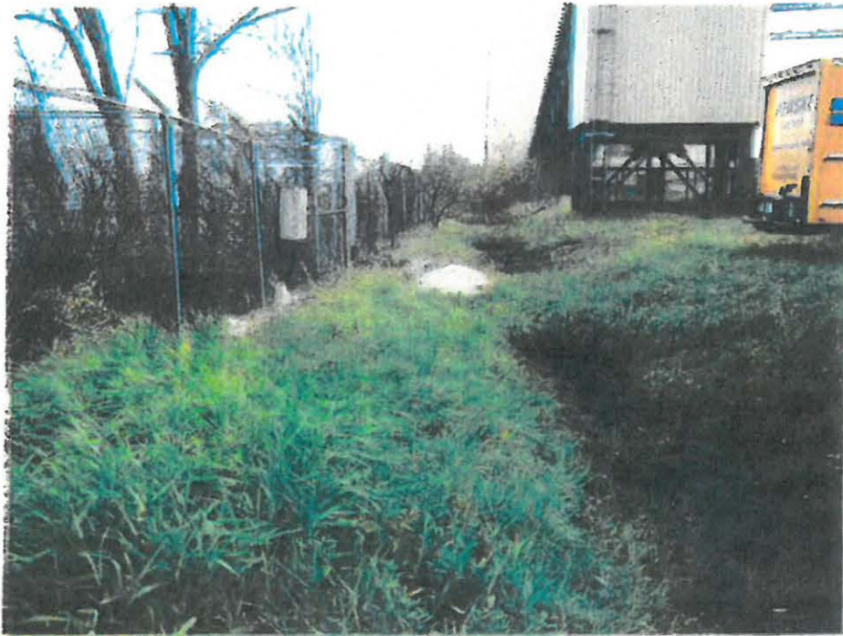
Photo 1: Looking south along the existing earthen drainage swale. The portion that is proposed to be lined with concrete is in the rear-center of the photo, along the Crusher House, which is in the background-right of the photo.
