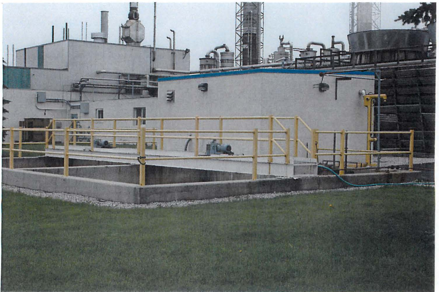
Looking Southwest—Existing Pump House
