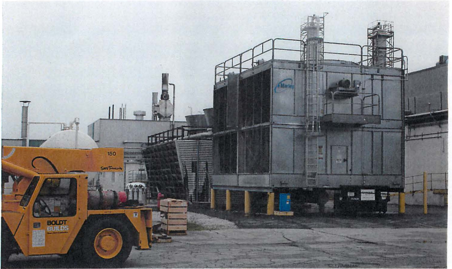
Looking Southwest—Existing Cooling Towers
