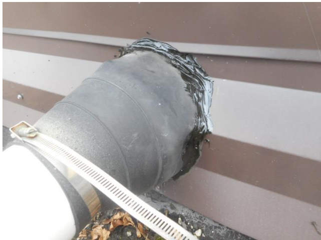
Transit Garage – Roof #1 – Open pipe penetration through metal counterflashing was sealed with polyurethane sealant.
