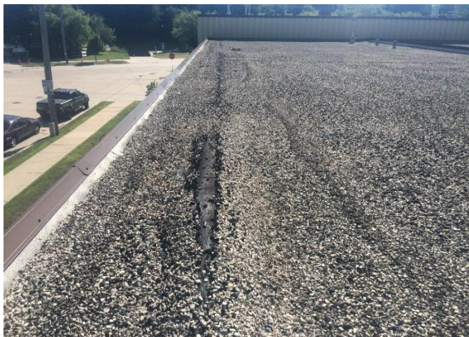
Transit Garage - Roof #4 – Overview of large blistering areas visible along ply laps. Result of improper installation and adhesion. Fractured blisters lead to a water entry point.
