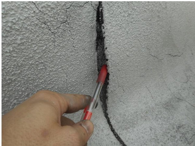
Transit Garage – Roof #2 – Open lap on flashing. Water entry point.
