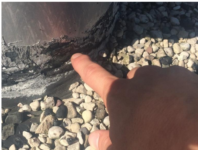
Transit Garage - Roof #5 – Cracked sealant around pipe penetration was filled and repaired with polyurethane sealant.
