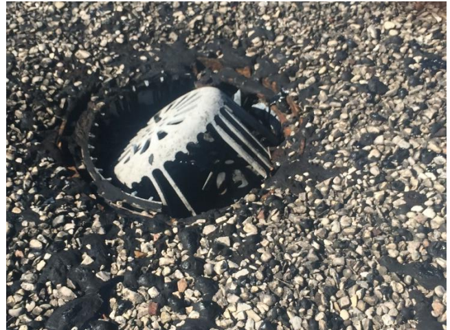
Transit Garage - Roof #5 – Crushed drain cover in need of replacement.
