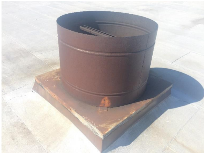
Transit Garage - Roof #3 – Numerous thoroughly rusted ventilation hoods. Aluminum rust prohibitive coating to prevent further metal deterioration recommended.
