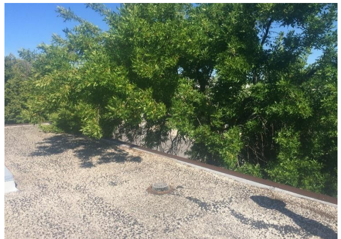
Transit Garage - Roof #4 – Large tree branches hanging over roof. This results in debris clogging the drain, and the risk of broken branches penetrating the roof system.
