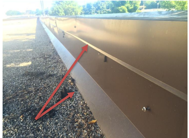
Transit Garage – Roof #1 – Fasteners only used sporadically during coping installation resulting in inadequate attachment.
