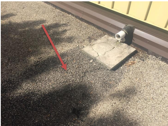
Transit Garage - Roof #1 – Lack of drain pipe extension to drain resulting in severe aggregate washout & membrane deterioration.
