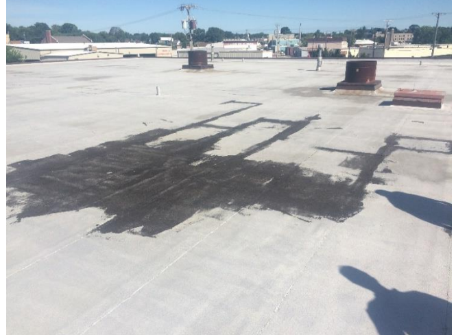
Transit Garage - Roof #2 – Overview of large area repair attempt with ineffective materials. Appears to be asphalt flood coat over MB membrane.
