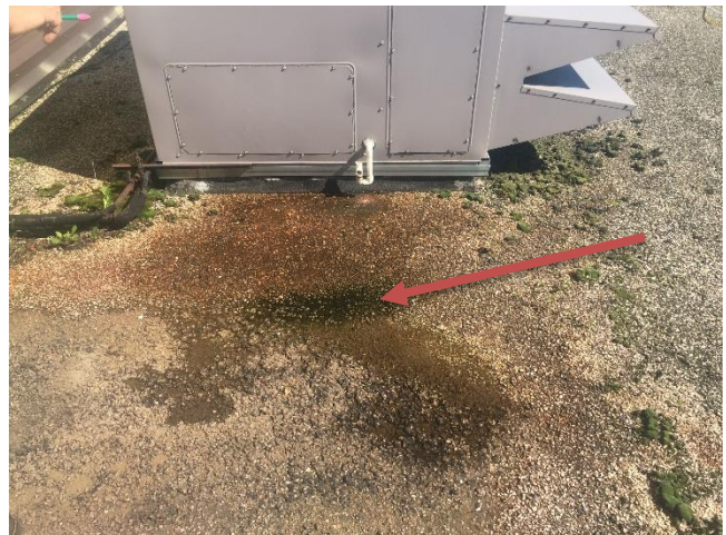
Transit Garage - Roof #1 – Lack of pipe extension lead to ponding water around A/C unit. This results in aggregate washout and vegetative/mold growth.
