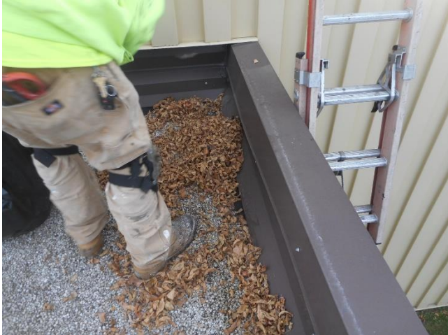
Transit Garage – Roof #1 – Significant organic debris can lead to clogged drains and ponding water on roofs.
