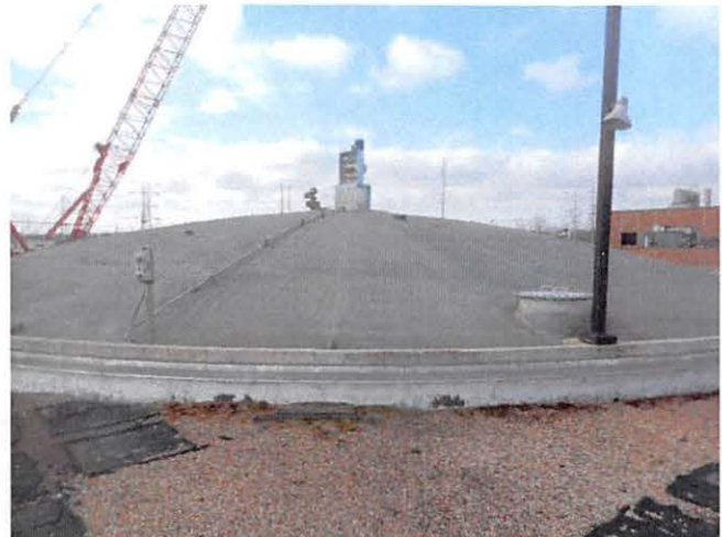
New Water Treatment Roof – 3 of 4 large digesters covered with spray foam insulation. 4 th digester is bare metal. Recommend coating all 4 to prevent deterioration seen on Revised digesters.
