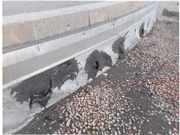
New Water Treatment Roof – Large holes in flashing around entire roof perimeter. Roof in failure mode and scheduled for replacement in 2018.
