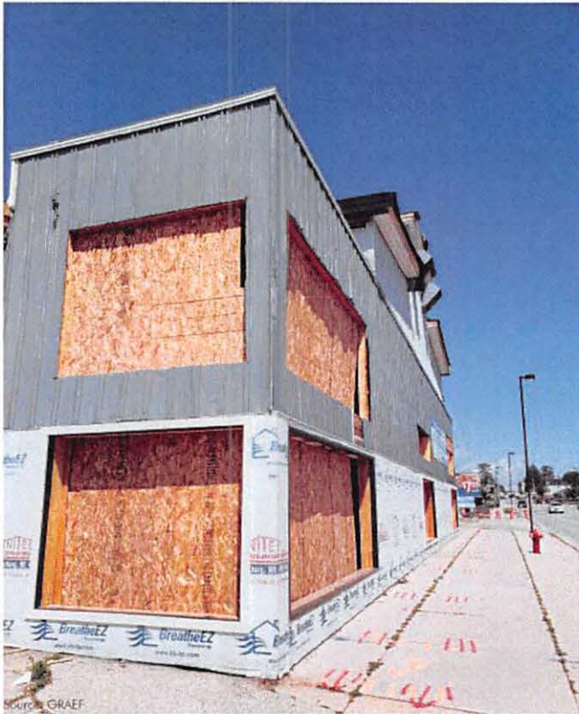
▲ A view of the rehabilitation of 822 N. 14th Street into a commercial space.
