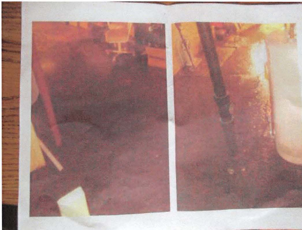
2-Photos provided by insured of sewage in basem
