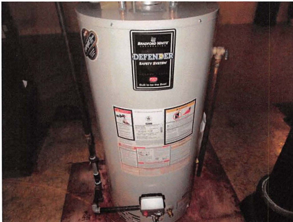
16-New water heater
