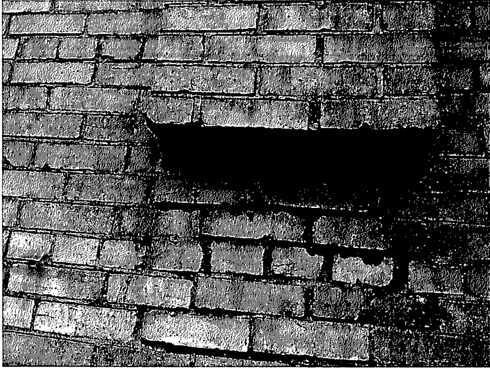
Figure 27: Deteriorated mortar joints.
