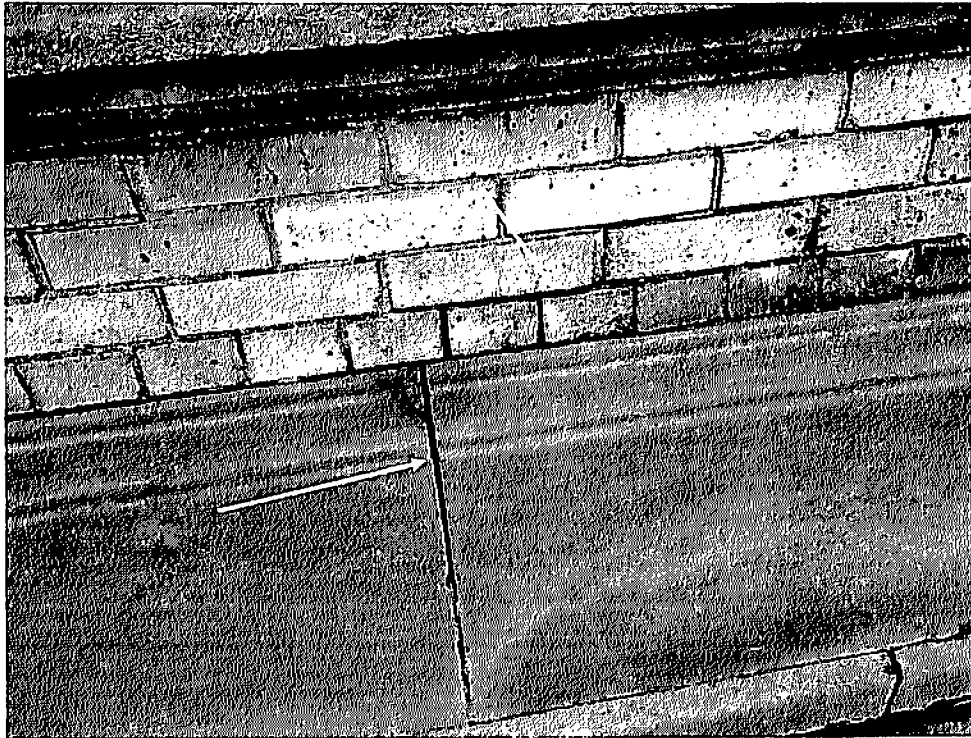
Figure 28: Deteriorated and open mortar joints.
