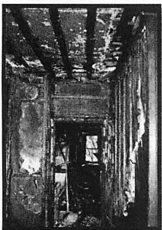
BURNED INTERIOR ROOM IN A LOCAL RESIDENCE.
