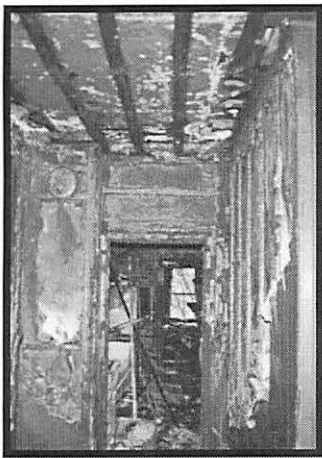
BURNED INTERIOR ROOM IN A LOCAL RESIDENCE.
