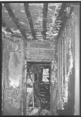
BURNED INTERIOR ROOM IN A LOCAL RESIDENCE.
