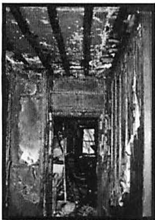
BURNED INTERIOR ROOM IN A LOCAL RESIDENCE.
