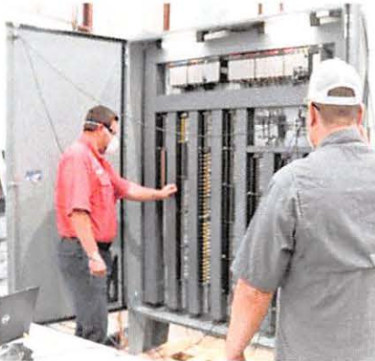
Control Panel FAT
