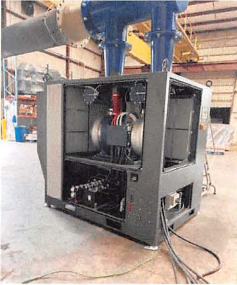
DT Series Prep for ASME Performance Testing
