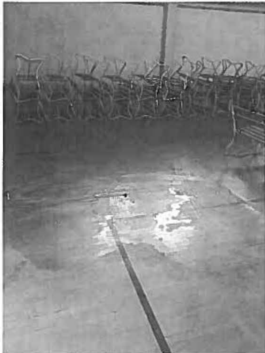
Roof leaking damage on gym floor
