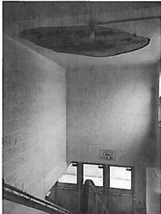
Continued ceiling damage
