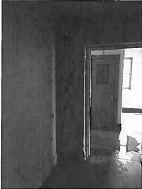
New damage from Winter 2016-2017
