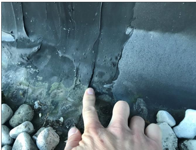
Roof #1 – Crack in sealant in tented flashing.
