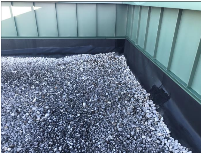
Roof #1 – Significant tenting visible around perimeter of Roof #1.
