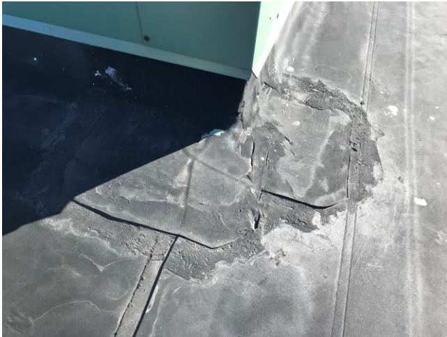
Roof #6 – Delaminated areas visible in corner details.
