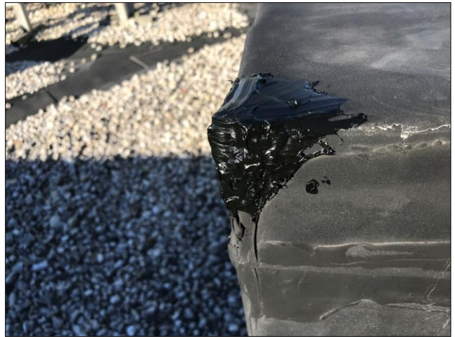
Roof #1 – Area was repaired with a small patch of uncured EPDM flashing material and covered with polyurethane sealant.
