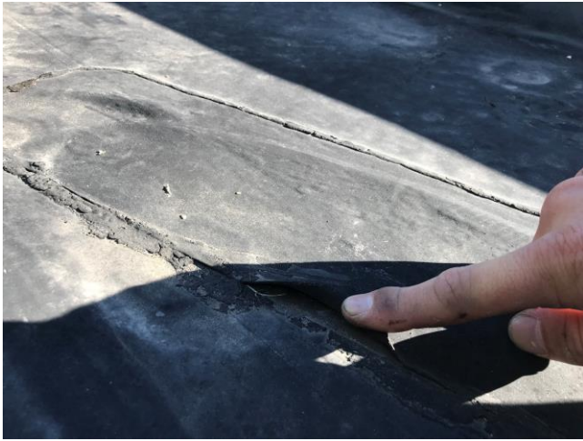
Roof #4 – Delaminated perimeter of previous patch.
