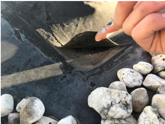
Roof #1 – Delaminated area of patch.
