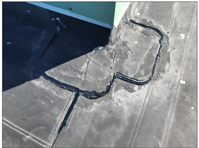
Roof #4 – Sealant was applied to perimeter areas and flashing material was set back into place.
