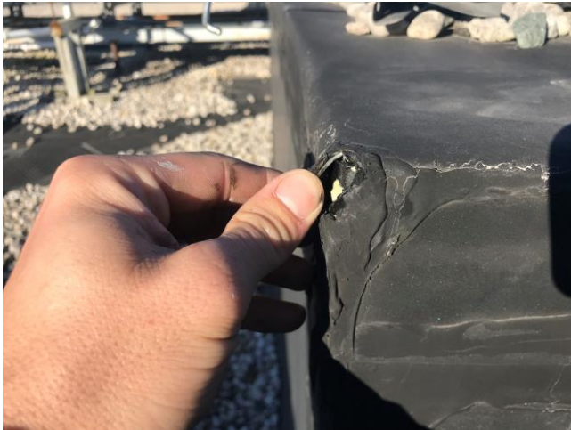
Roof #1 – Hole found in corner of raised roof area.
