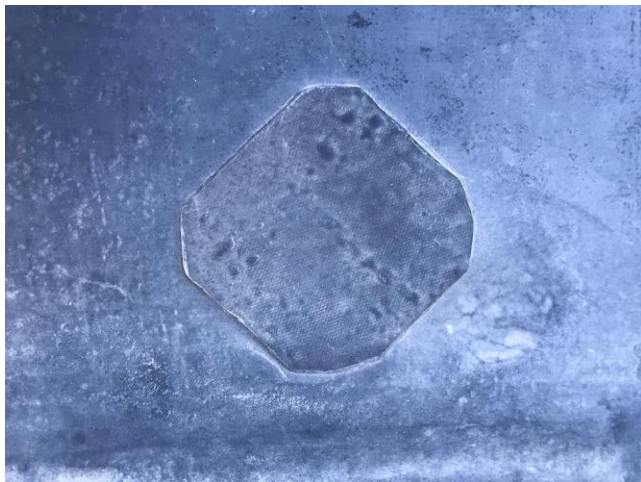
Roof #6 – Previous patch, no sealant.
