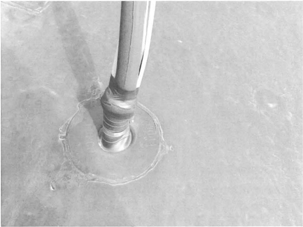
Figure 16: Improperly sealed A/C line penetration.
