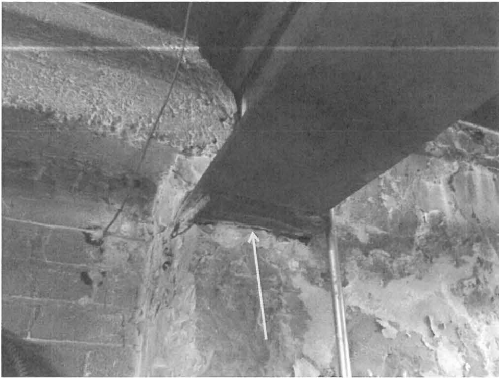
Figure 37: Corrosion of steel beam.
