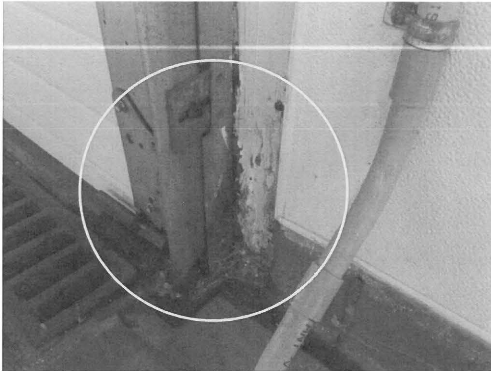
Figure 49: Deterioration of wood trim at garage door.
