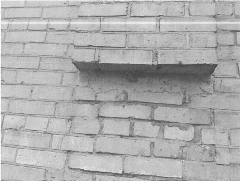
Figure 27: Deteriorated mortar joints.
