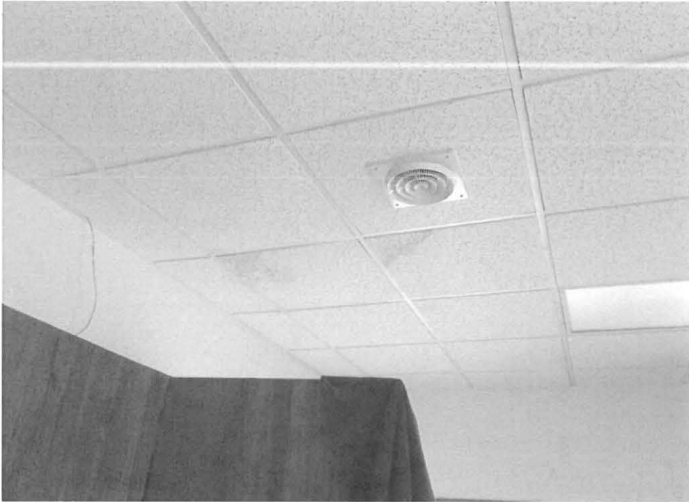
Figure 47: Stained ceiling tiles.
