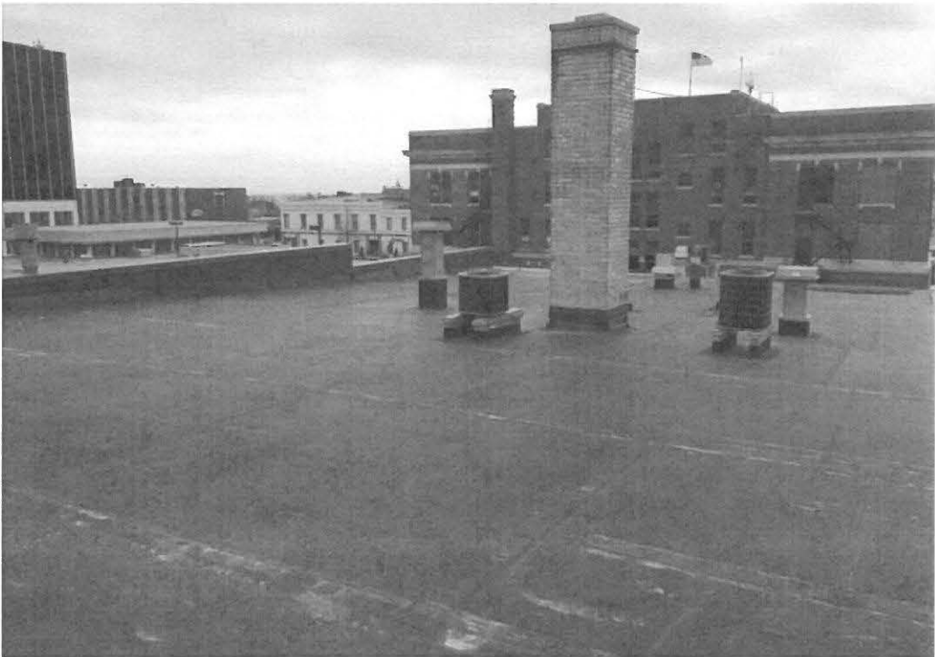
Figure 8: Full adhered EPDM roof system.
