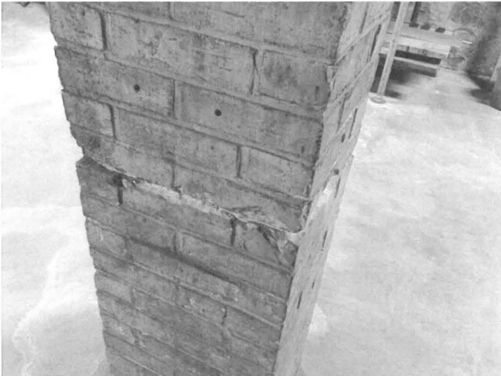
Figure 42: Brick deterioration; Deteriorated mortar joints.
