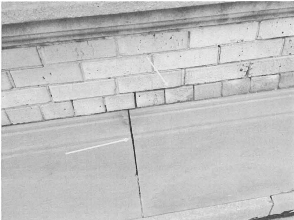
Figure 28: Deteriorated and open mortar joints.
