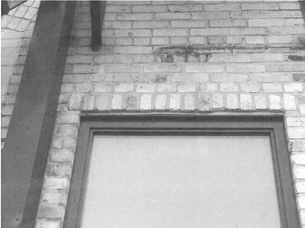
Figure 30: Corroded steel lintel.
