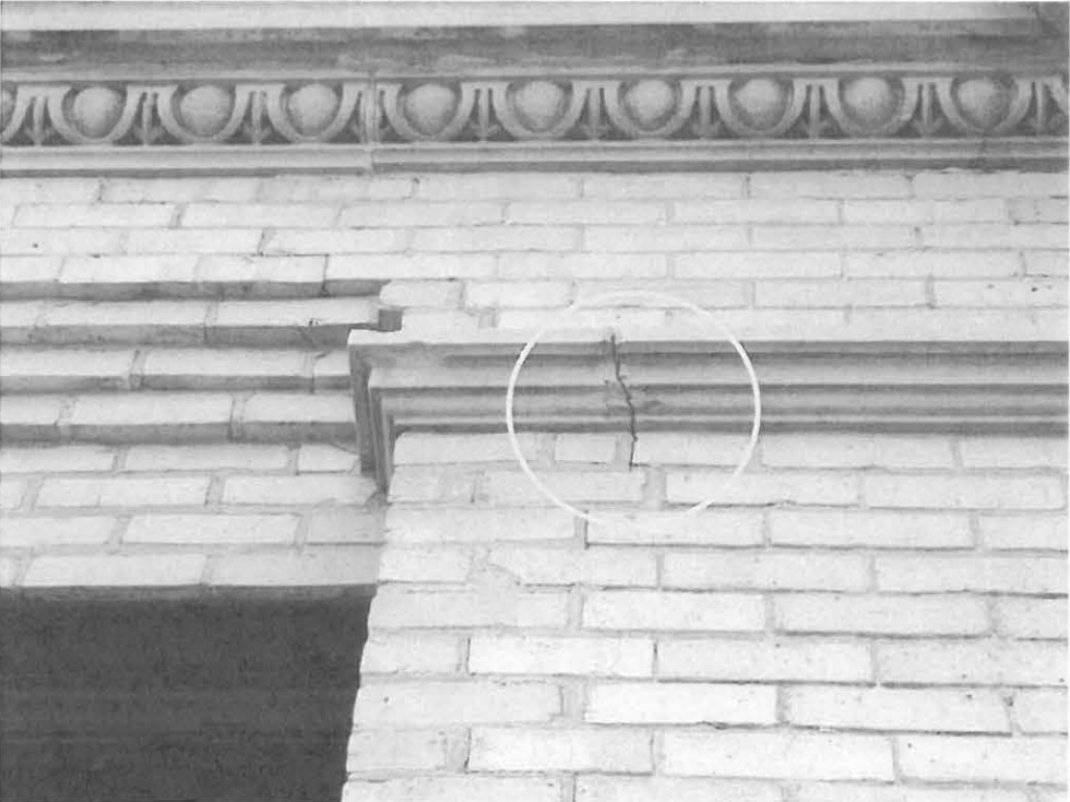
Figure 32: Cracked stone unit.
