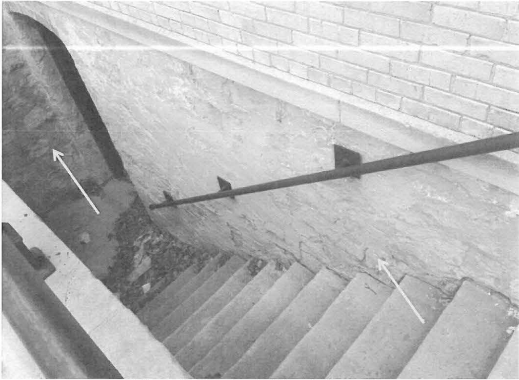
Figure 7: Deteriorated foundation walls.
