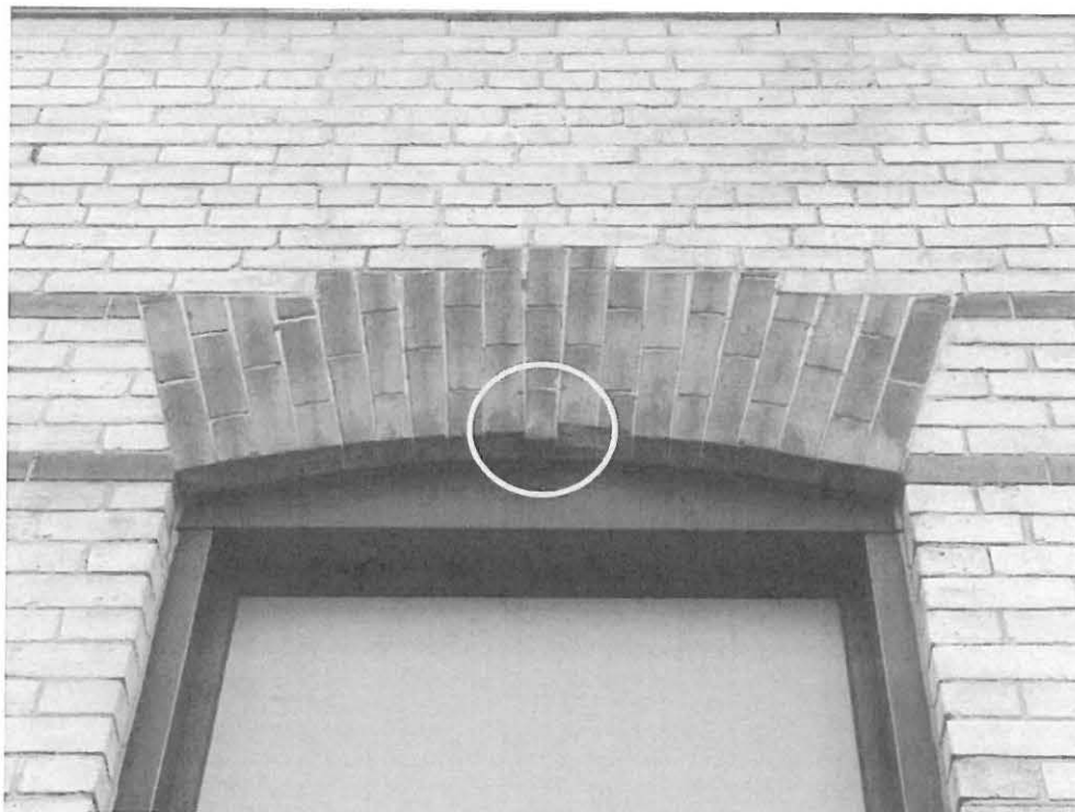
Figure 26: Loose brick unit.
