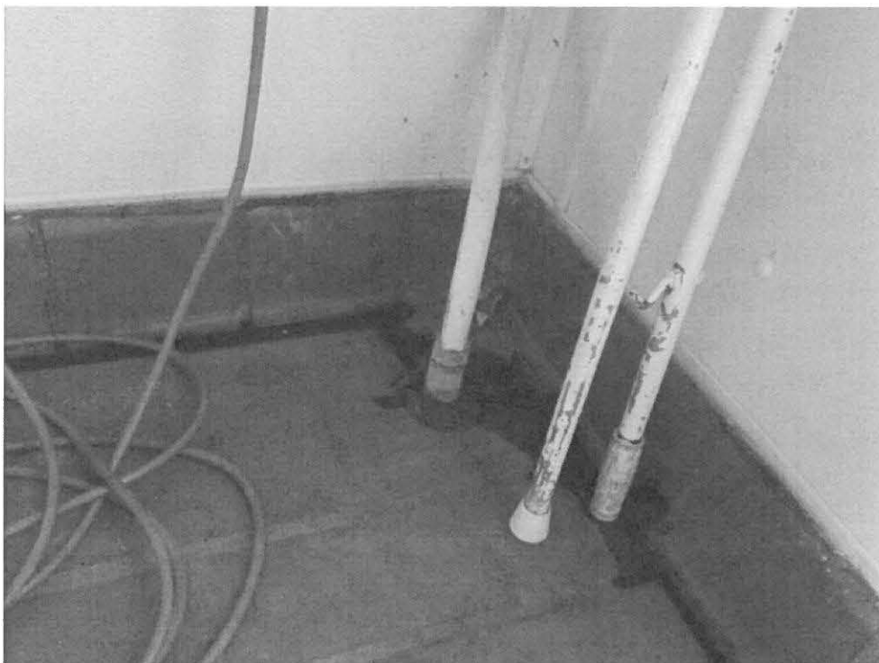
Figure 50: Unsealed penetrations allowing leaking into basement.
