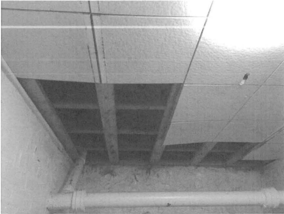
Figure 43: Missing ceiling tiles.
