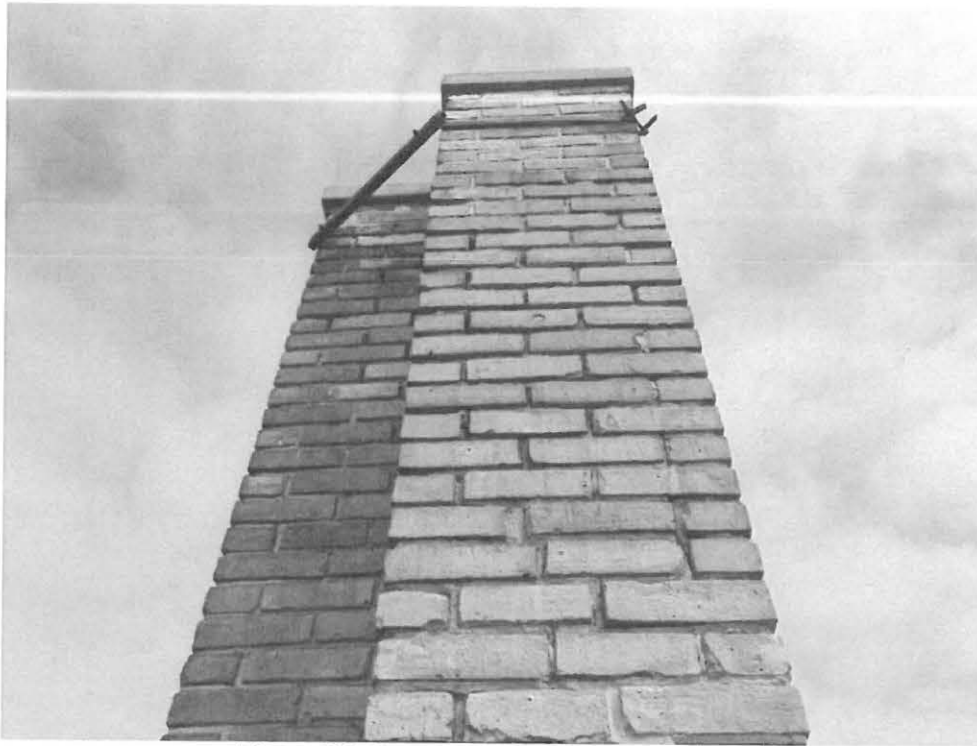
Figure 25: Deteriorated brick at chimney.
