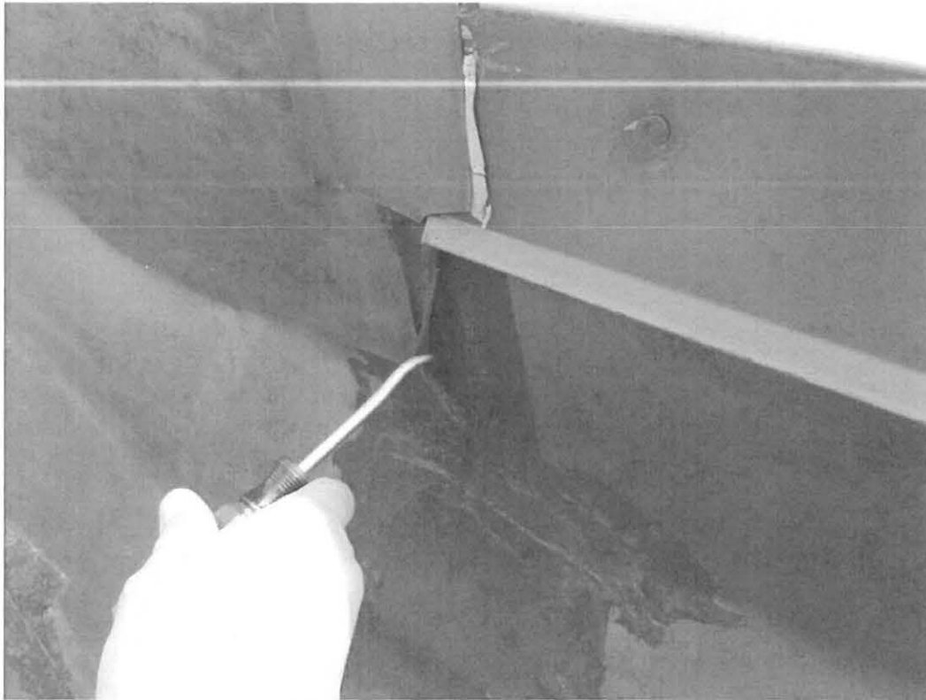
Figure 17: Open flashing seam.
