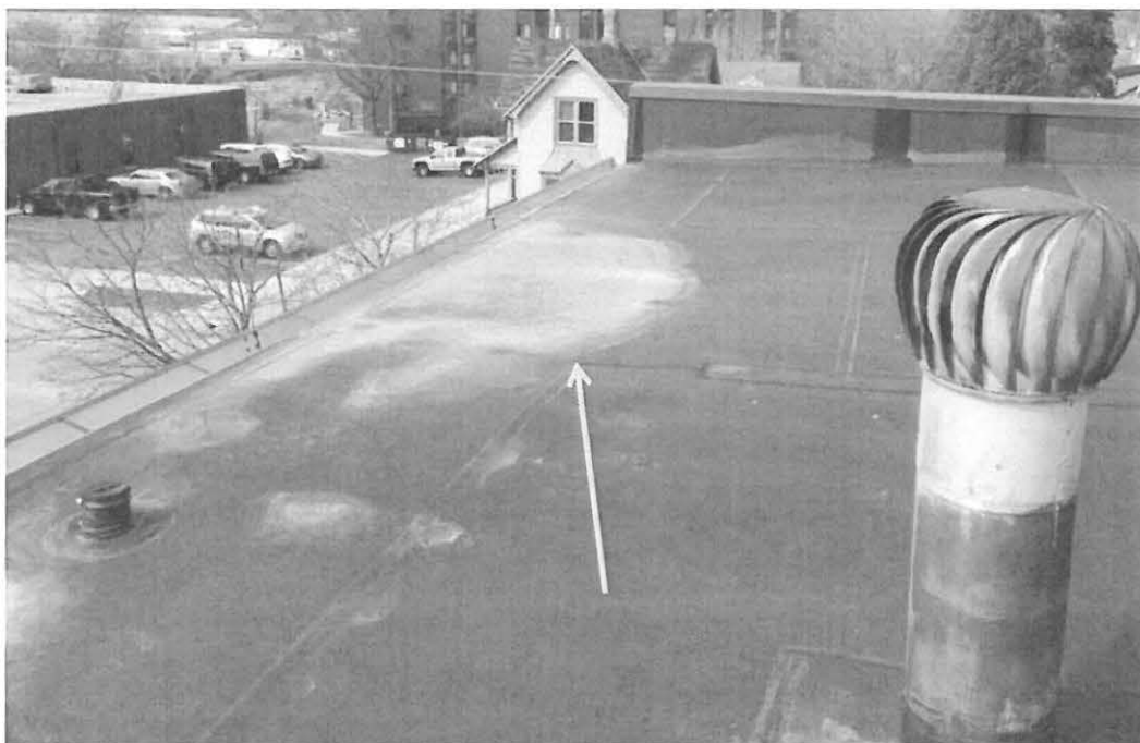
Figure 18: Ponding at south roof edge.
