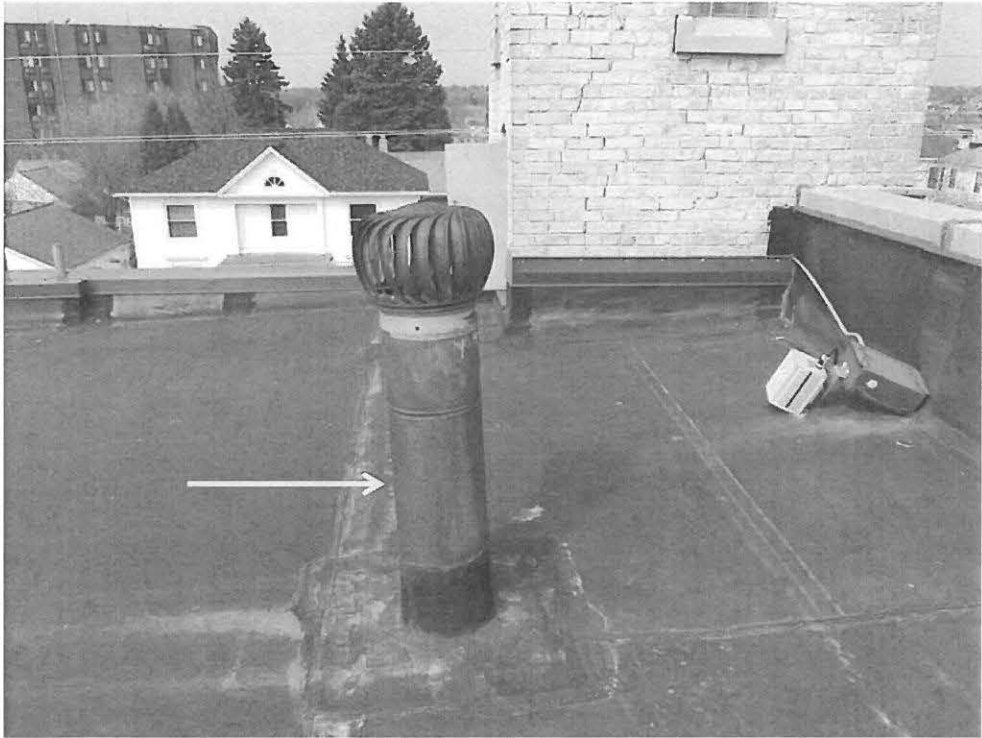
Figure 12: Corroded metal vent.
