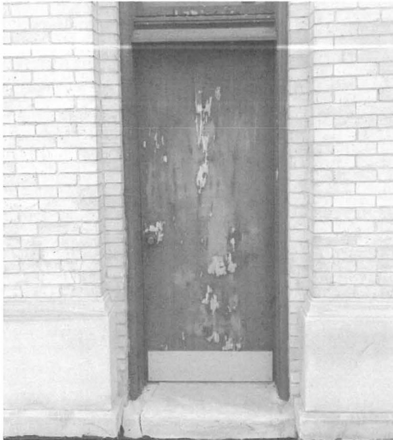
Figure 23: Deteriorating wood door.
