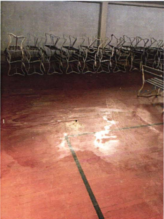
Roof leaking damage on gym floor
