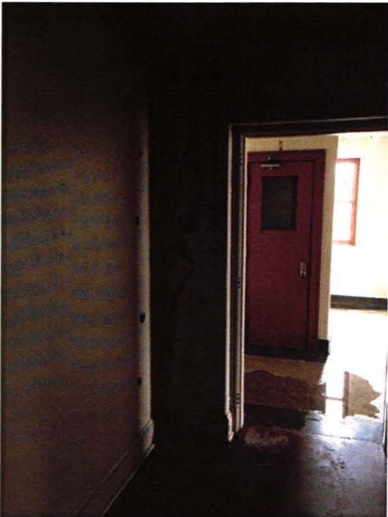
New damage from Winter 2016-2017
