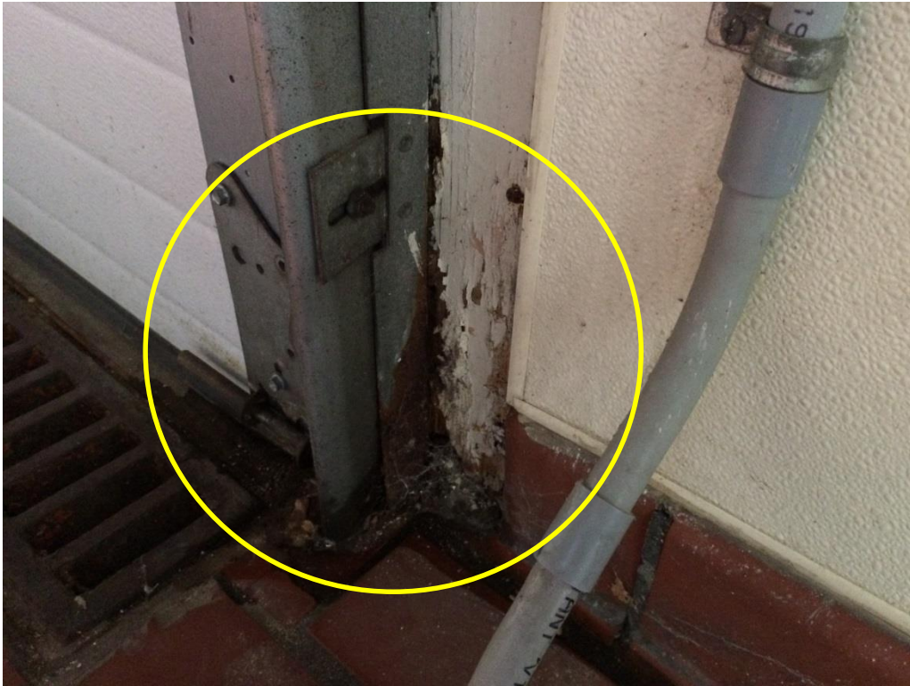
Figure 49: Deterioration of wood trim at garage door.
