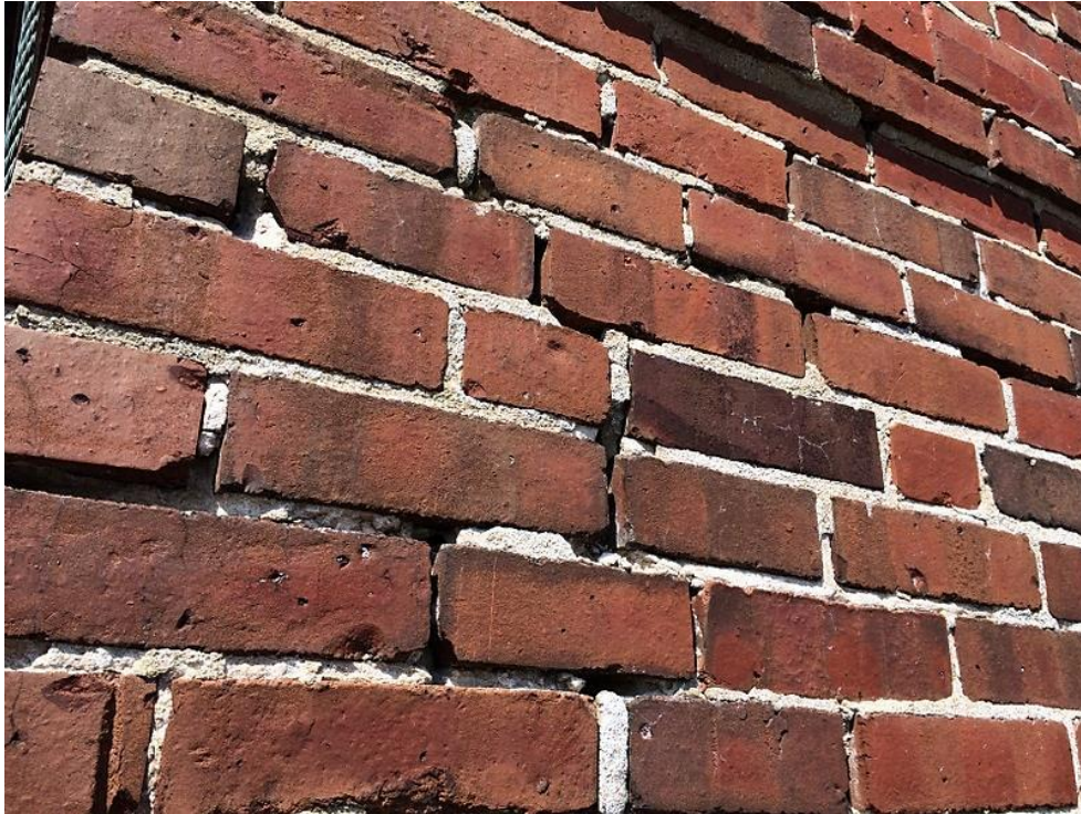
Figure 41: Brick/mortar deterioration on building facade
