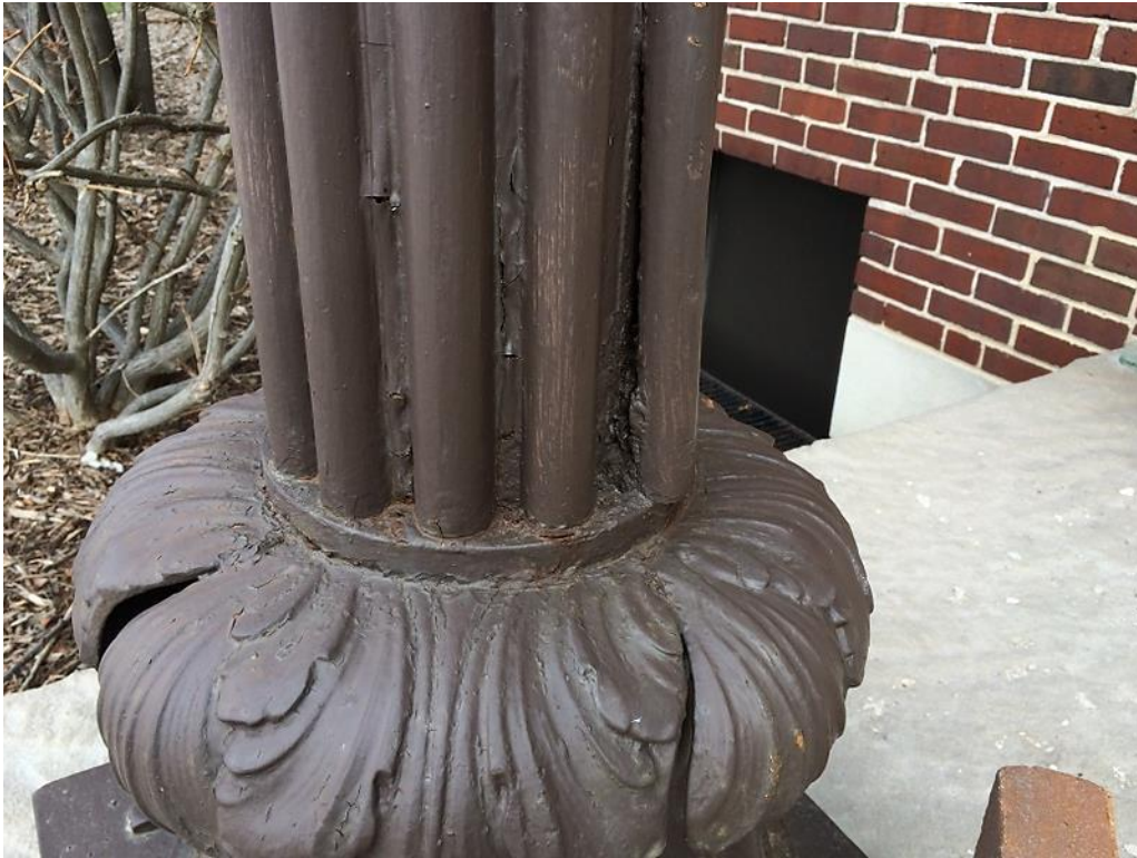
Figure 15: Corrosion/peeling paint on light poles at main entrance on south elevation
