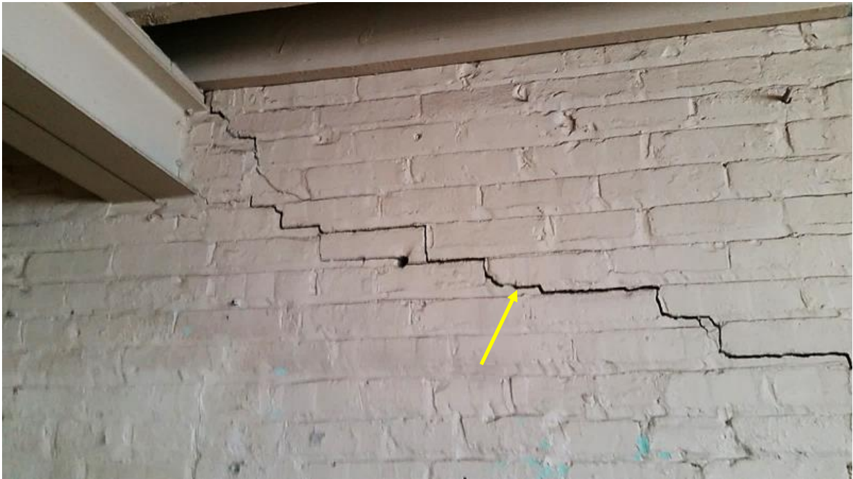
Figure 32: Interior brick cracking.
