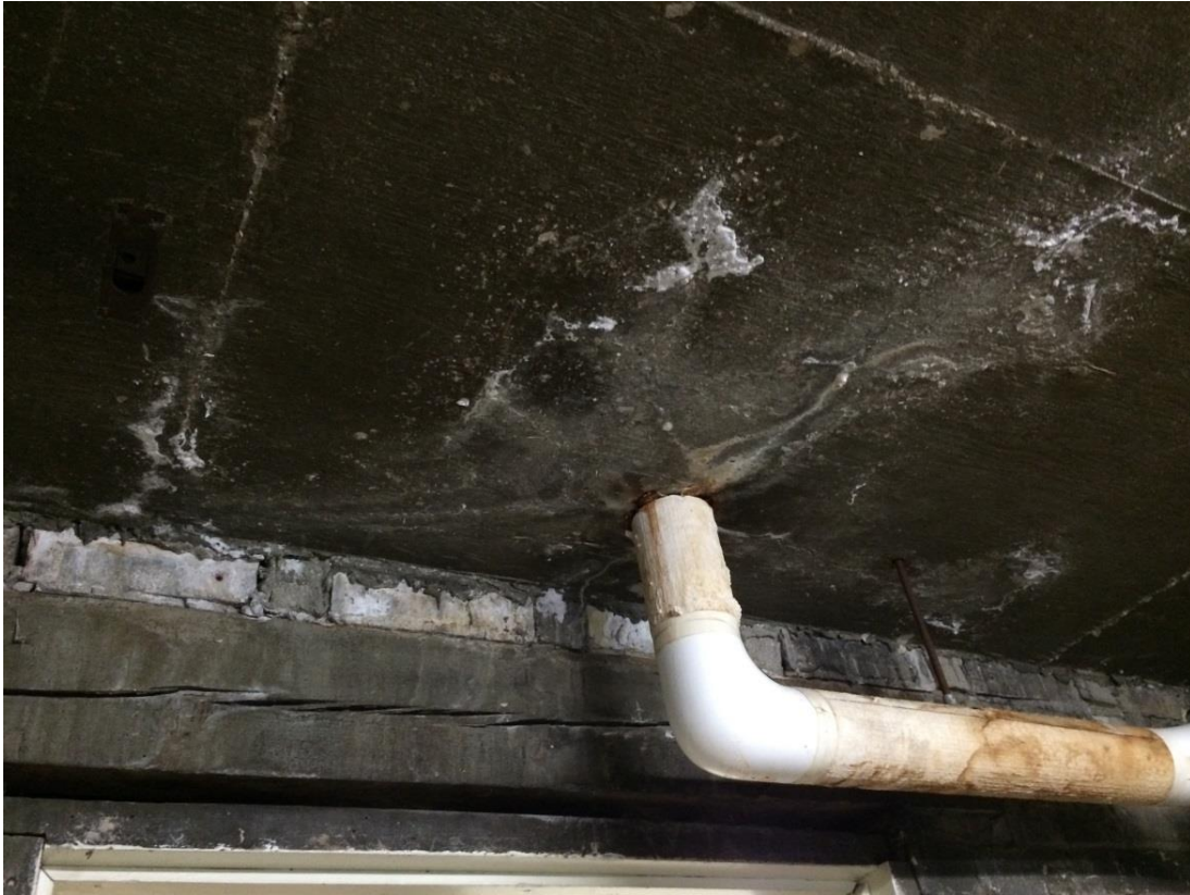
Figure 45: Corrosion, spalls and efflorescence due to leaking at floor drain.
