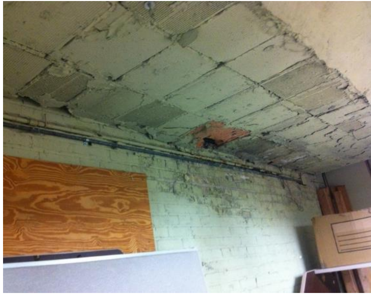
Figure 59: Deterioration, water leakage beneath west entrance stair
