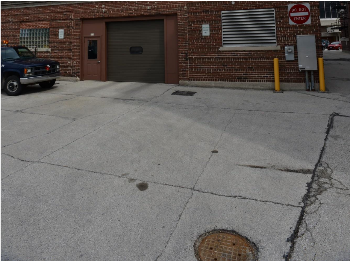
Figure 7: Deteriorating asphalt paving.
