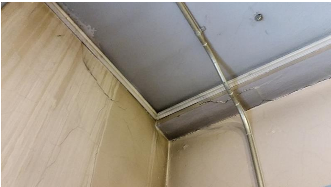
Figure 76: Fourth floor wall paint cracking
