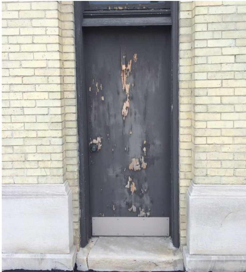
Figure 23: Deteriorating wood door.
