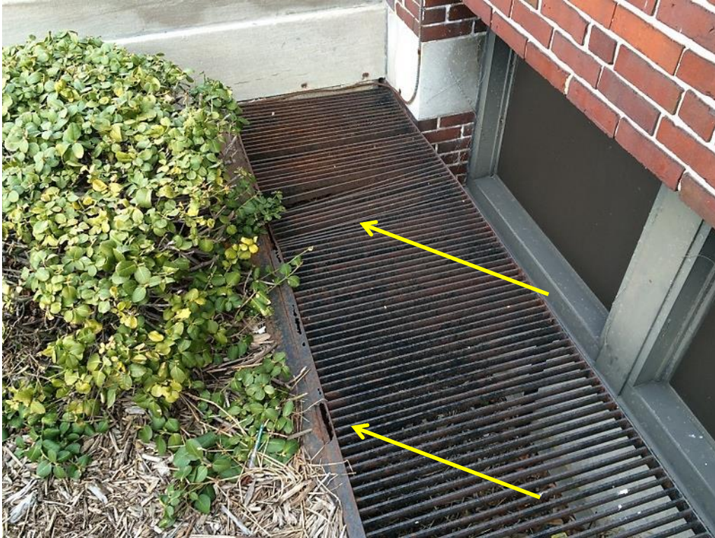
Figure 17: Corroded/damaged window well grate
