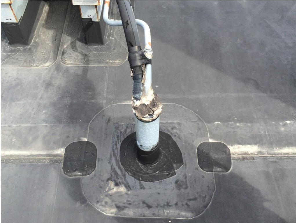
Figure 15: Deteriorated seal at A/C line penetration.
