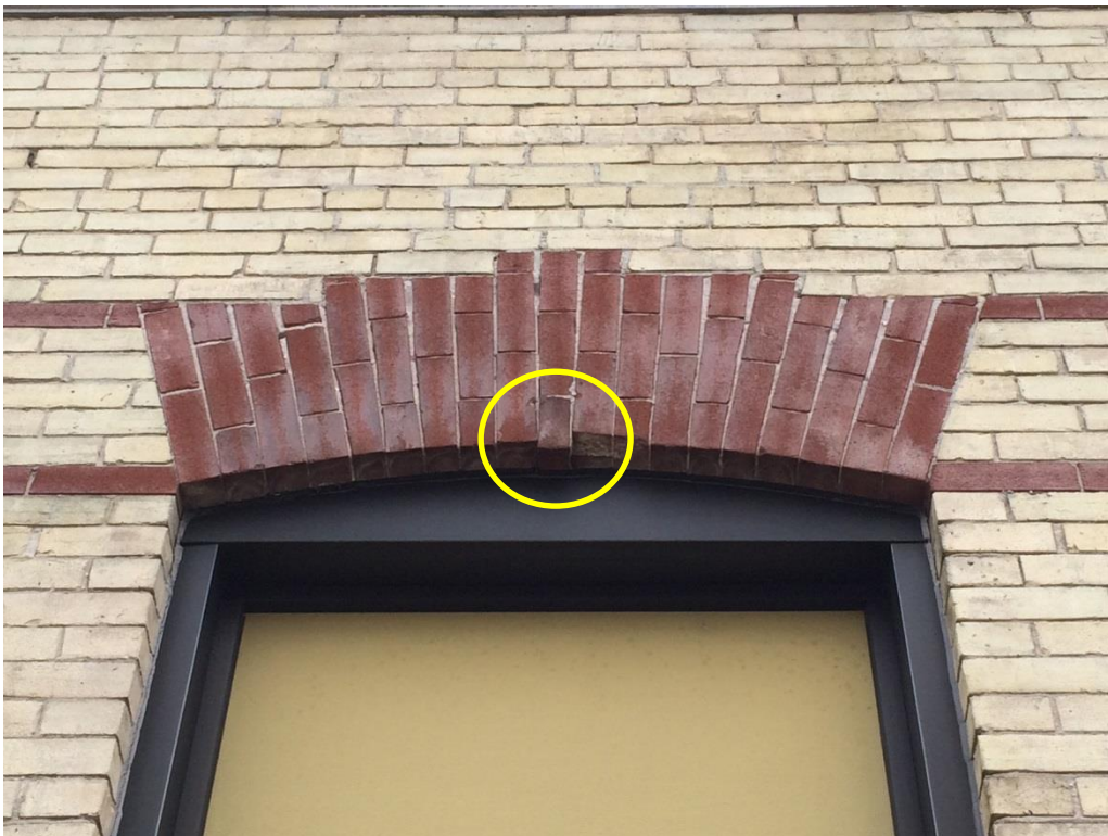
Figure 26: Loose brick unit.
