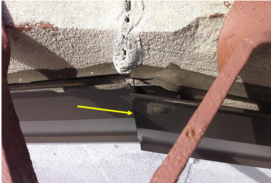
Figure 11: Open joint between metal counter flashings.
