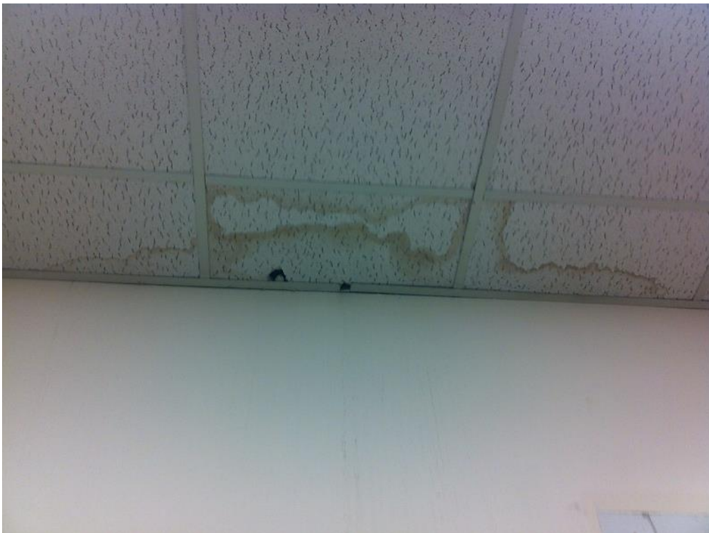
Figure 64: Damaged ceiling tiles showing signs of leaks
