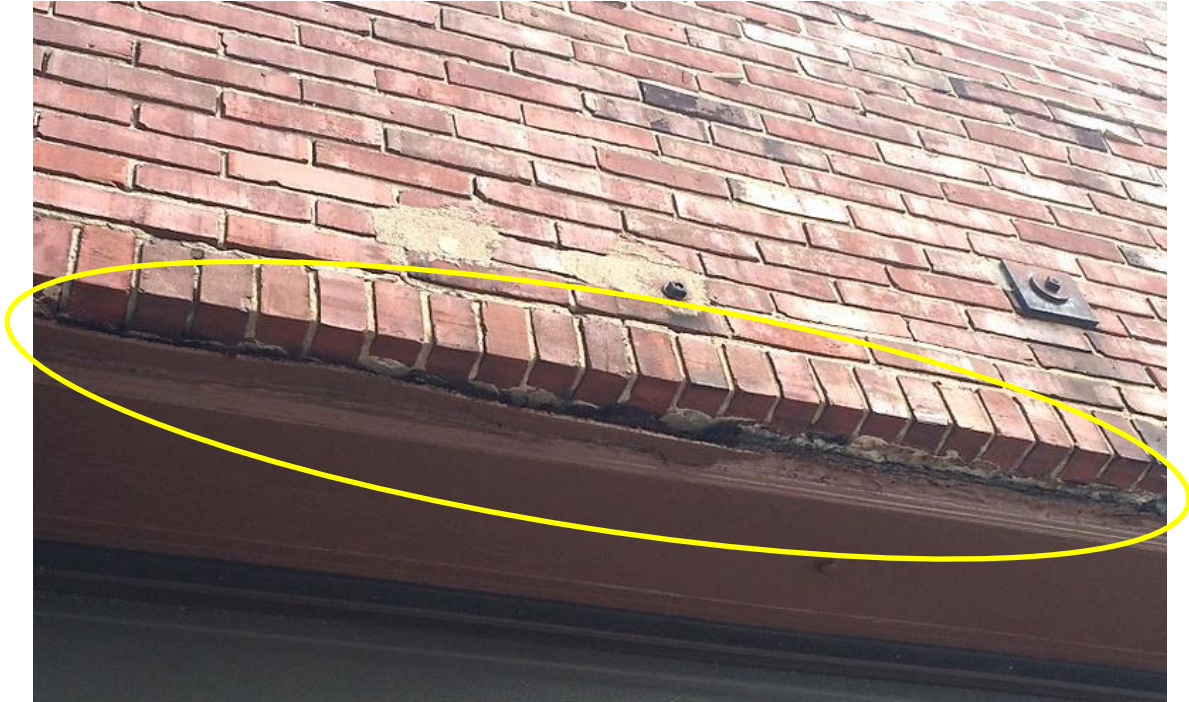
Figure 29: Corroded steel door lintel.
