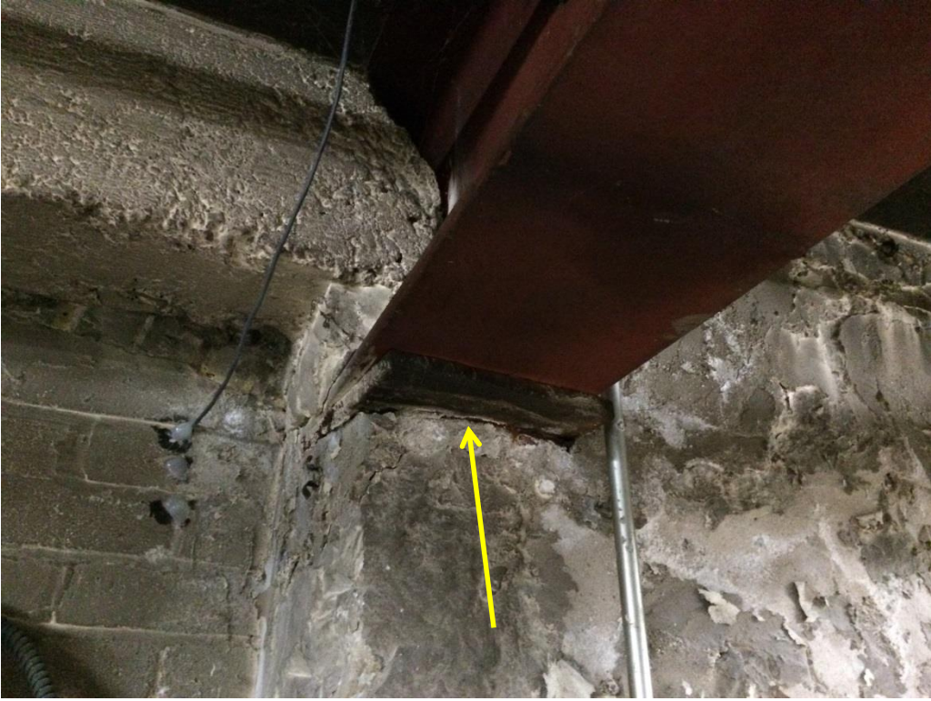
Figure 37: Corrosion of steel beam.
