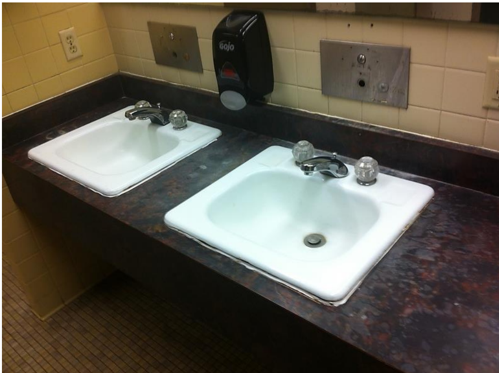
Figure 66: Aged bathroom fixtures
