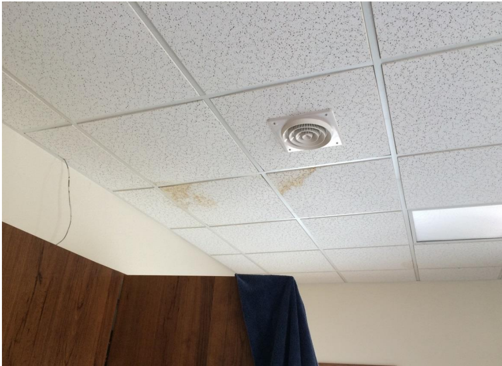
Figure 47: Stained ceiling tiles.
