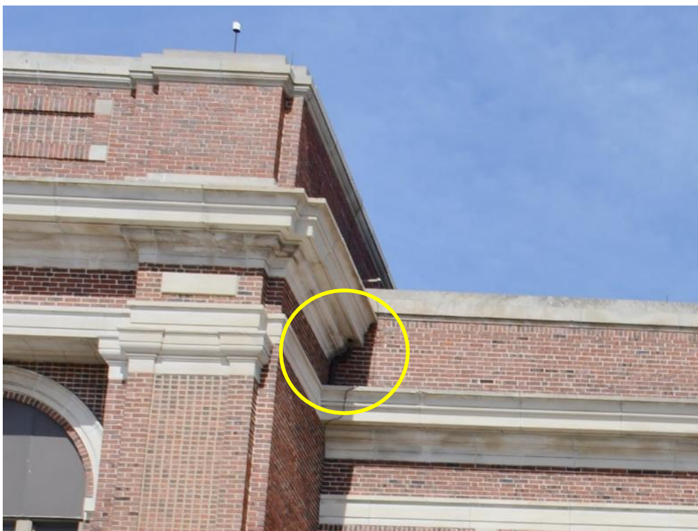
Figure 14: Disconnected downspout, south facade
