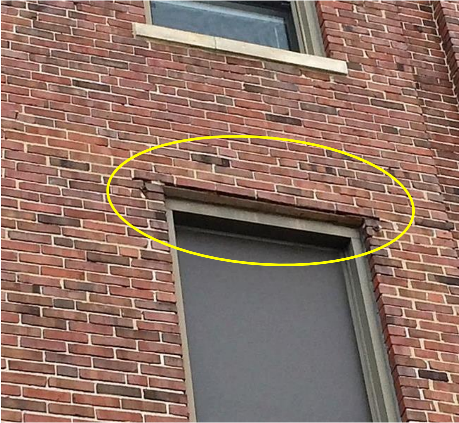
Figure 37: Corroded lintel causing brick movement.
