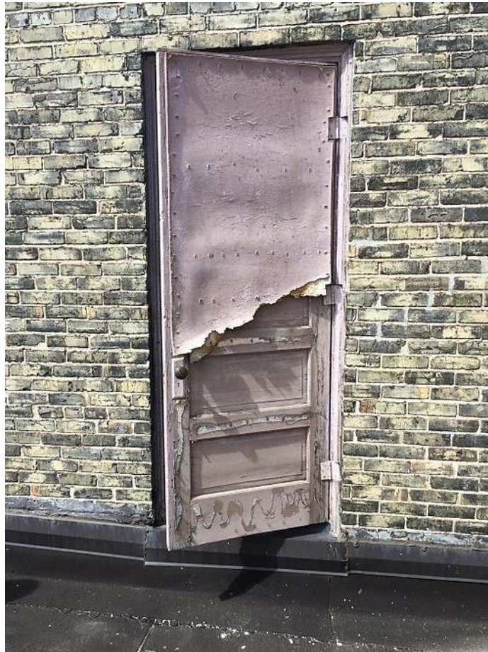
Figure 34: Damaged roof access door
