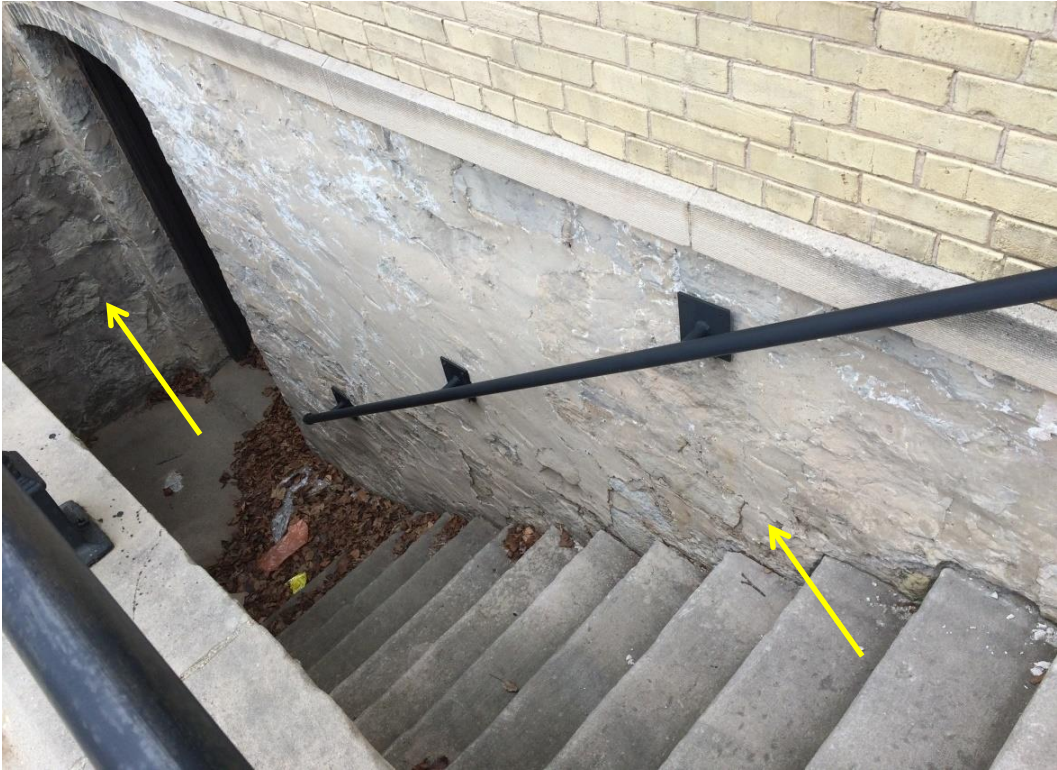
Figure 7: Deteriorated foundation walls.
