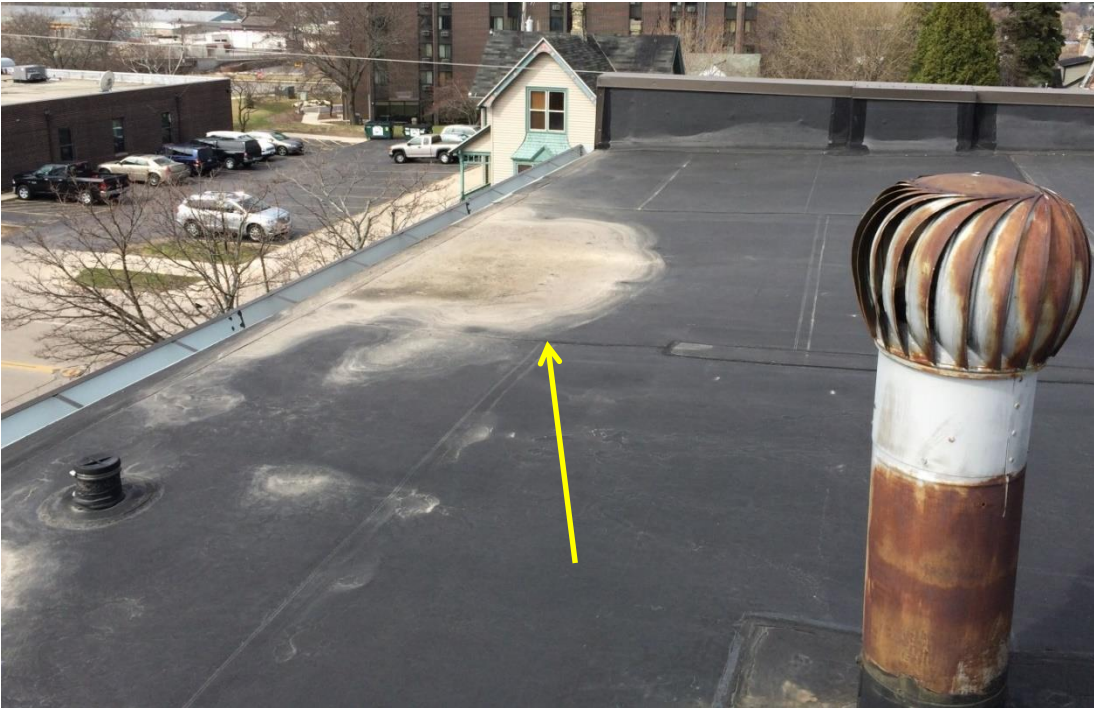
Figure 18: Ponding at south roof edge.
