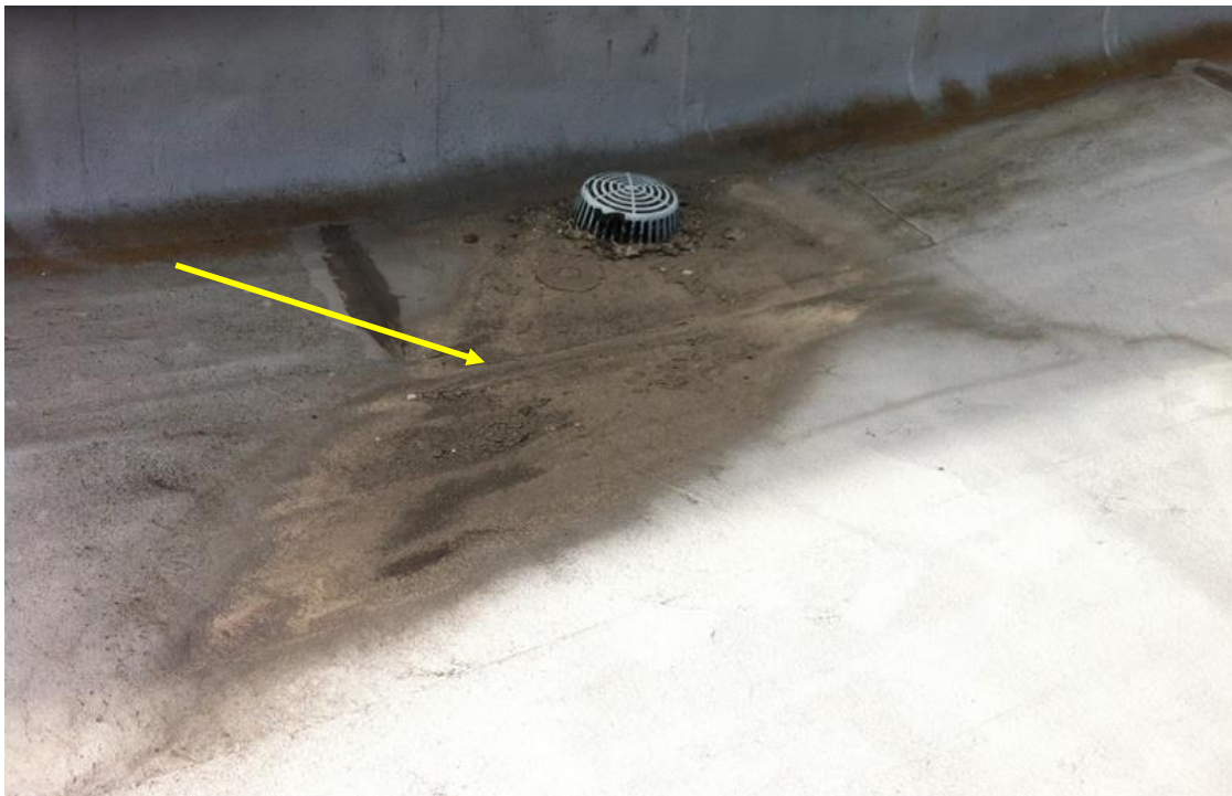
Figure 16: Ponding at roof drain.
