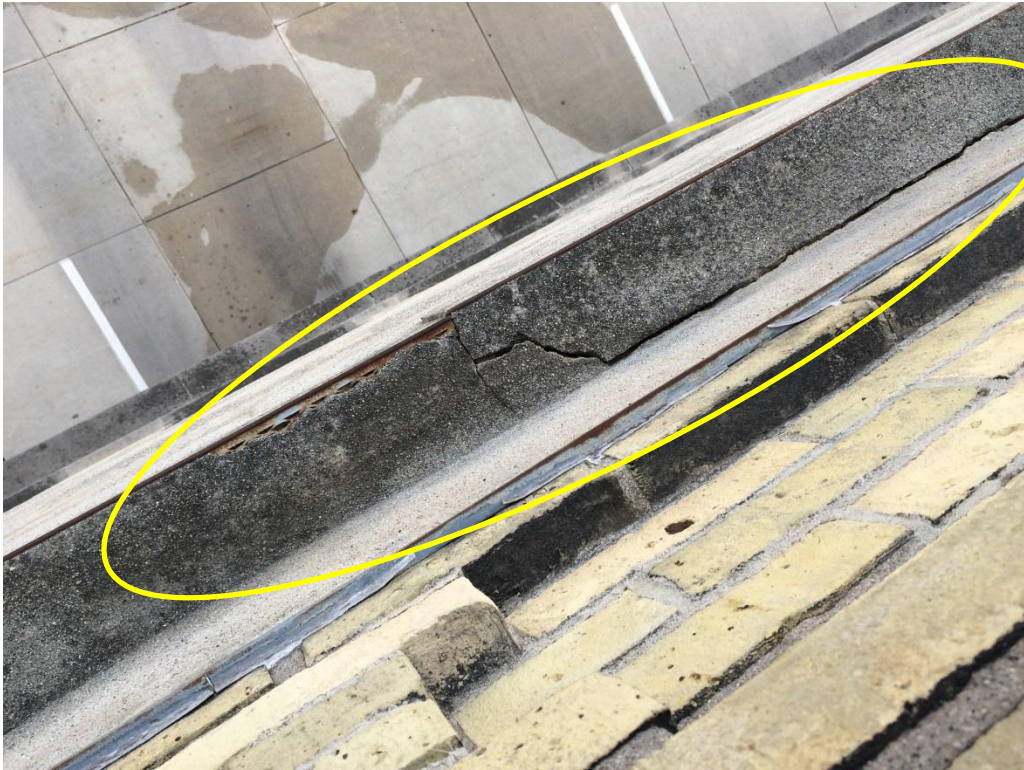
Figure 29: Deteriorating cementitious parge coating.
