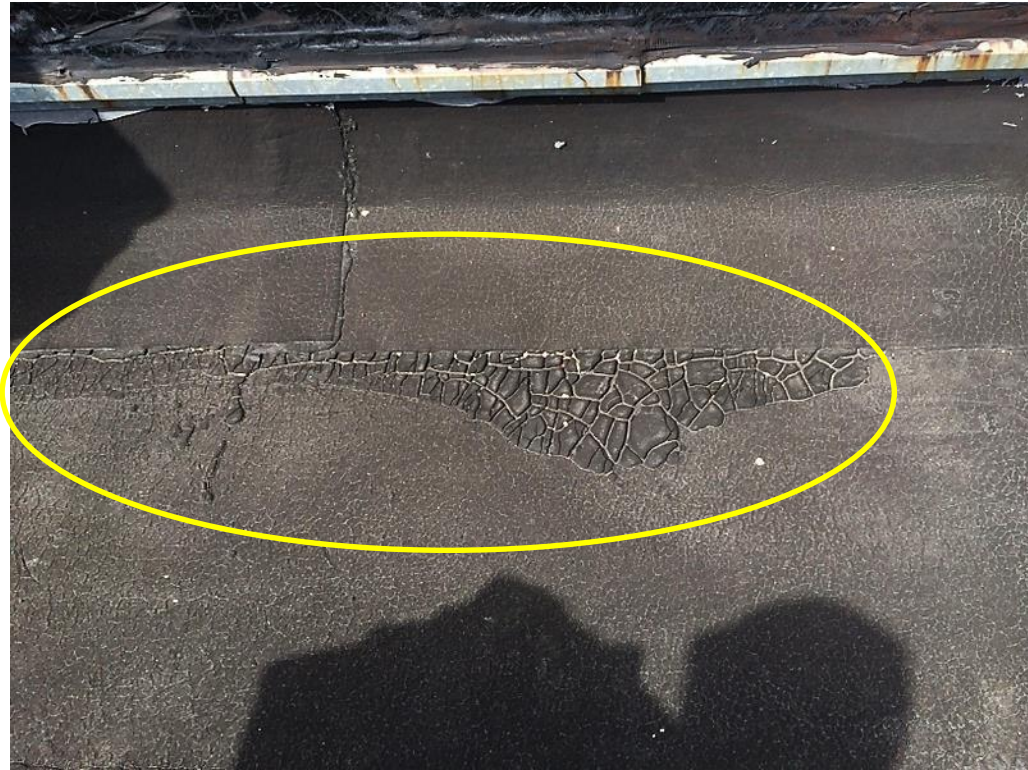
Figure 25: Deteriorated/asphalt cracking at modified bitumen membrane surface.
