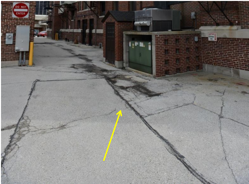
Figure 13: Deteriorating asphalt pavement at alley, north elevation
