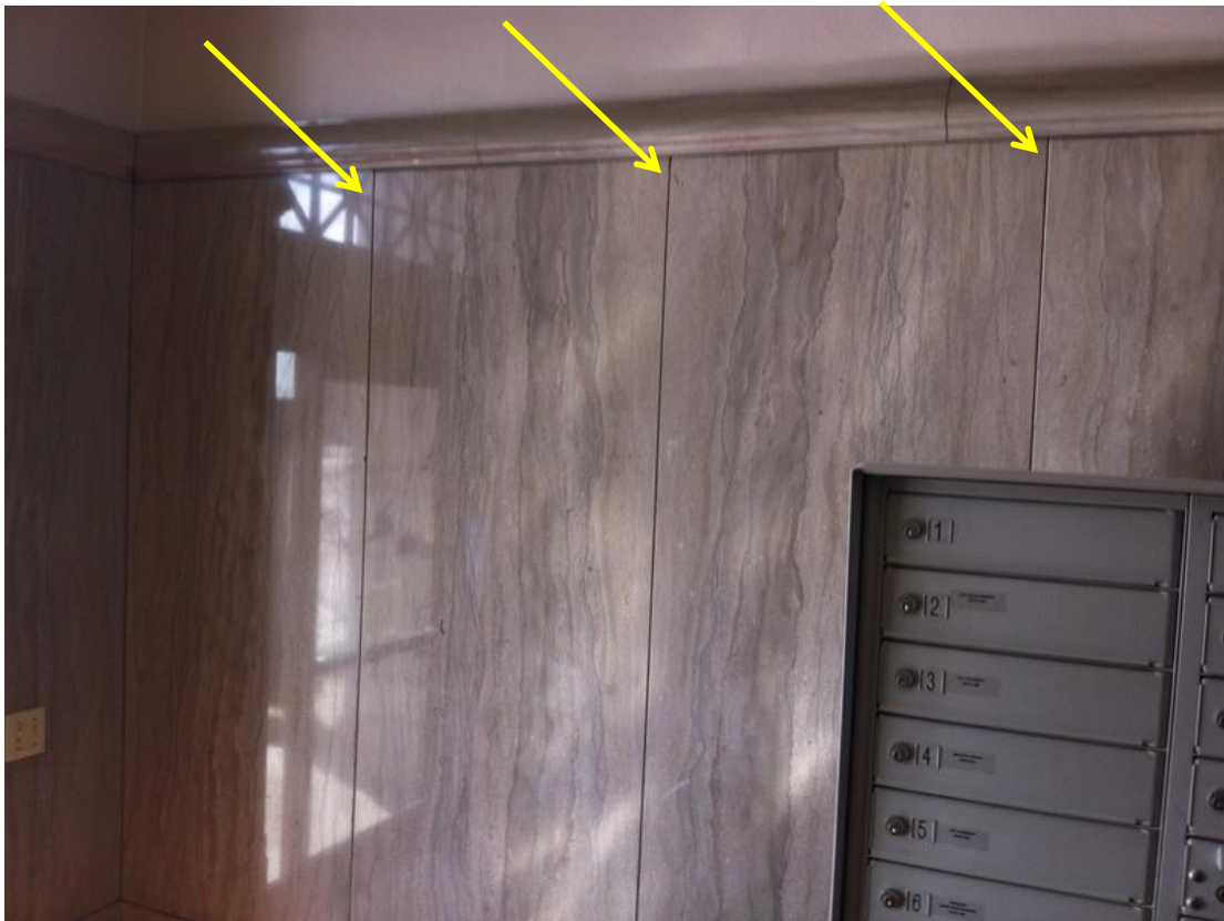
Figure 69: Marble joints missing and deteriorated sealant
