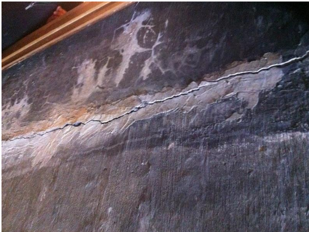
Figure 62: Foundation cracking in north basement exit stairwell
