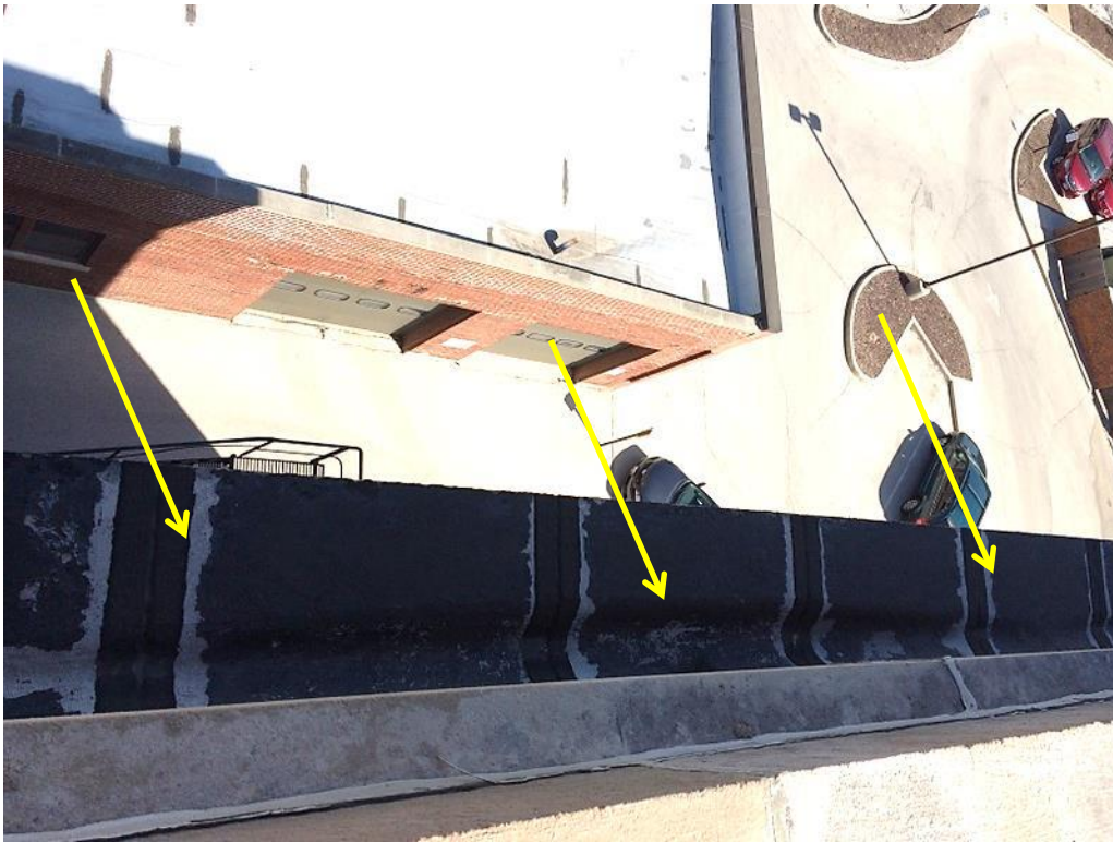
Figure 47: Deteriorated asphalt coating on skyward facing cornice/gutter.
