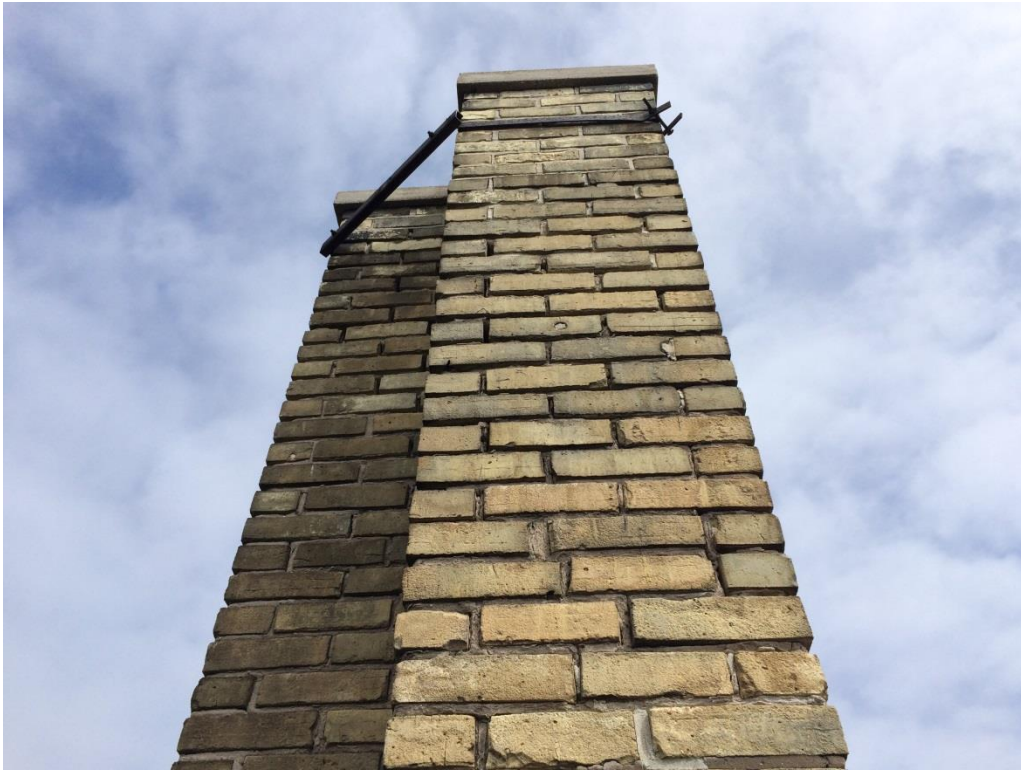
Figure 25: Deteriorated brick at chimney.
