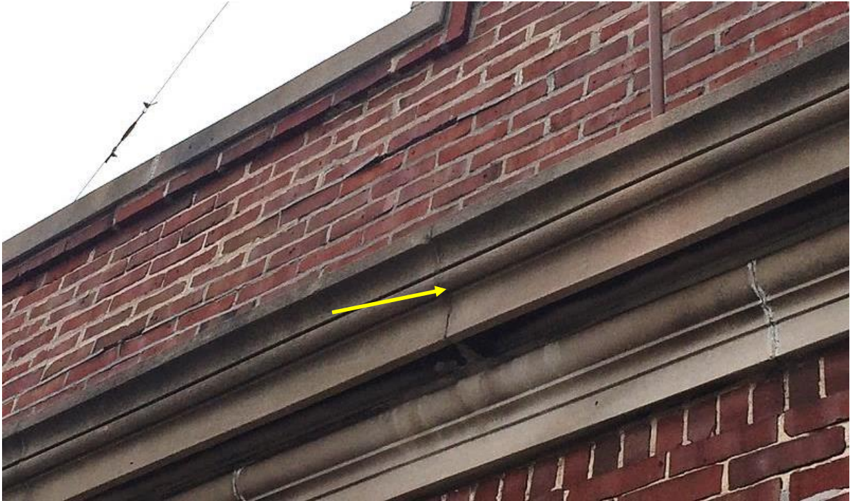
Figure 31: Mortar joint deterioration on stone.
