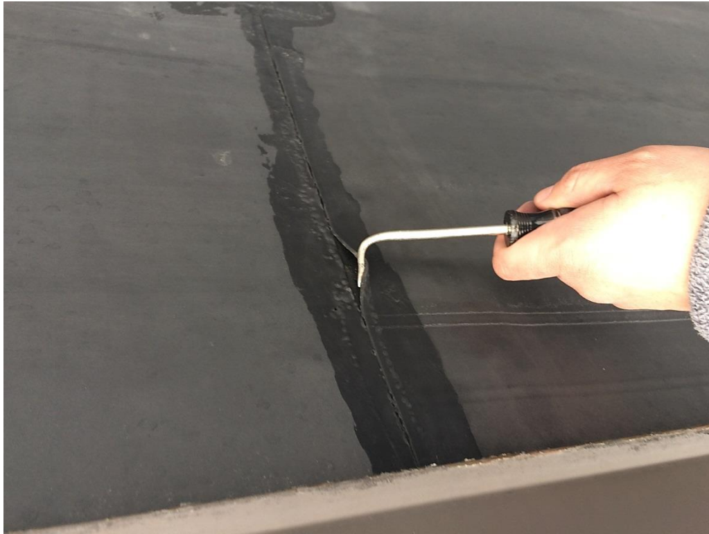
Figure 11: Open roof seam.
