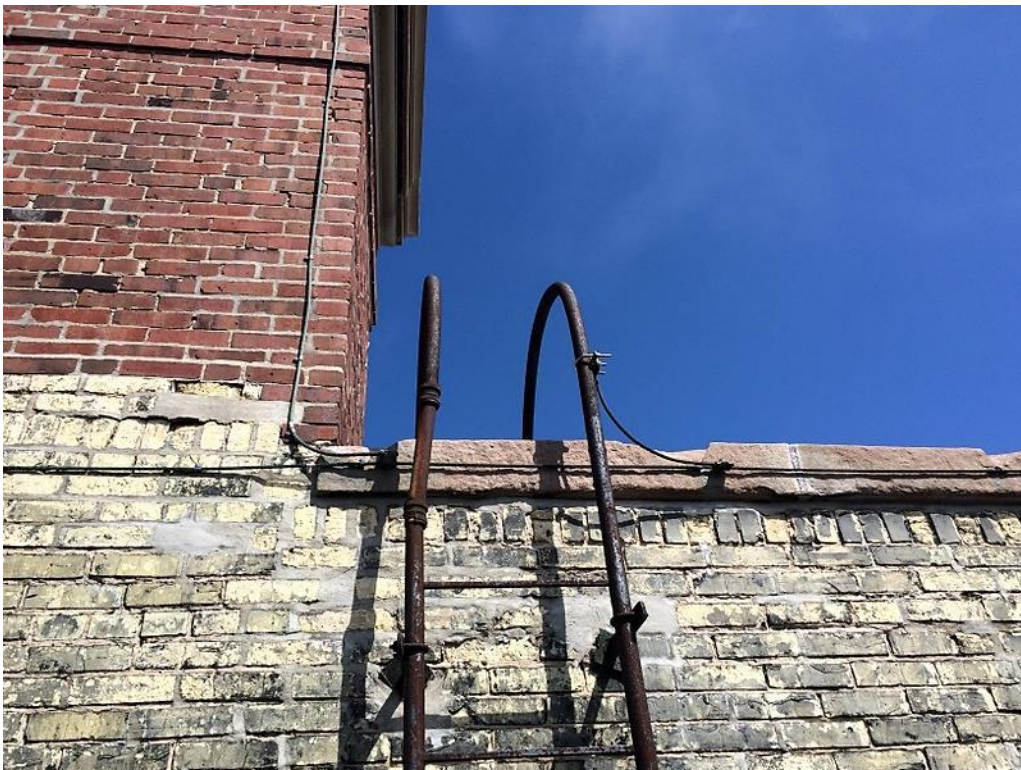
Figure 16: Corroded/damaged fire escape
