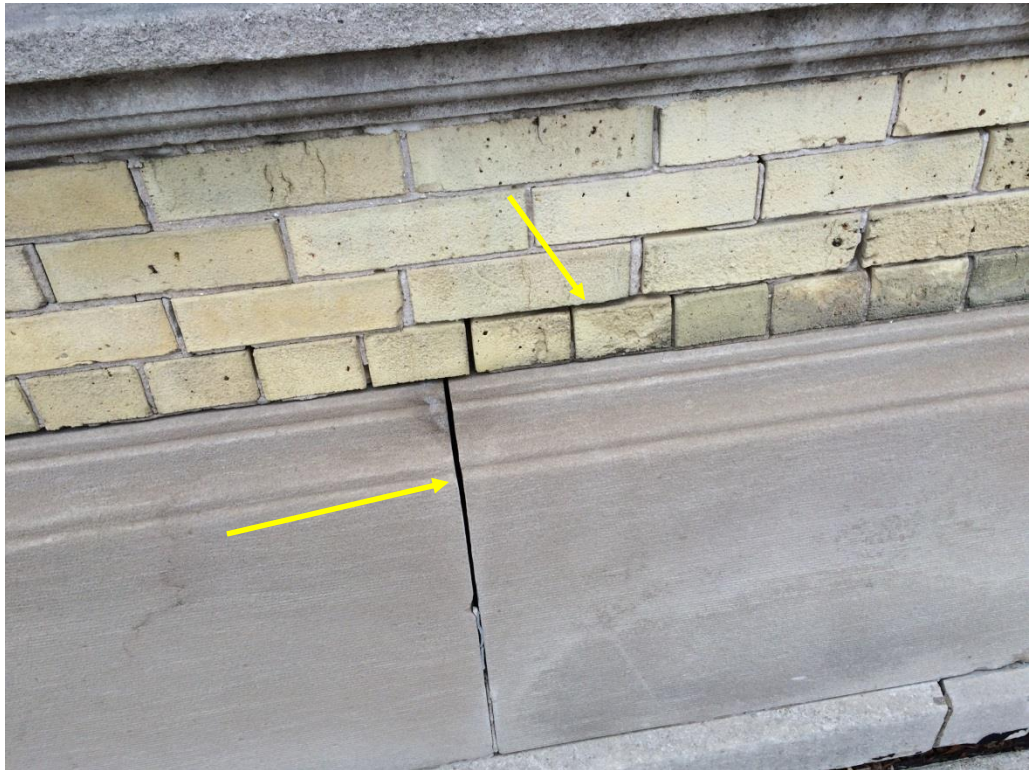
Figure 28: Deteriorated and open mortar joints.
