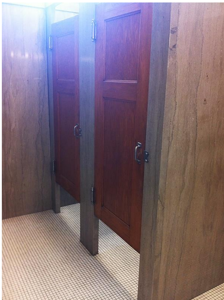
Figure 68: Second floor women's restroom, not ADA accessible
