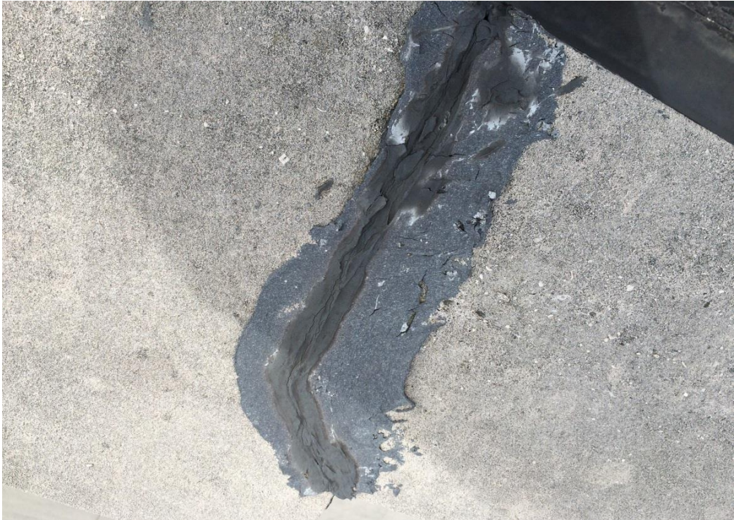
Figure 9: Deteriorated stone coping sealant.
