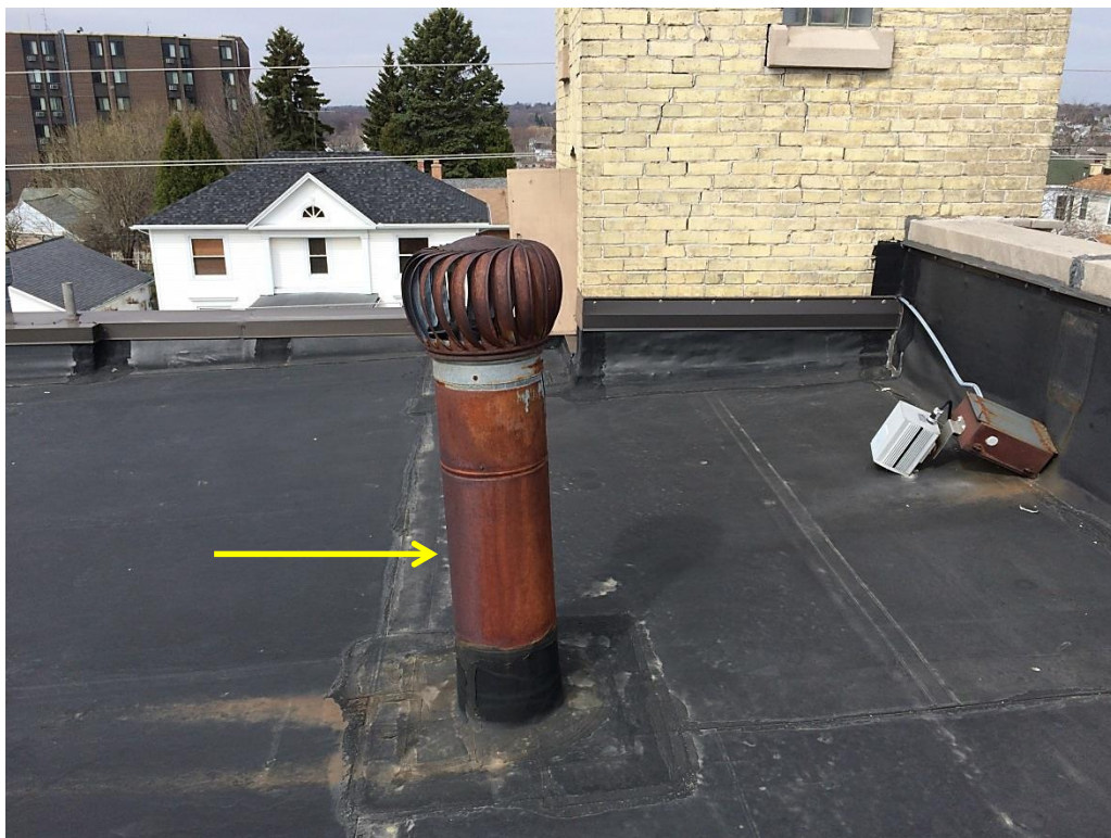
Figure 12: Corroded metal vent.
