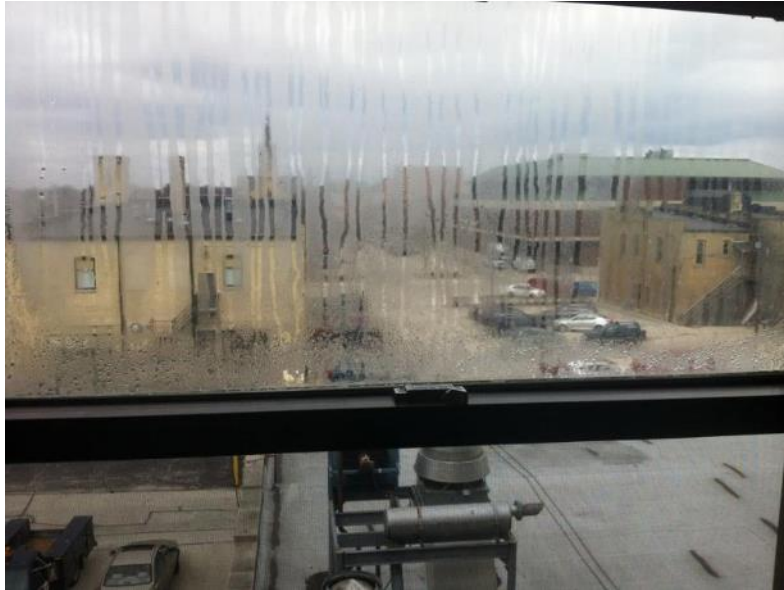
Figure 31: Condensation in between window panes of IGU.
