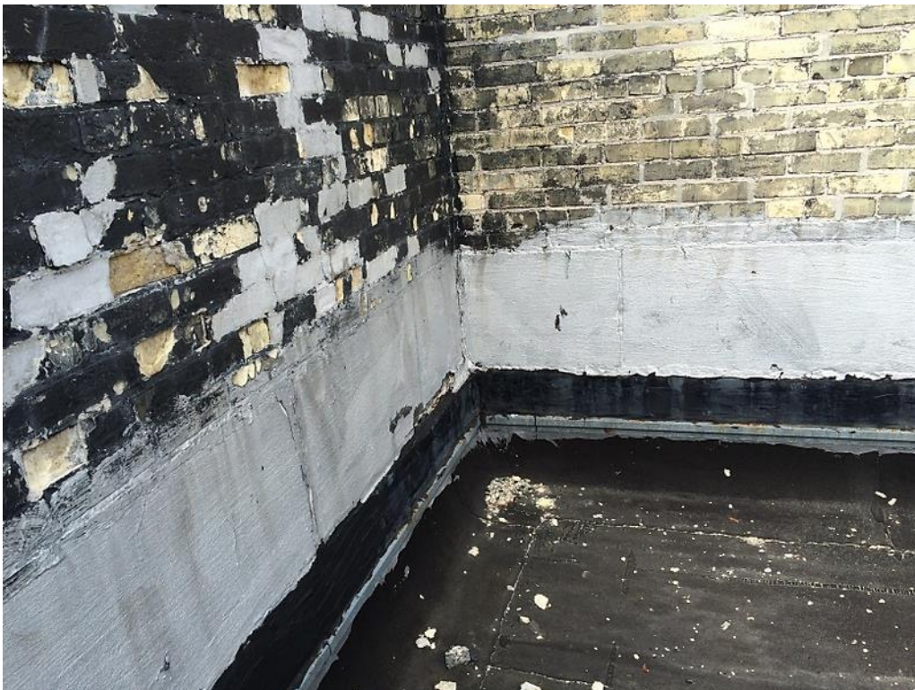
Figure 48: Deteriorated brick at inside face of parapet
