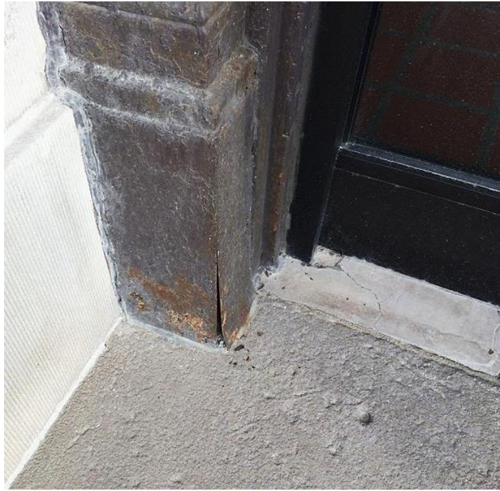
Figure 35: Corroded and deteriorated door frame
