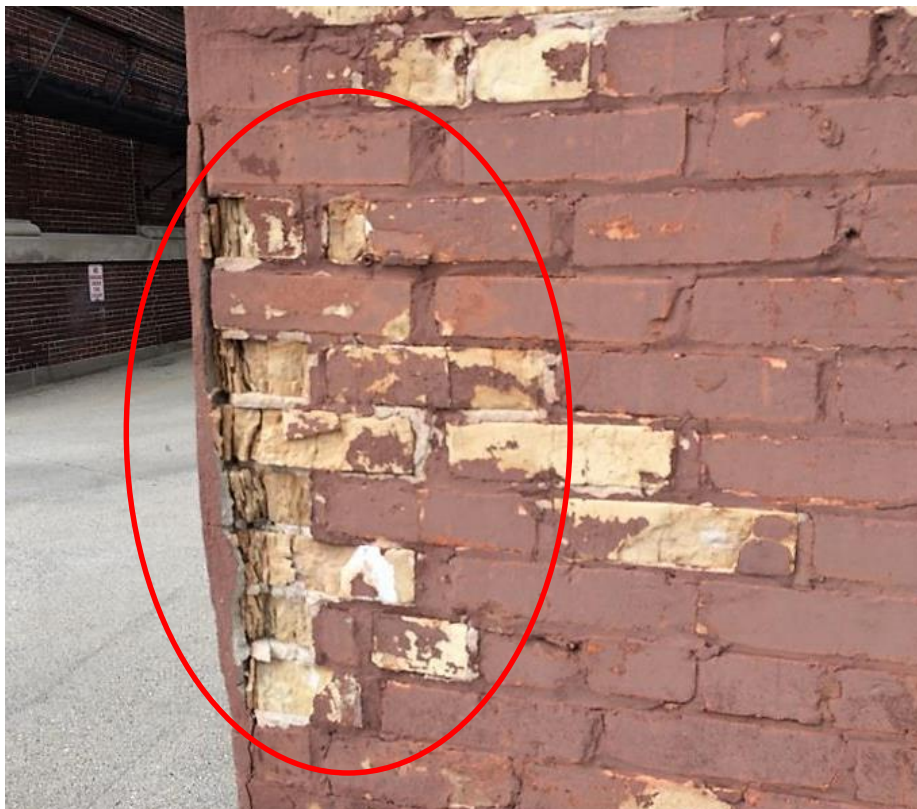
Figure 22: Deteriorated brick masonry.
