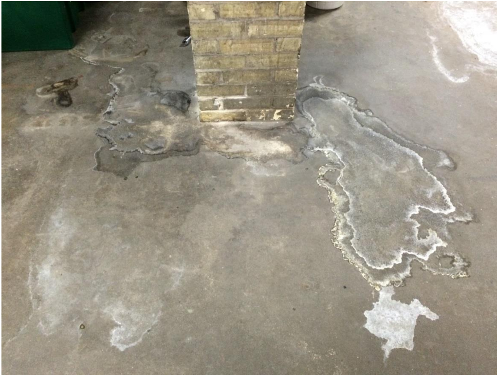
Figure 41: Water staining on floor.
