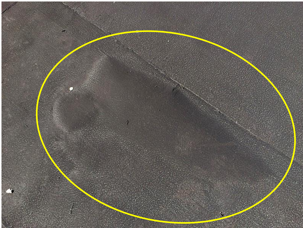
Figure 26: Blister within roof system.
