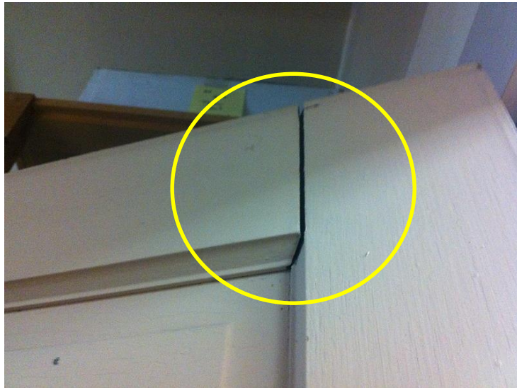
Figure 67: Door separating at joint
