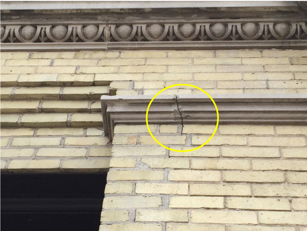
Figure 32: Cracked stone unit.
