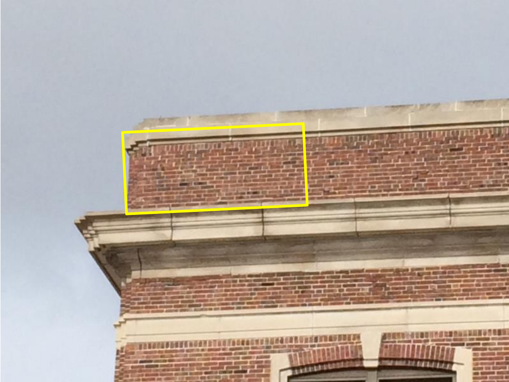
Figure 49: Out of plane brick movement
