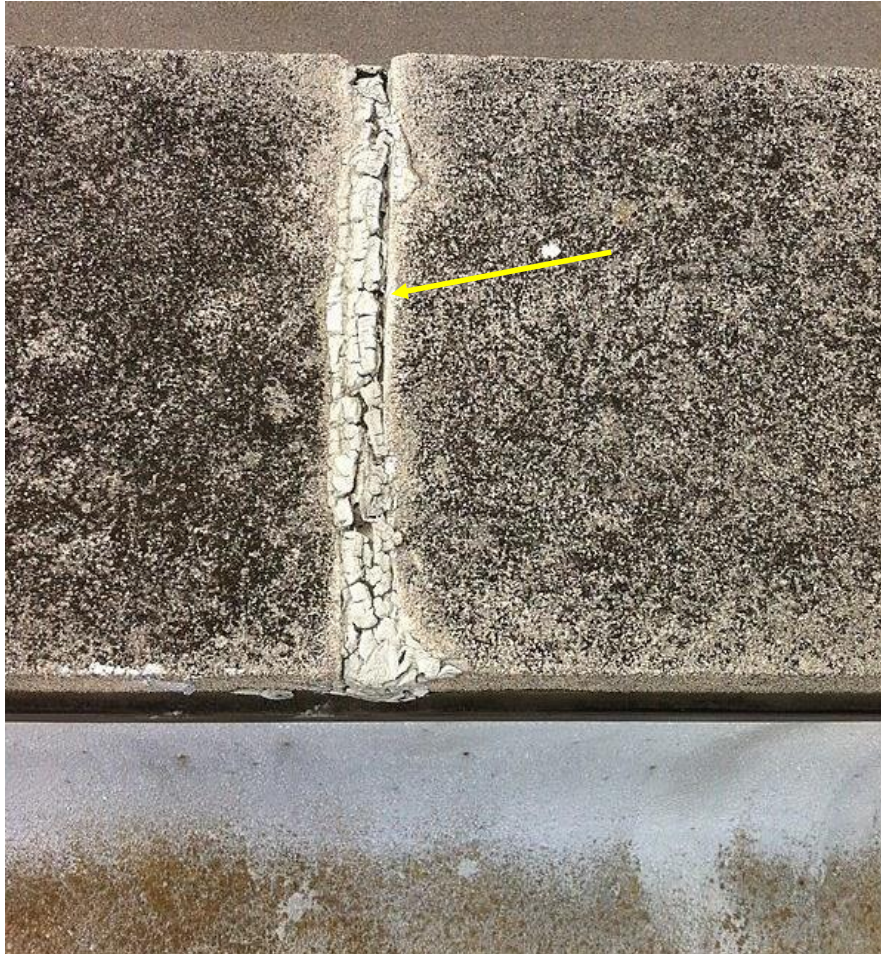
Figure 9: Failed skyward facing stone coping joint.
