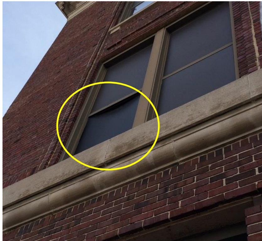
Figure 32: Detached window panel on west facade.
