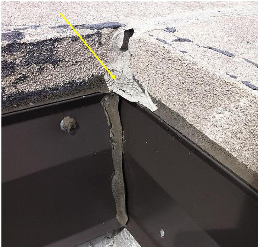
Figure 12: Open sealant joint at top of counter flashing.
