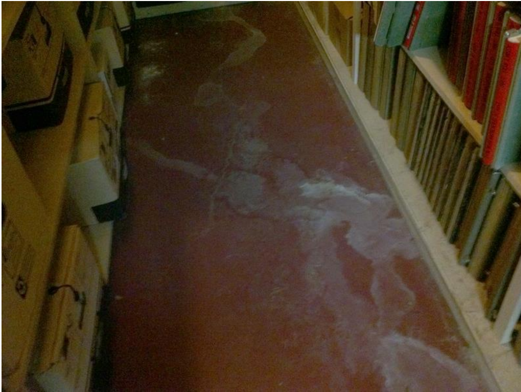
Figure 51: Efflorescence/water staining along basement floor
