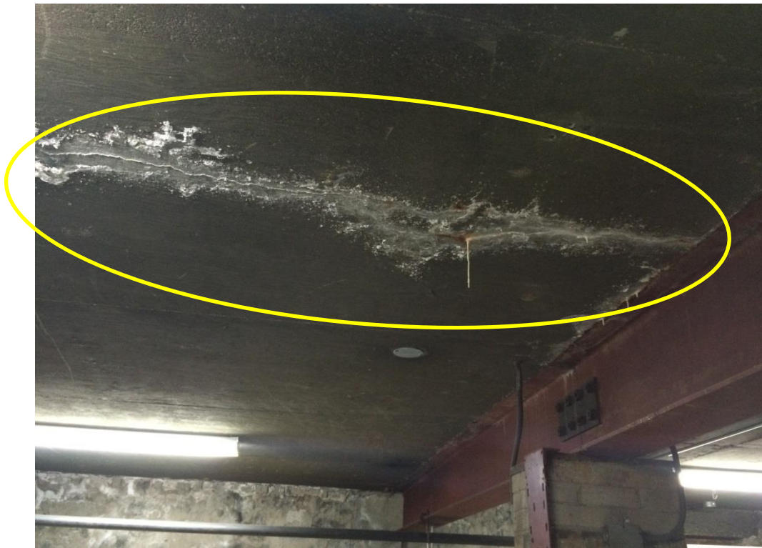
Figure 40: Efflorescence on ceiling.
