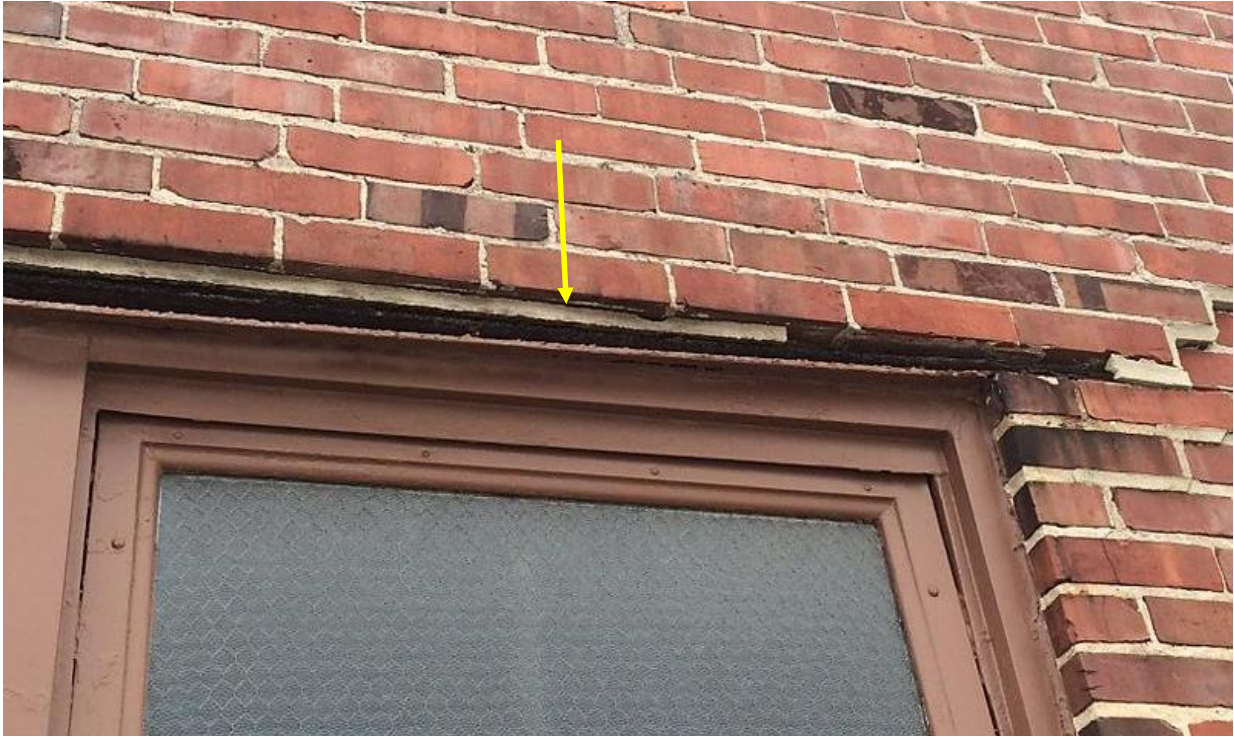
Figure 27: Corroded steel window lintel.
