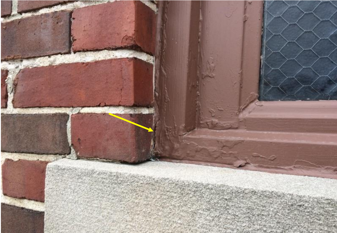
Figure 17: Window sealant deterioration.
