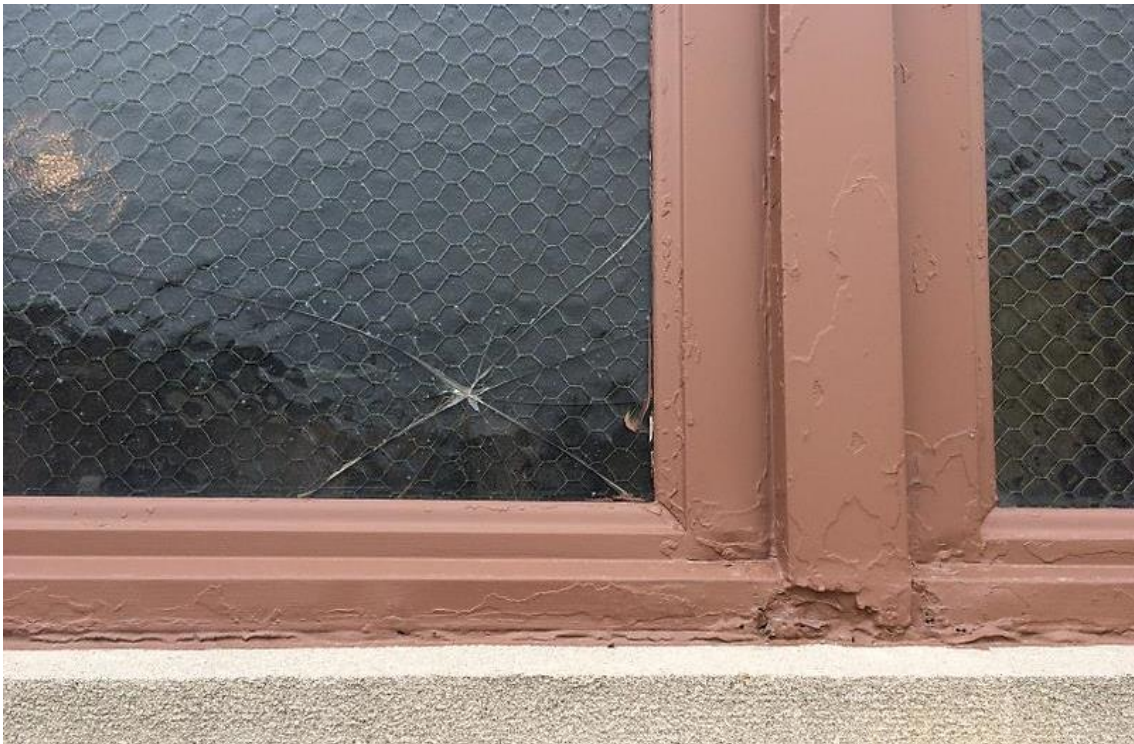
Figure 18: Cracked glass window pane.
