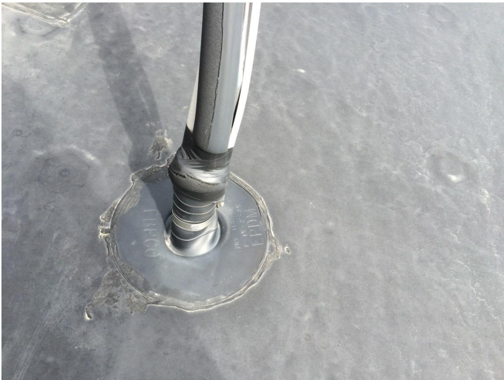
Figure 16: Improperly sealed A/C line penetration.
