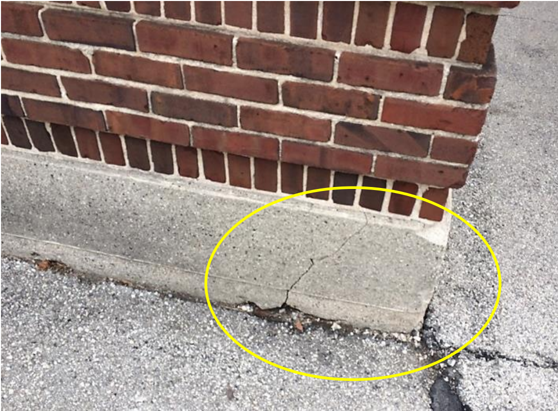
Figure 30: Cracked concrete foundation wall.
