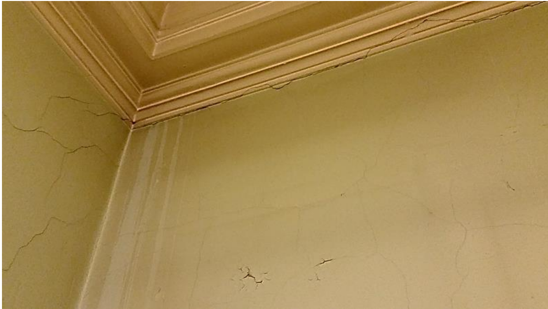
Figure 75: Fourth floor paint cracking
