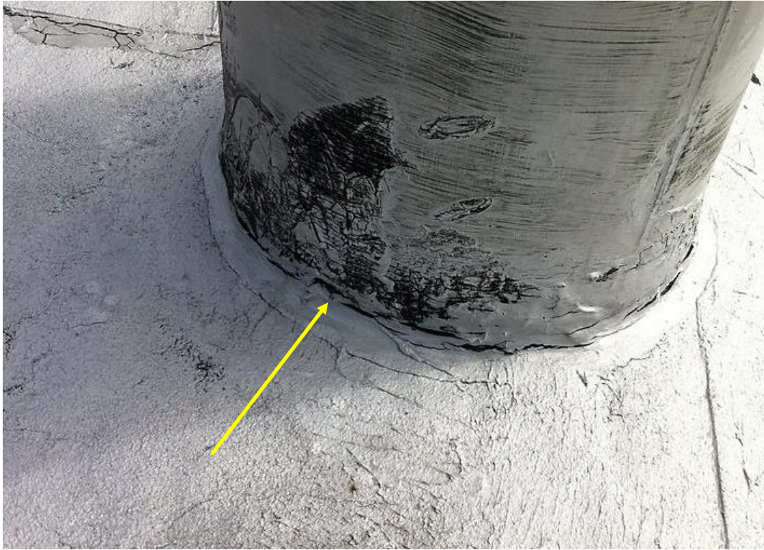
Figure 15: Failed joint at penetration.
