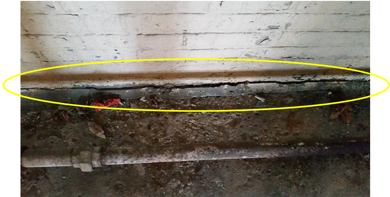
Figure 37: Failed floor to wall joint.
