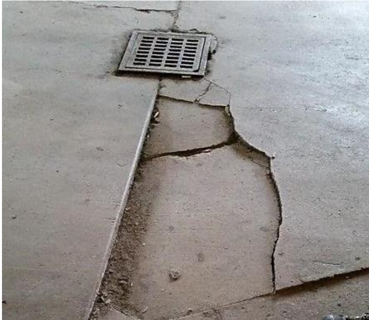
Figure 35: Concrete floor cracking.
