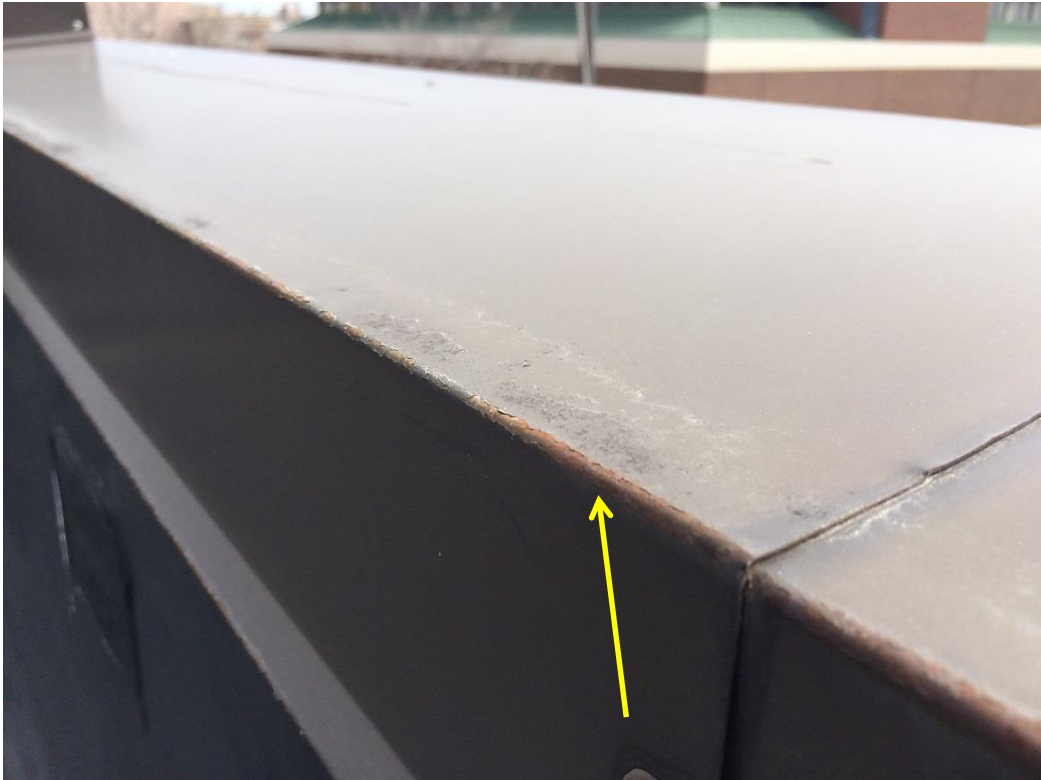
Figure 10: Coping paint deterioration.
