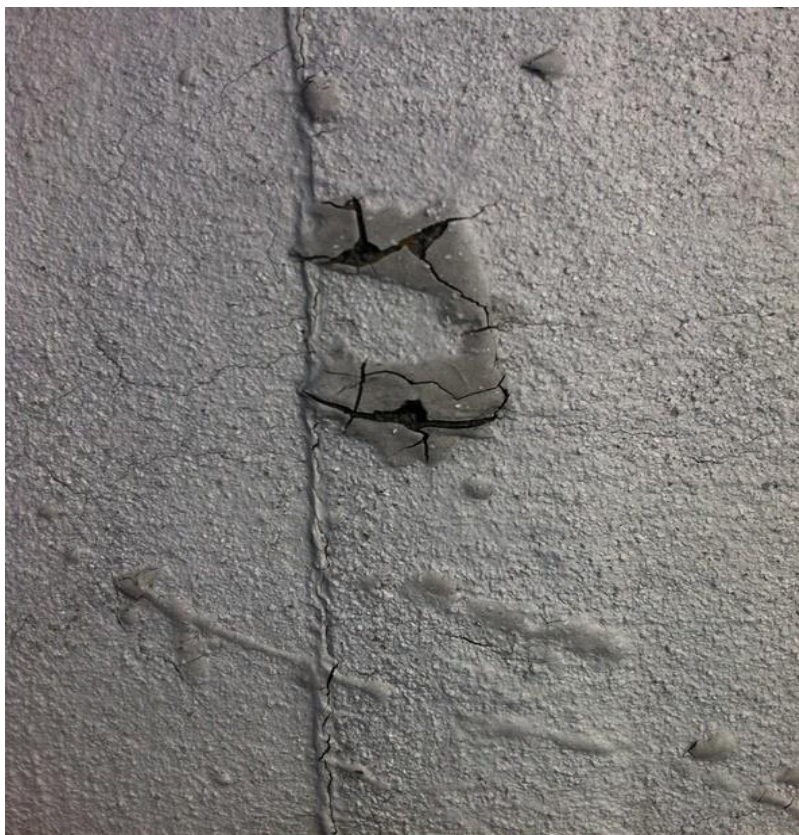
Figure 14: Membrane cracking and bubbling.
