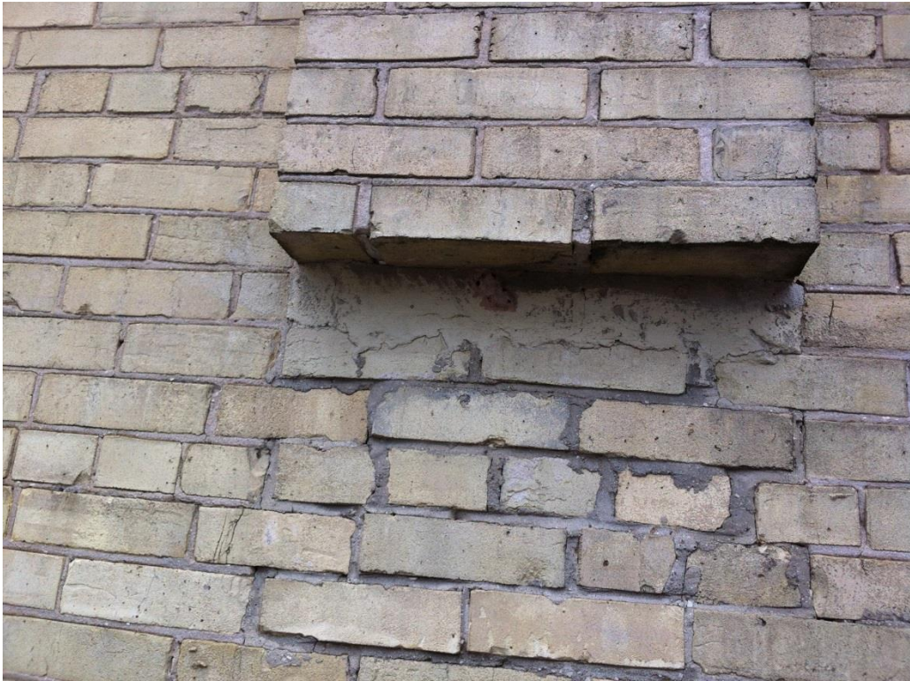
Figure 27: Deteriorated mortar joints.
