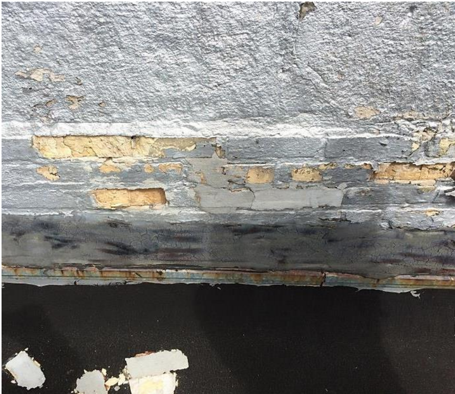
Figure 28: Failed aluminum coating above counter flashing
