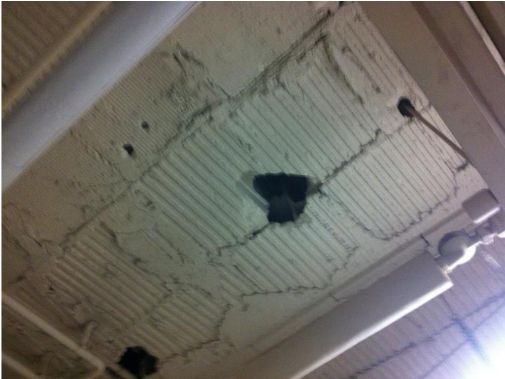
Figure 57: Hole in clay tile ceiling
