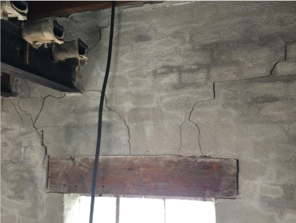
Figure 31: Interior cracking at lintel.
