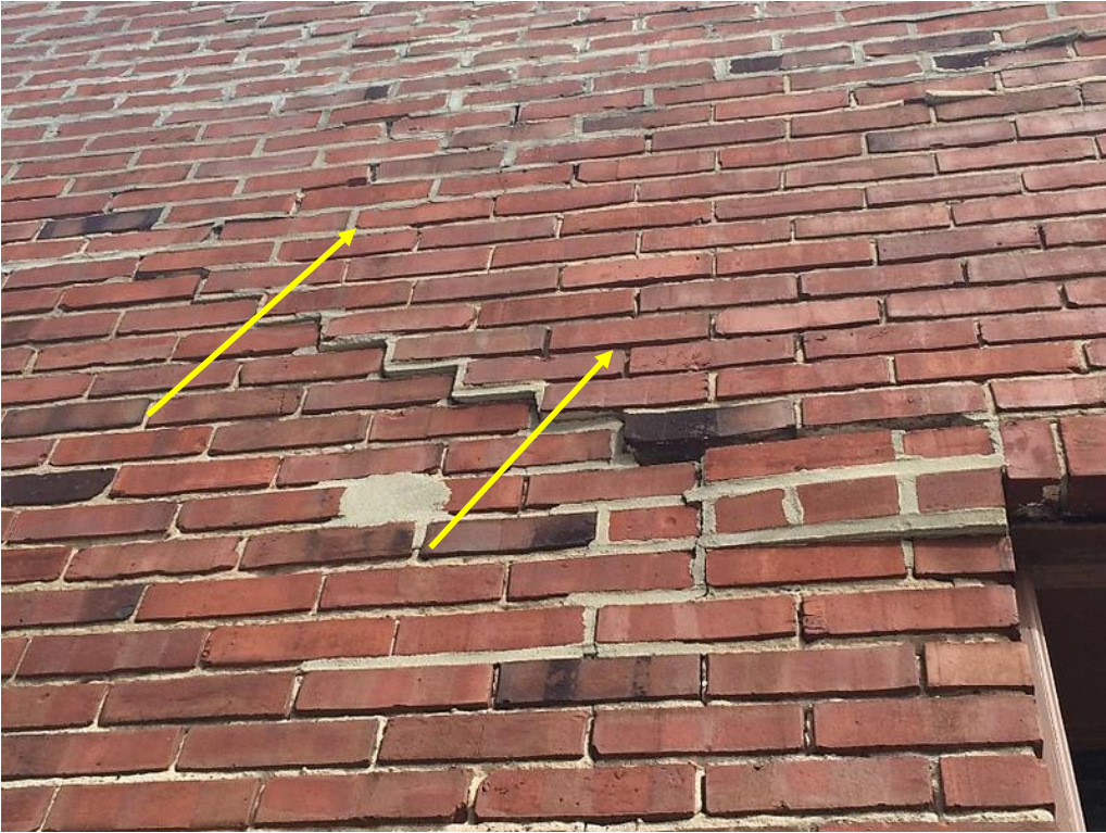
Figure 25: Out of plane brick movement.
