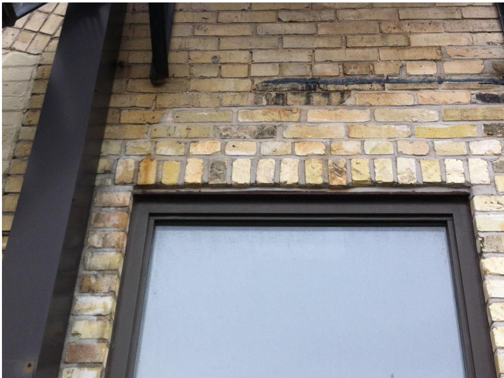
Figure 30: Corroded steel lintel.
