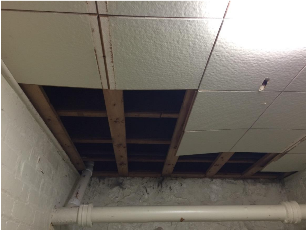
Figure 43: Missing ceiling tiles.
