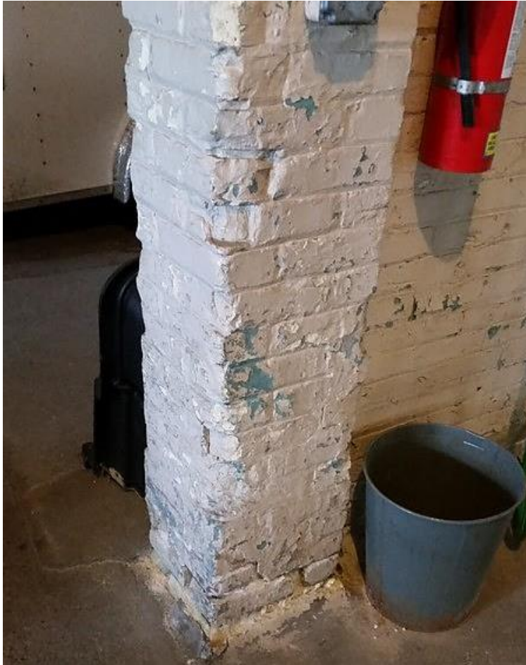
Figure 33: Interior brick deterioration.
