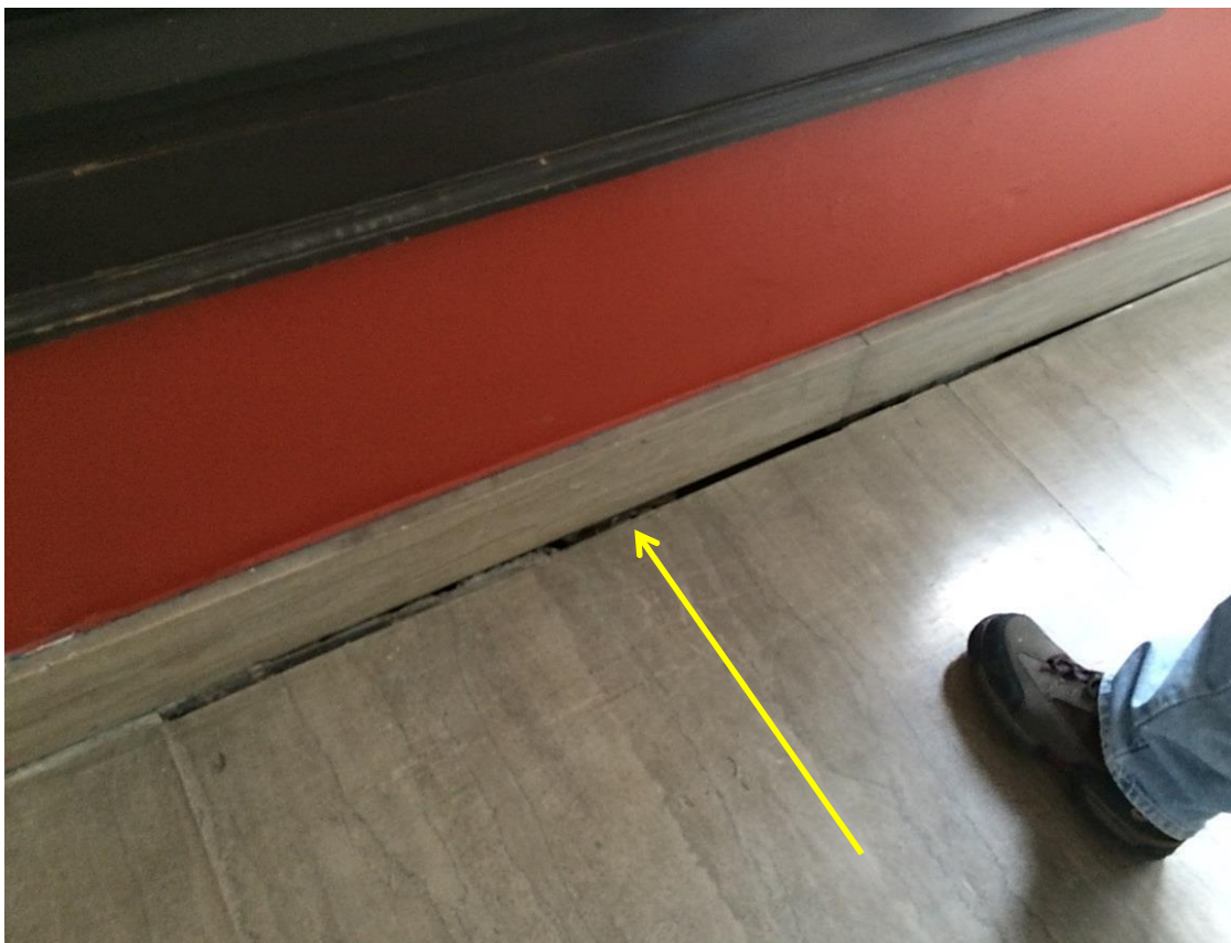
Figure 72: Floor separation from wall in stairwell at fourth floor, north
