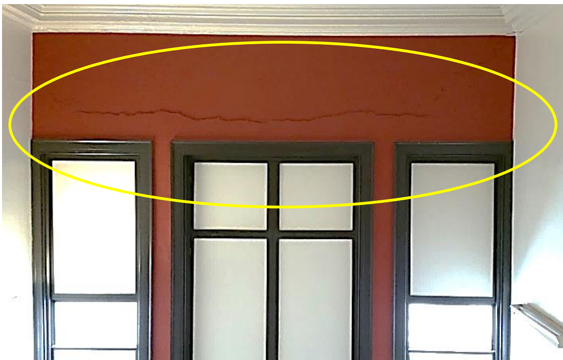
Figure 70: Significant wall cracking in stairwell at fourth floor on north facade
