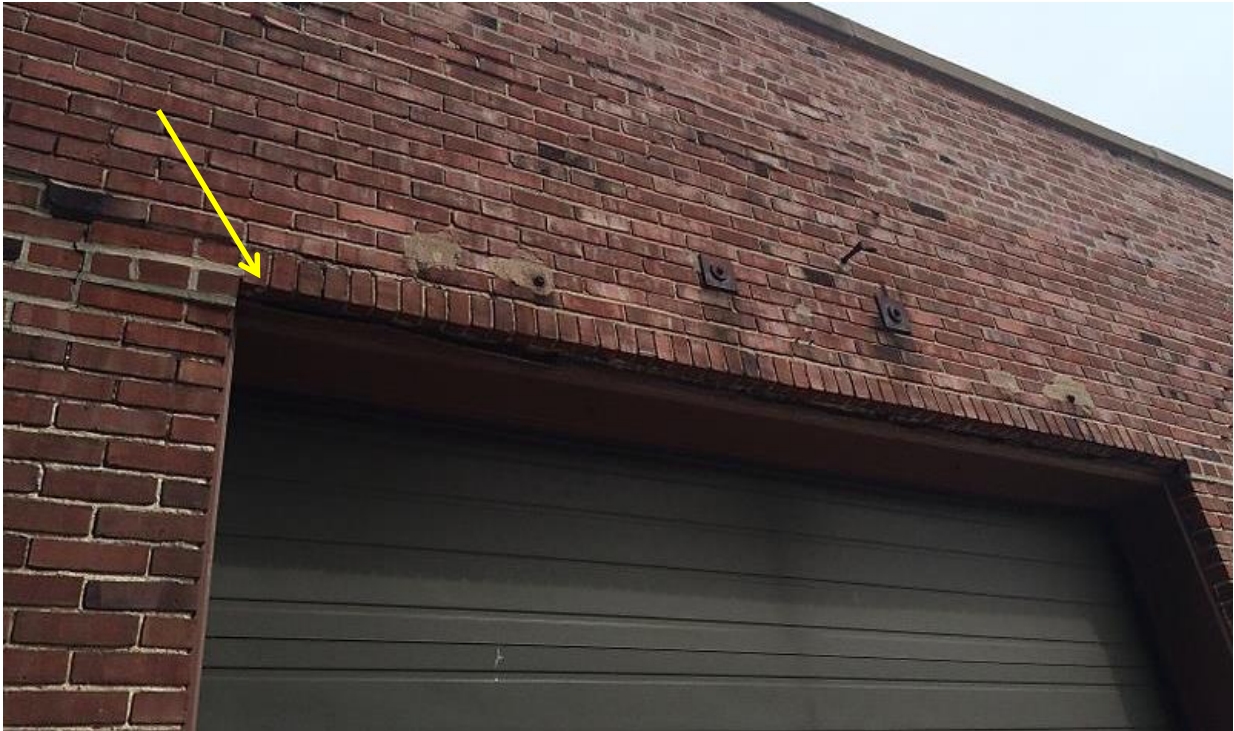
Figure 28: Corroded steel door lintel.
