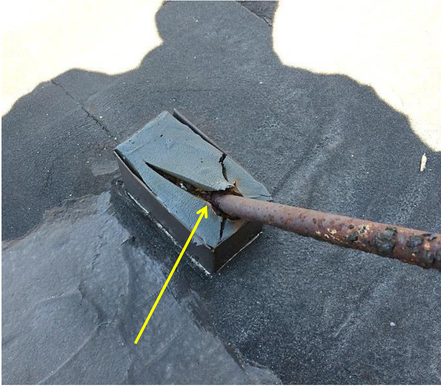
Figure 27: Deteriorated pitch pocket
