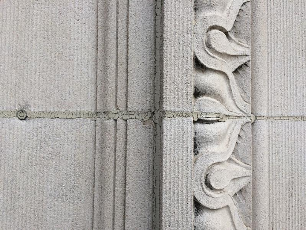
Figure 46: Deteriorated stone mortar joints with deteriorated sealant over mortar.
