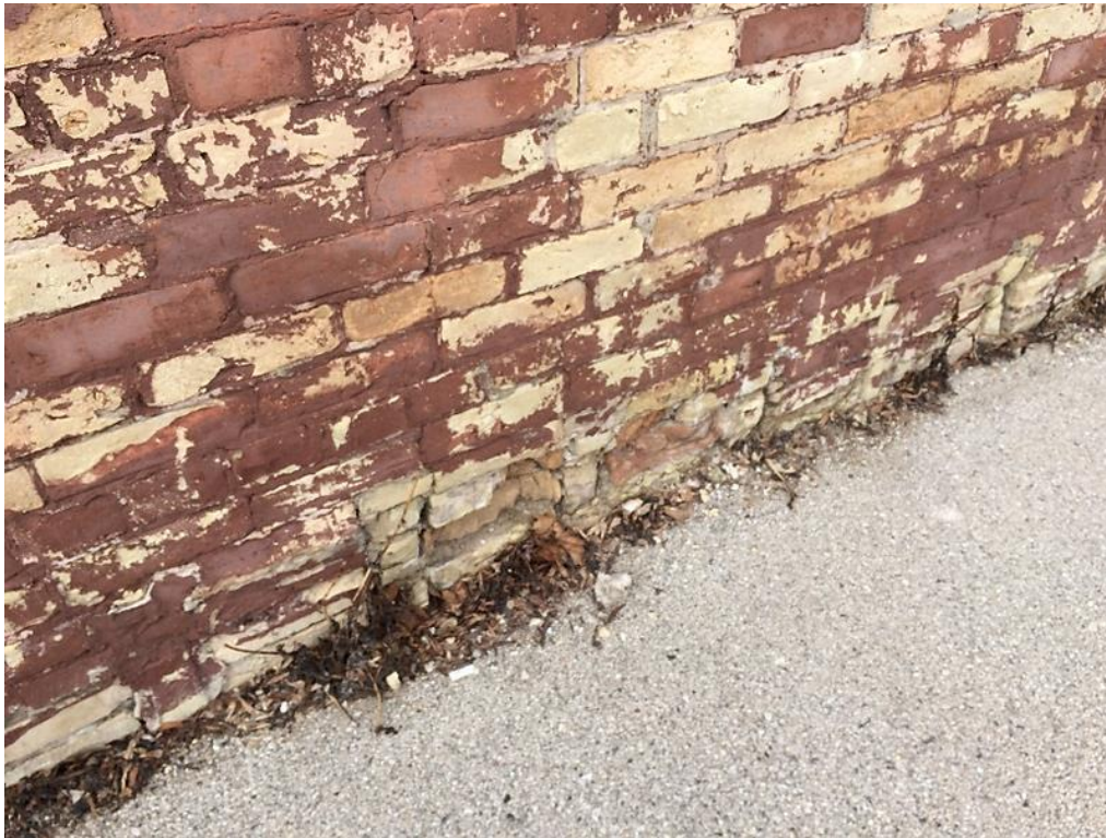
Figure 23: Deteriorated mortar joints.
