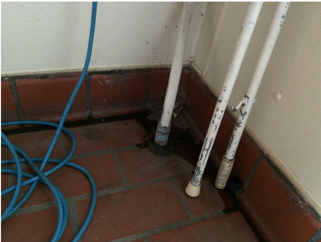
Figure 50: Unsealed penetrations allowing leaking into basement.
