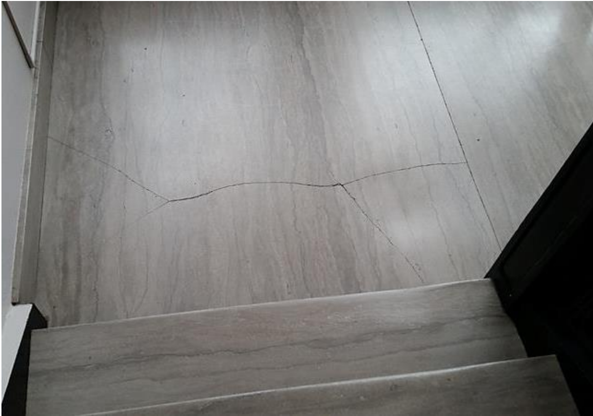
Figure 73: Cracked marble floor in stairwell at fourth floor
