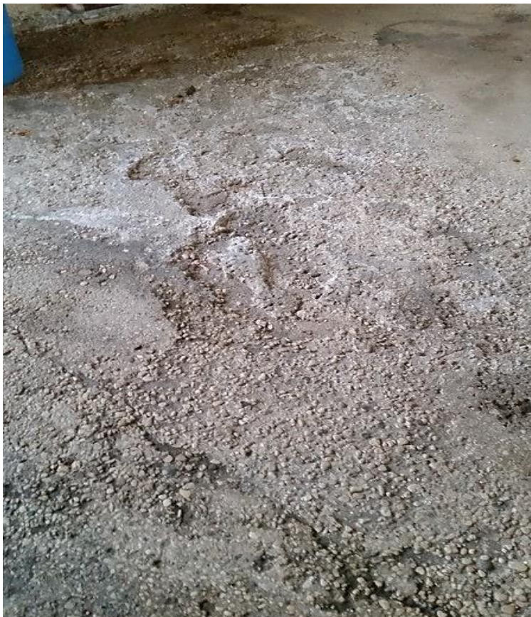
Figure 36: Deteriorating concrete floor.
