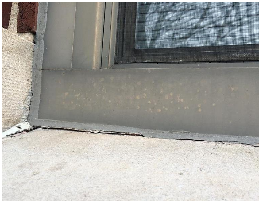
Figure 30: Deteriorated sealant at window perimeter
