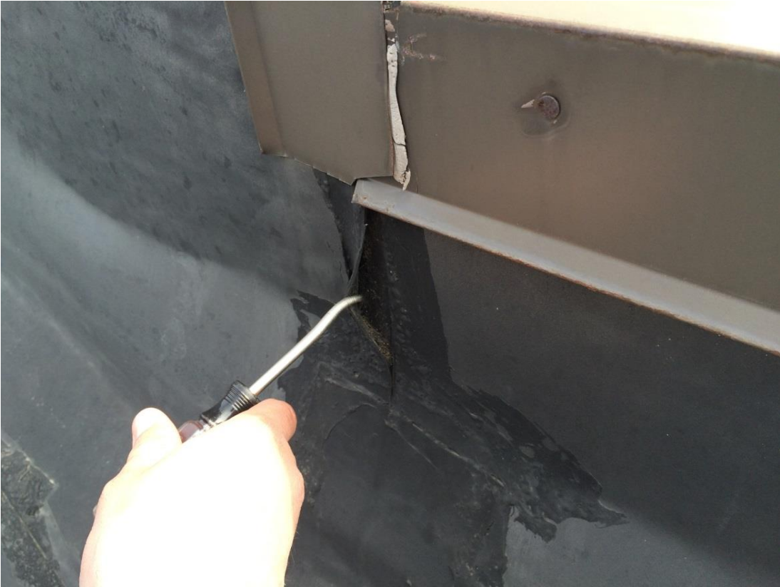
Figure 17: Open flashing seam.
