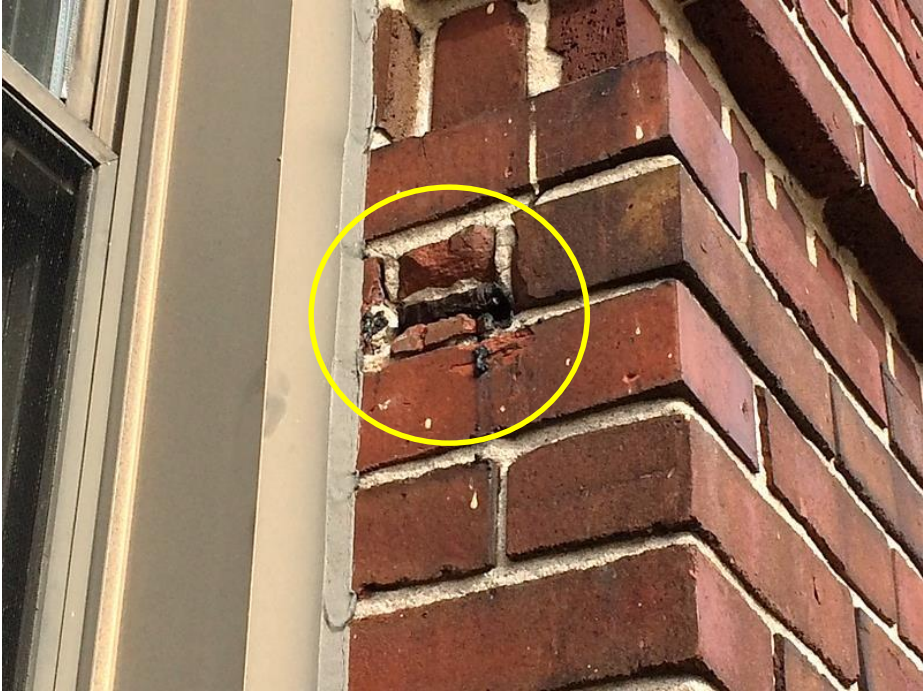
Figure 38: Corroding embedded steel at window jamb
