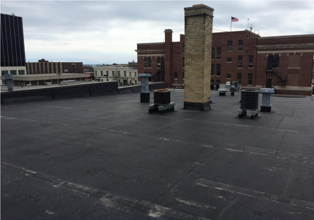
Figure 8: Full adhered EPDM roof system.
