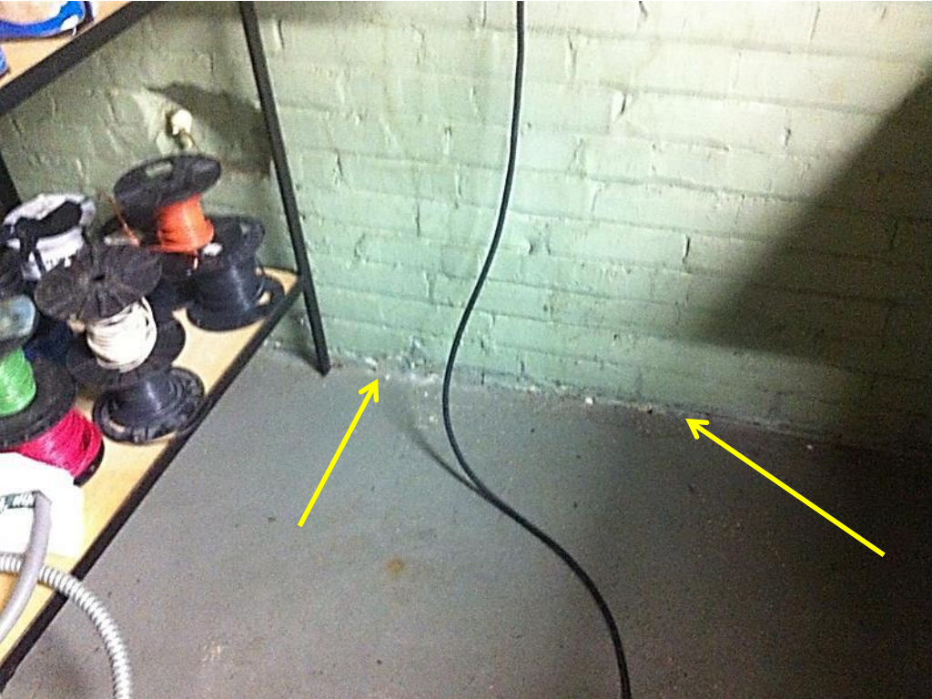
Figure 50: Leaks present along foundation wall
