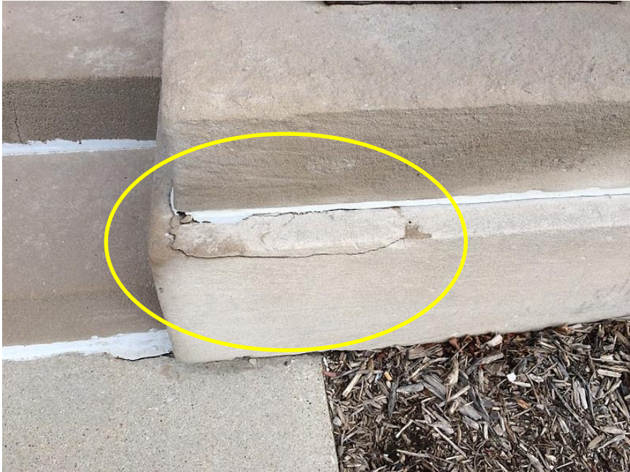
Figure 12: Spalled stone at main entrance, south facade
