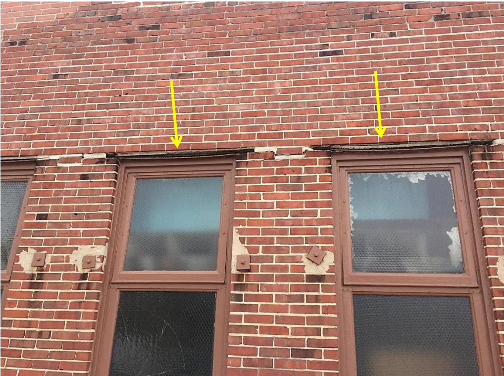
Figure 26: Corroded steel window lintels.
