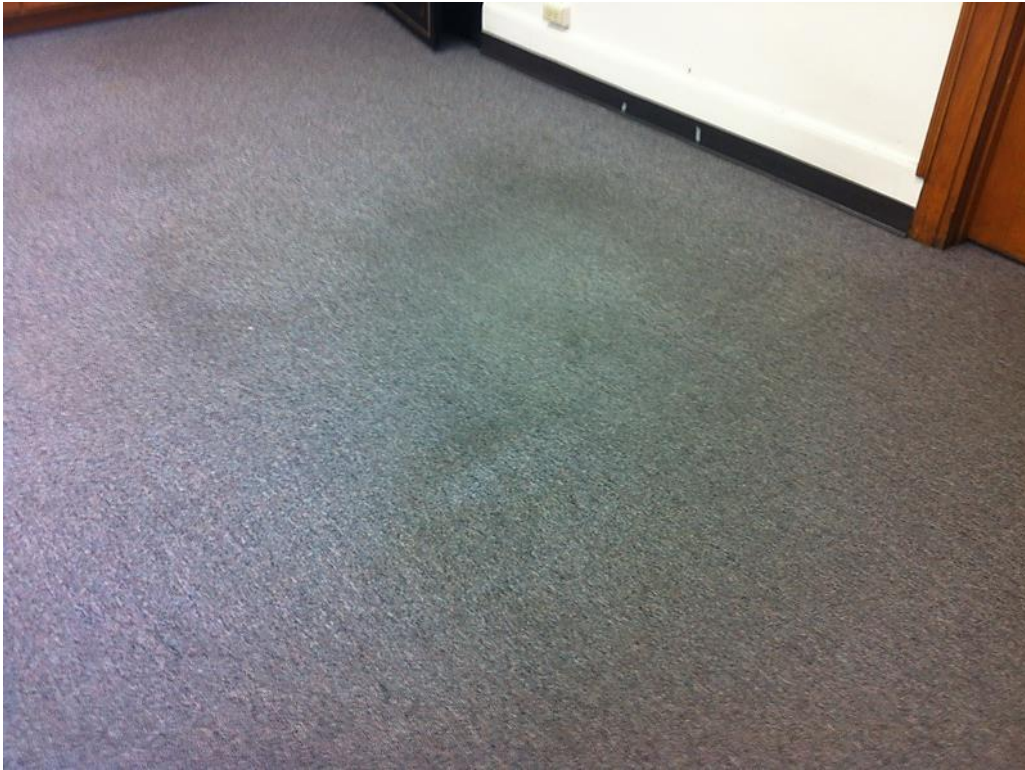
Figure 63: Office carpet in poor condition
