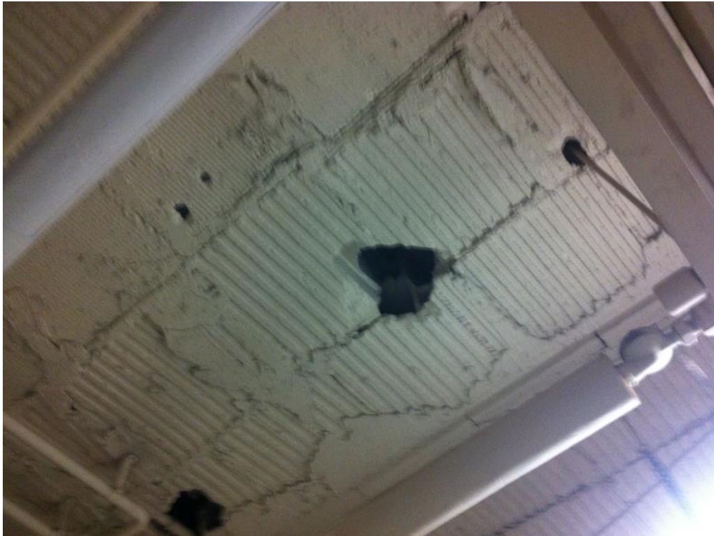
Figure 57: Hole in clay tile ceiling
