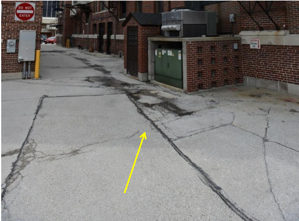
Figure 13: Deteriorating asphalt pavement at alley, north elevation
