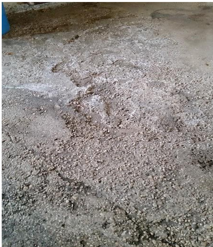
Figure 36: Deteriorating concrete floor.
