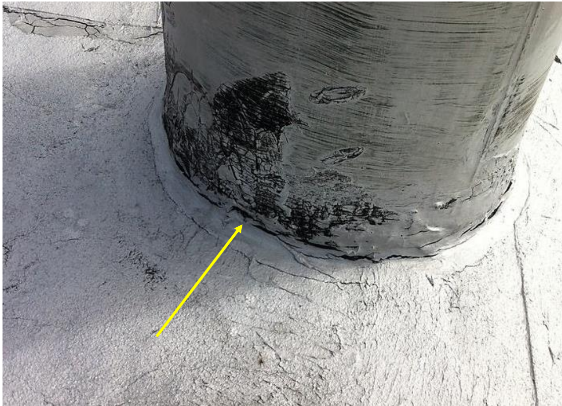
Figure 15: Failed joint at penetration.
