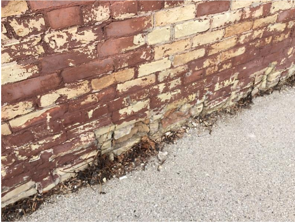
Figure 23: Deteriorated mortar joints.
