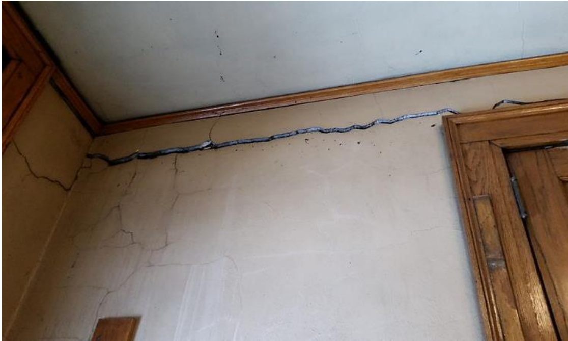
Figure 71: Significant wall cracking at fourth floor on east wall that returns to exterior north wall.
