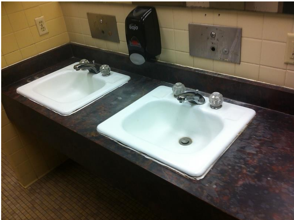
Figure 66: Aged bathroom fixtures
