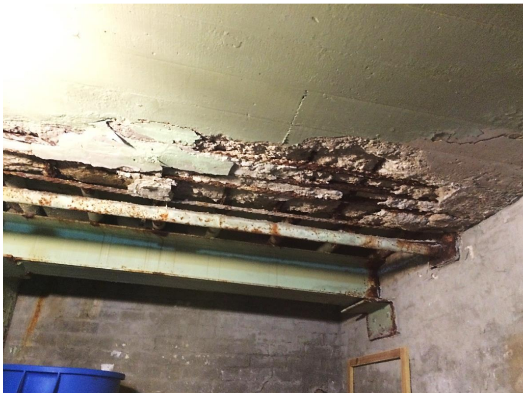
Figure 58: Exposed rebar/structure deterioration in vault below alley.
