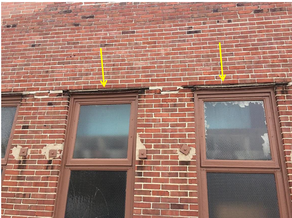
Figure 26: Corroded steel window lintels.
