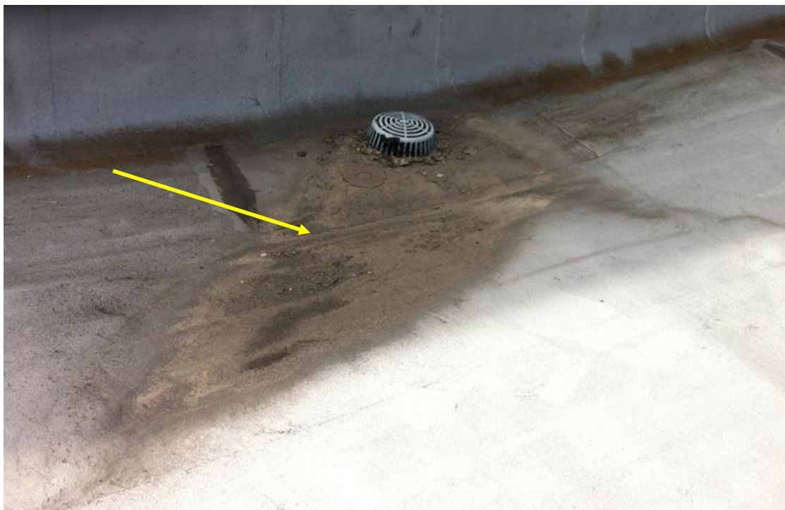
Figure 16: Ponding at roof drain.
