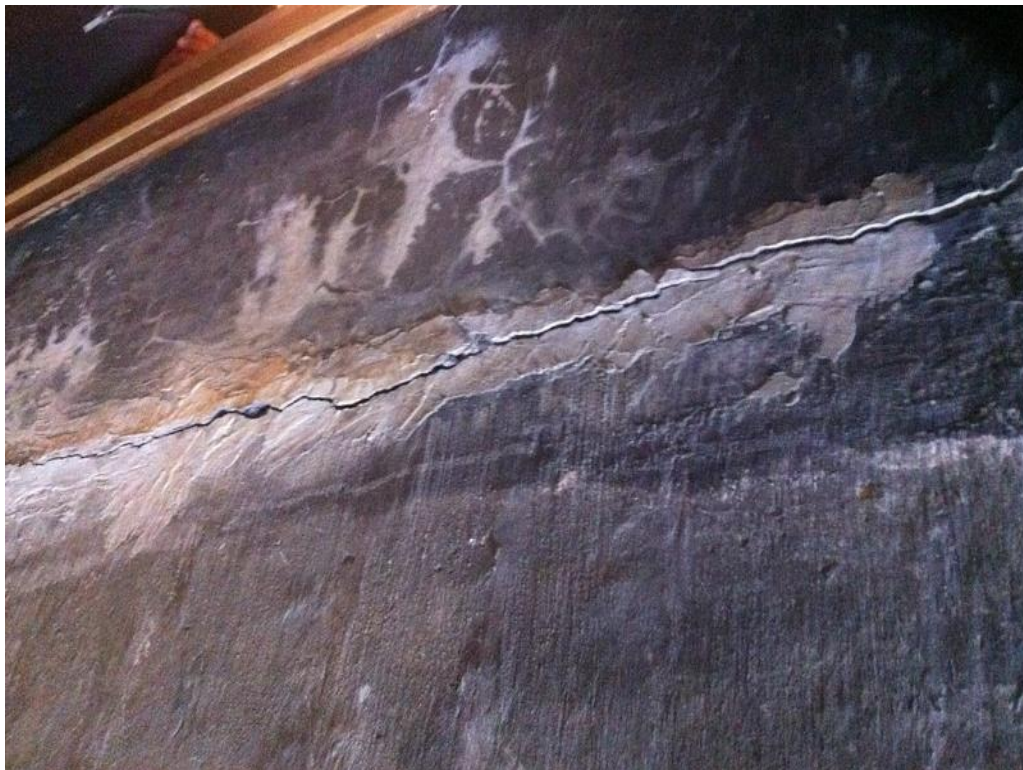
Figure 62: Foundation cracking in north basement exit stairwell
