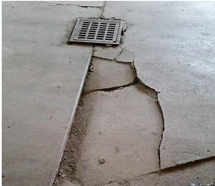
Figure 35: Concrete floor cracking.
