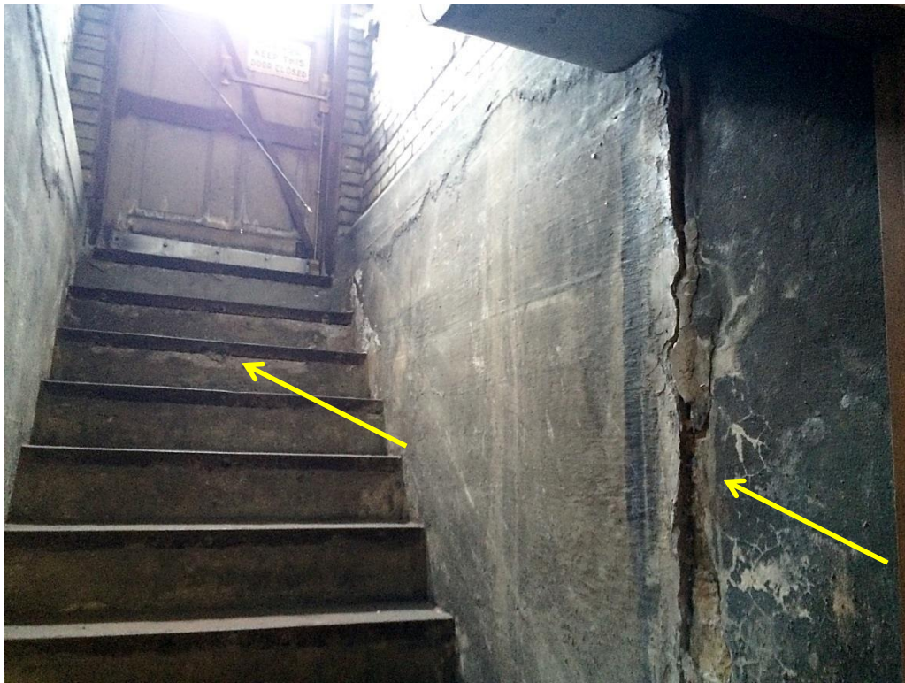
Figure 61: Opened wall joint and spalled steps in north basement exit stairwell
