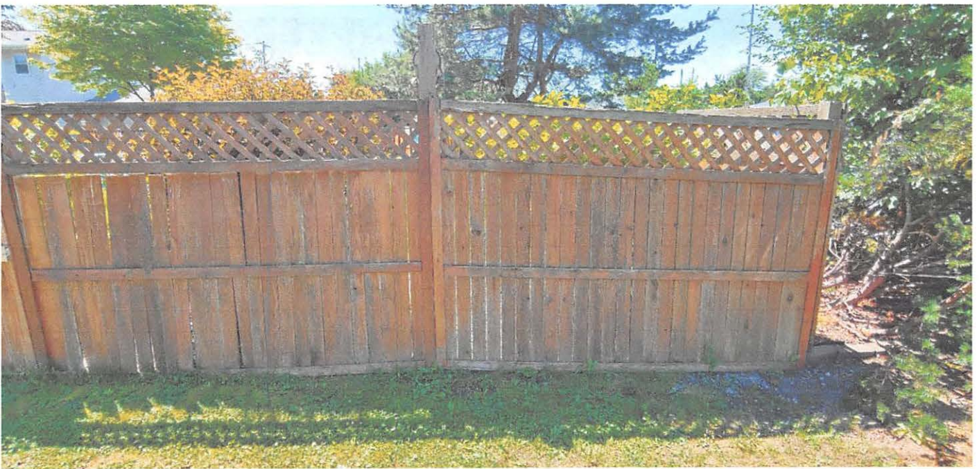
Figure 8: Greying with loose/damaged pickets.
