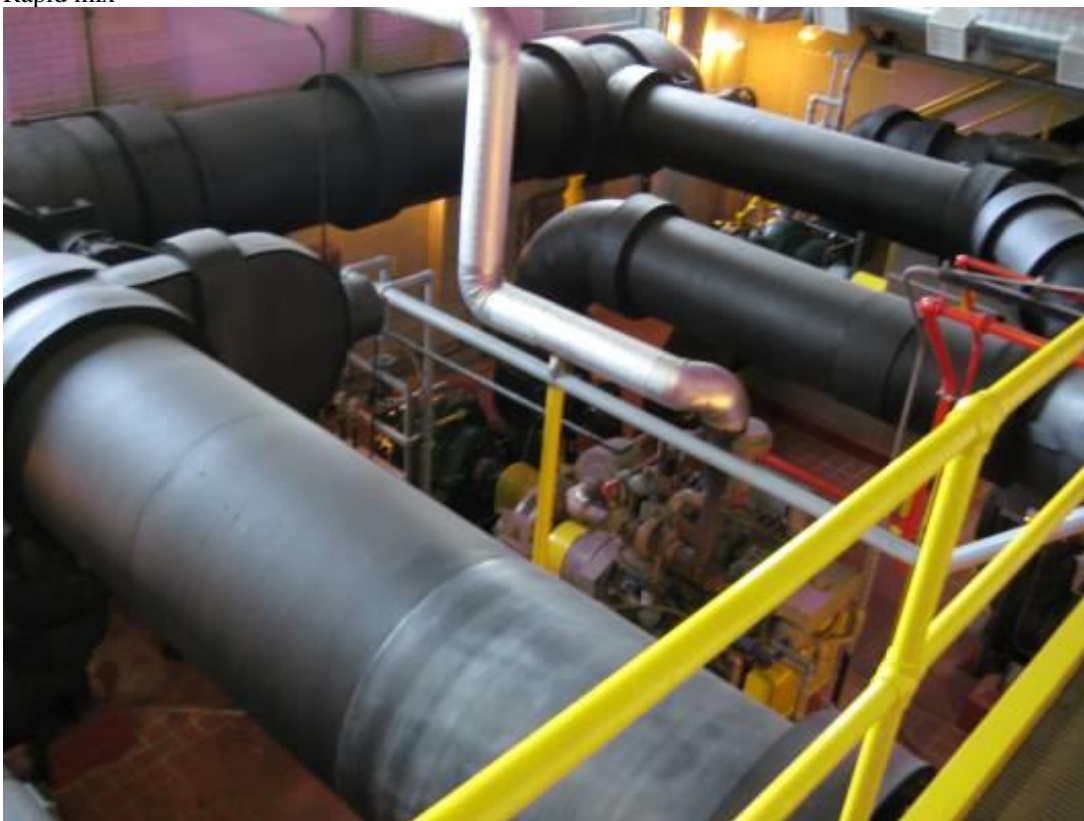
Low Lift Pumps
