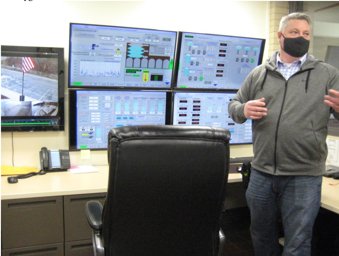
Sheboygan Control/Computer/Security Room
