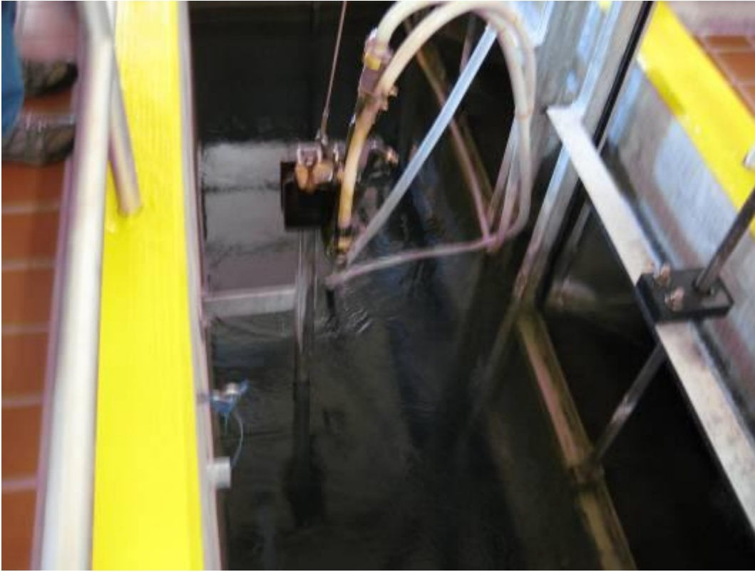
South Flocculation/Sedimentation basins
