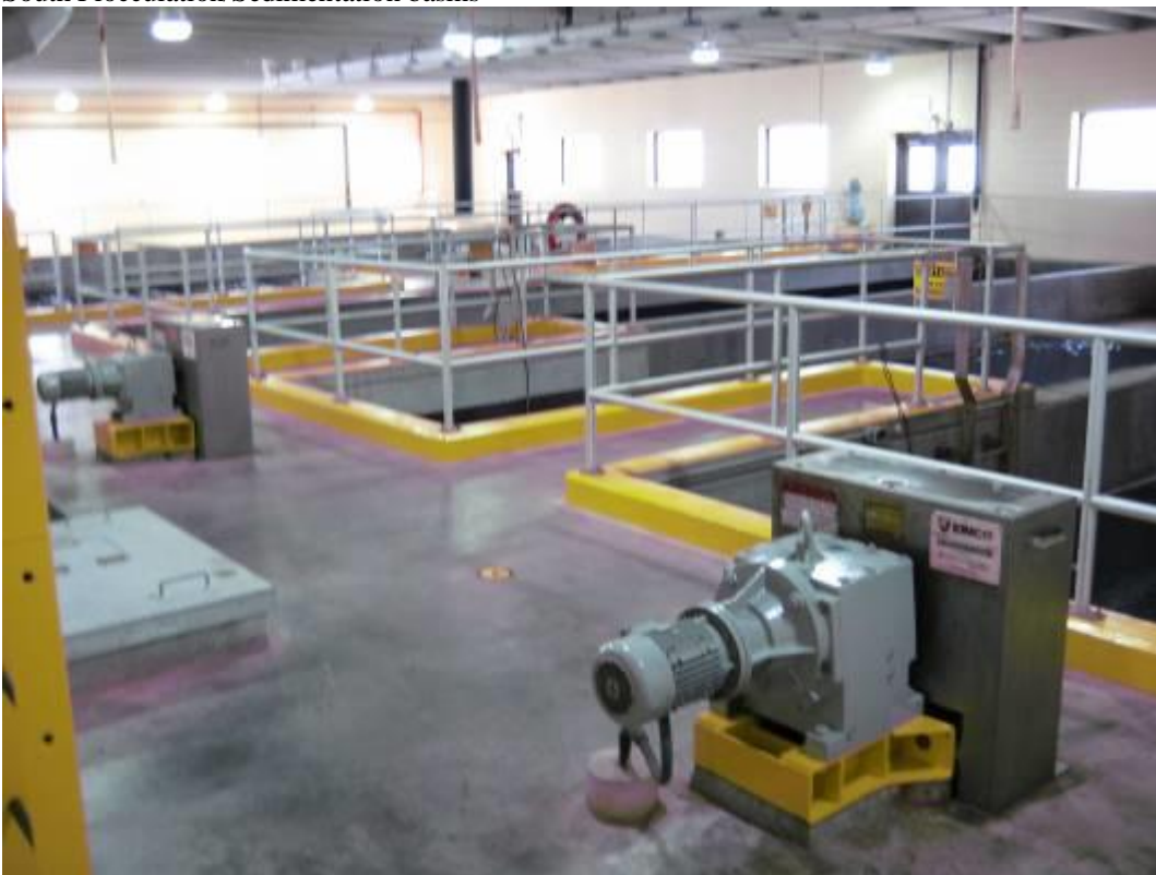
South Flocculation/Sedimentation basins
