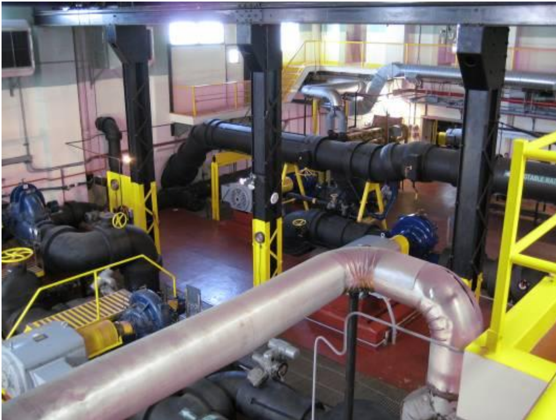
High Lift Pumps
