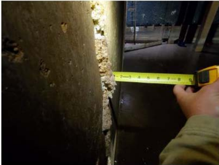
Photograph 3: Efflorescence up to 1.5" thick at interior wall, upper east cell, looking north.
