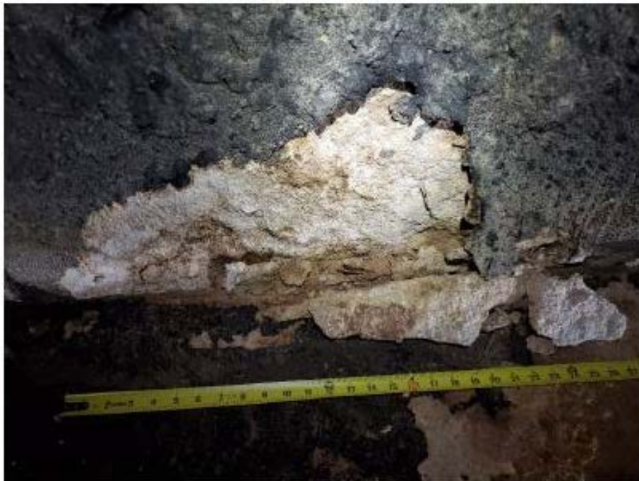
Photograph 4: Delamination and spalls along bottom of upper east cell, typical along north half.
