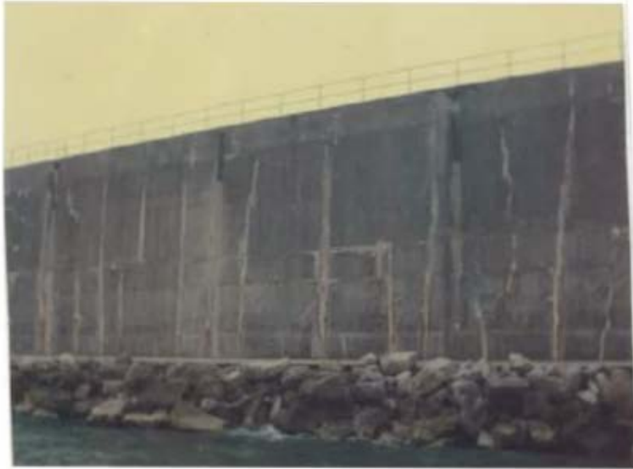
Photograph 33: 1993 Pre-repair photo, scupper 2, 3 and 4 shown.
