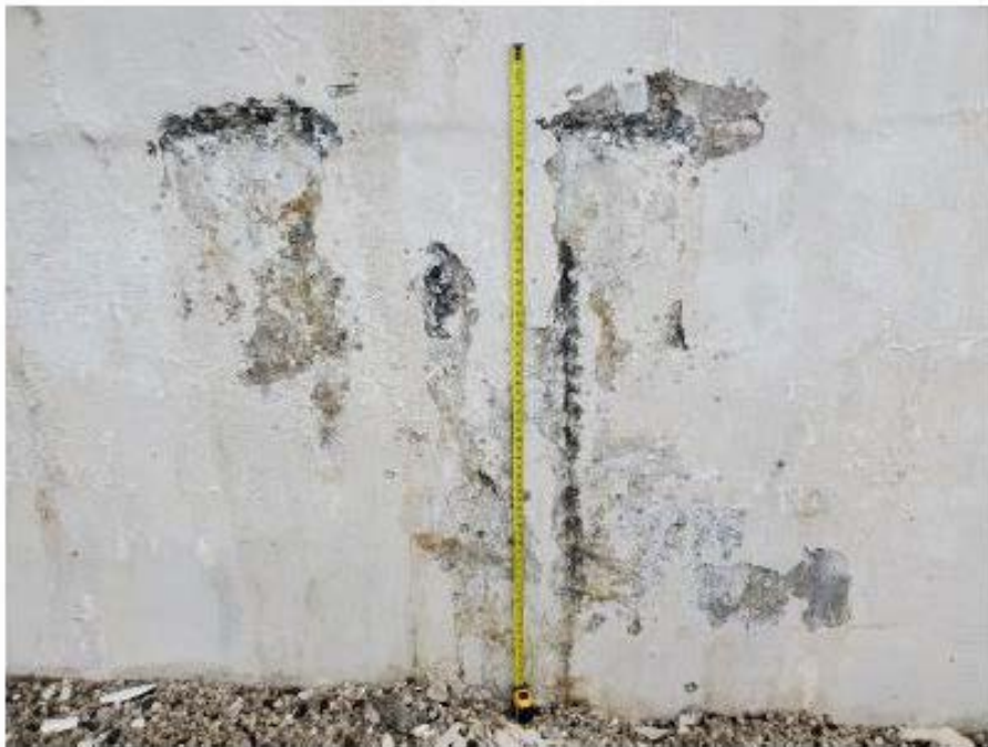
Photograph 12: Condition of exterior concrete wall beneath skim coat on south wall.
