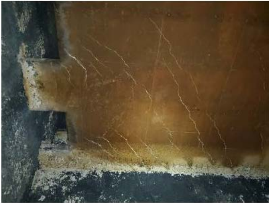
Photograph 1: Diagonal cracking typical at corners in underside of slab ceiling slabs.
