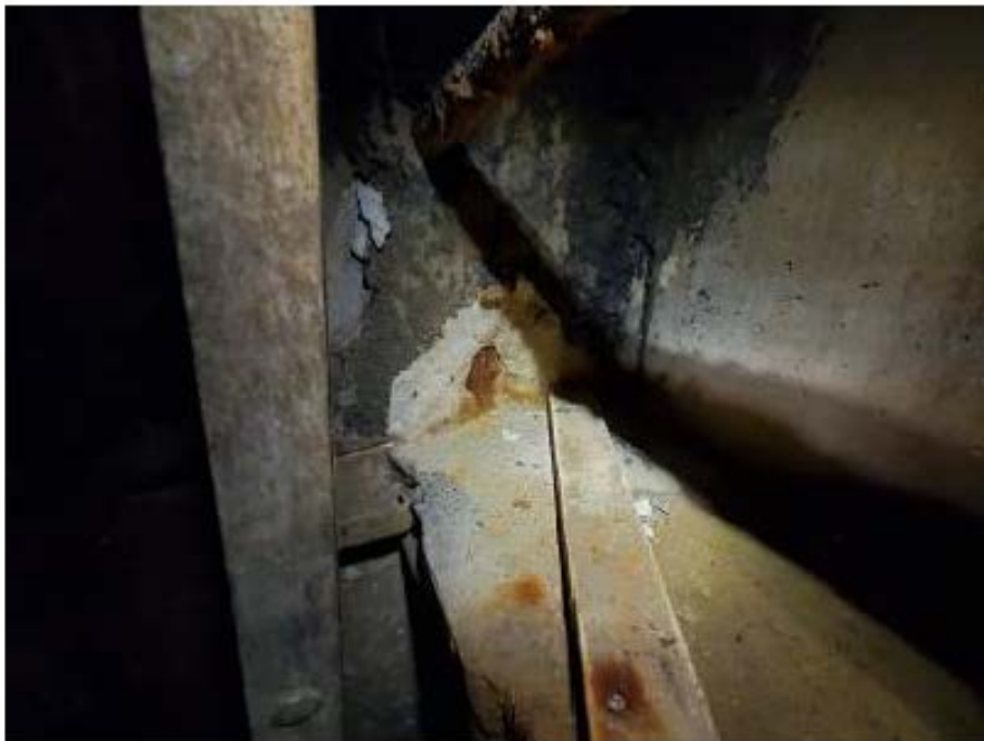
Photograph 2: 2' wide x 1' high spall in south wall of upper east mixing basin at floor.
