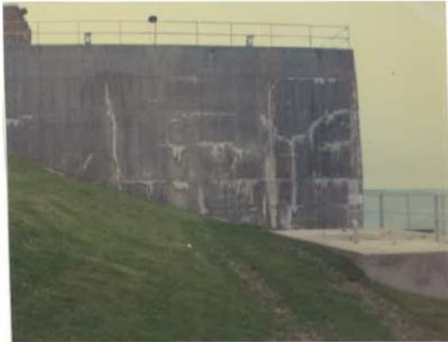
Photograph 39: 1993 Pre-repair photo, south wall shown. .
