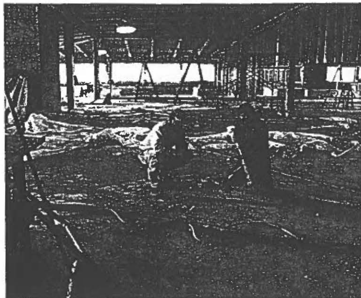
Workers prepared for fireproofing on the third floor of the library building. Interior work will continue through spring.
