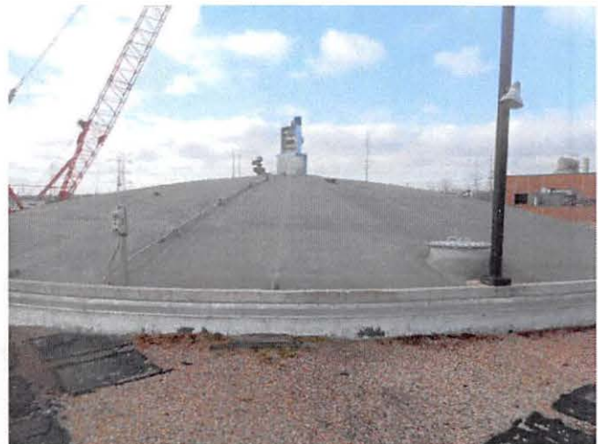
New Water Treatment Roof – 3 of 4 large digesters covered with spray foam insulation. 4 th digester is bare metal. Recommend coating all 4 to prevent deterioration seen on Revised digesters.
