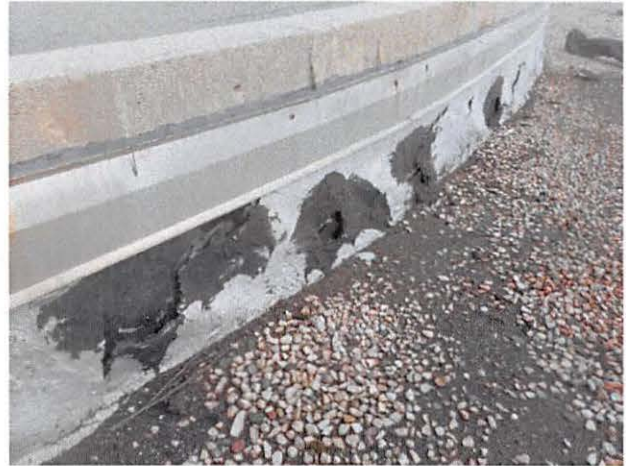
New Water Treatment Roof – Large holes in flashing around entire roof perimeter. Roof in failure mode and scheduled for replacement in 2018.
