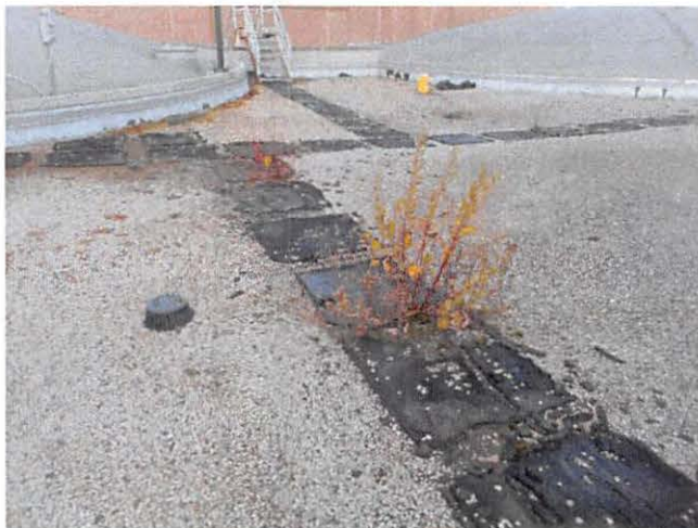
New Water Treatment Roof – Heavy vegetative growth occurring throughout roof system.
