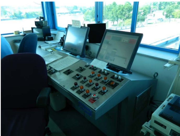
8 th Street Bridge Controls
