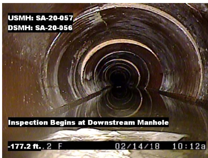
Debris in a Sanitary Sewer
