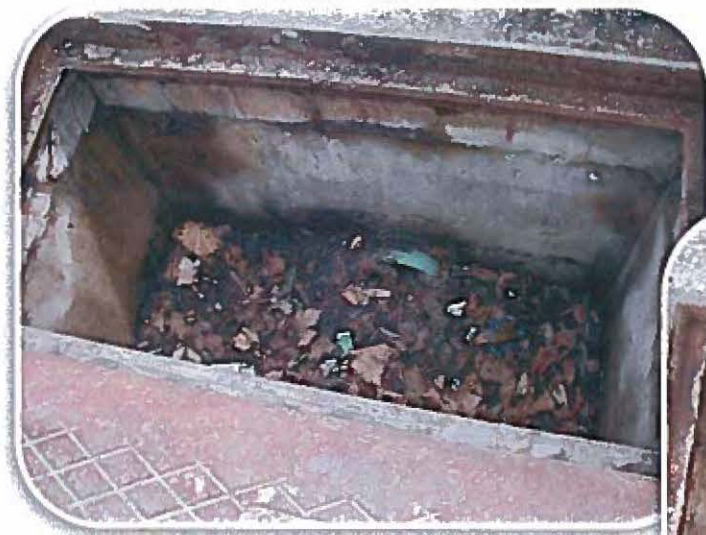
Catch Basin before Cleaning
