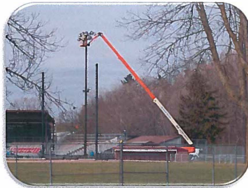
Ball Diamond Lighting Maintenance
