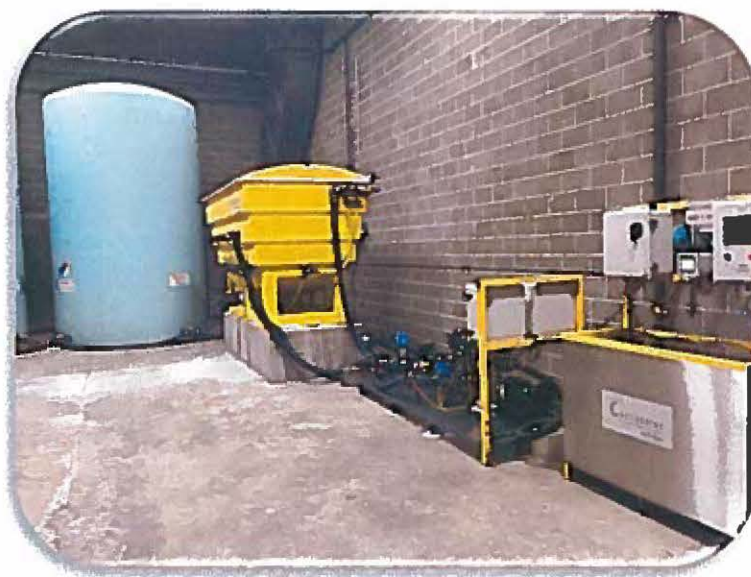
Salt Brine Production Equipment
