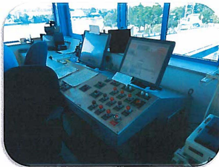
8 th Street Bridge Controls
