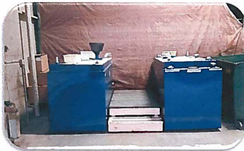
DPW Oil Collection Tanks
