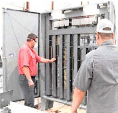
Control Panel FAT
