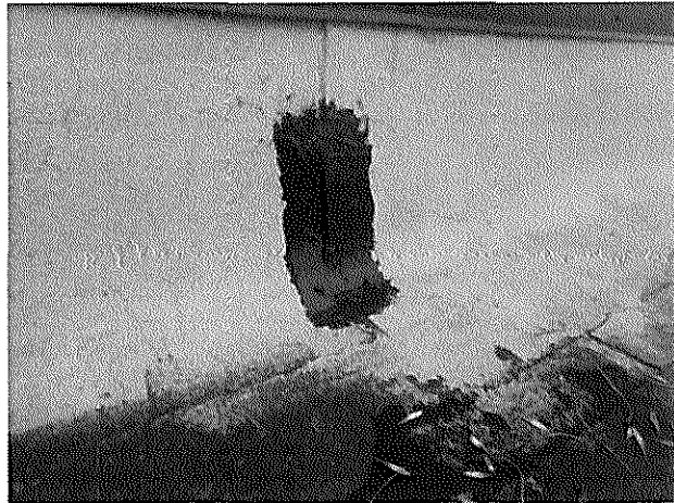
Transit Garage – Roof #2 – Open lap was repaired with 3-course of asphalt roofing mastic and fiberglass reinforcing fabric.
