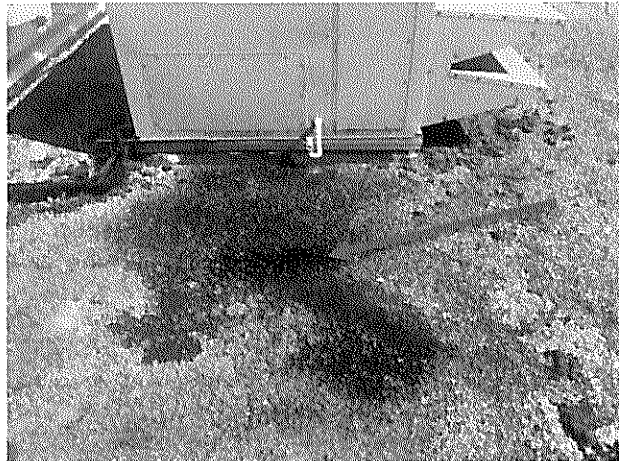
Transit Garage - Roof #1 – Lack of pipe extension lead to ponding water around A/C unit. This results in aggregate washout and vegetative/mold growth.
