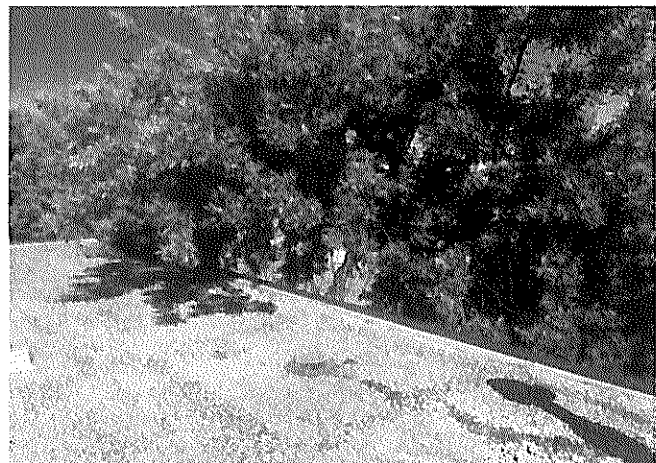
Transit Garage - Roof #4 – Large tree branches hanging over roof. This results in debris clogging the drain, and the risk of broken branches penetrating the roof system.
