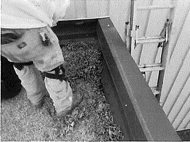
Transit Garage – Roof #1 – Significant organic debris can lead to clogged drains and ponding water on roofs.
